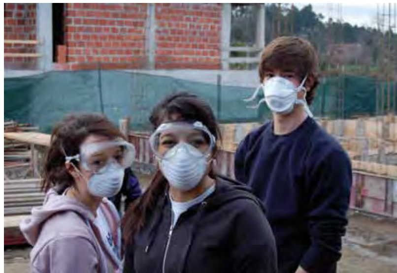
Habitat for Humanity student volunteers Mara Goodman, Zahra Masters, and Viktor Behrens mix concrete. Photo by Jacob Mulligan '10
