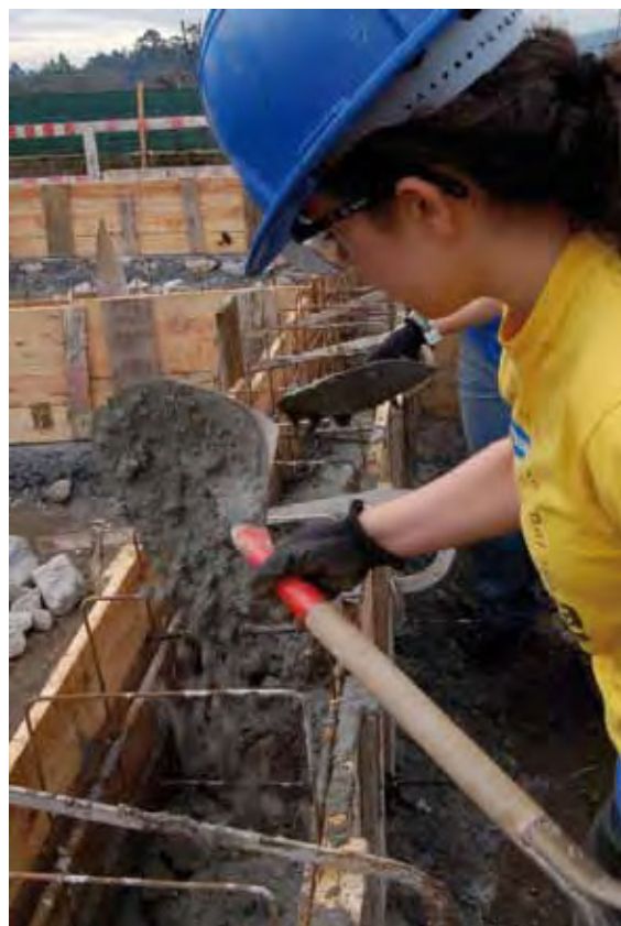
Elyse Guizzetti adds concrete to a foundation wall. Photo by Jacob Mulligan '10
