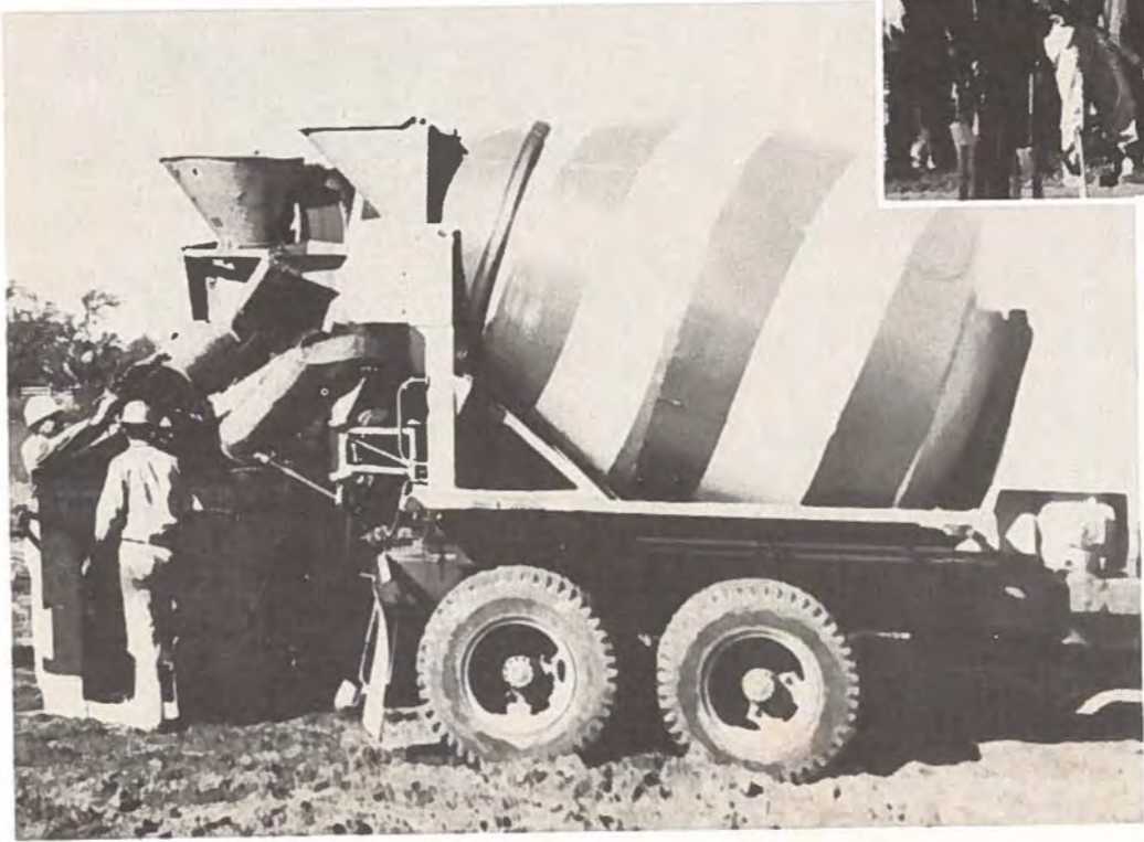
One of the many loads of redi-mix used in pouring the floor of the gym is being unloaded.
