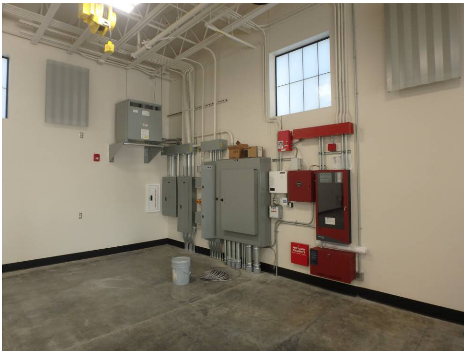
Electrical panels/ fire alarm panels (8/14)
