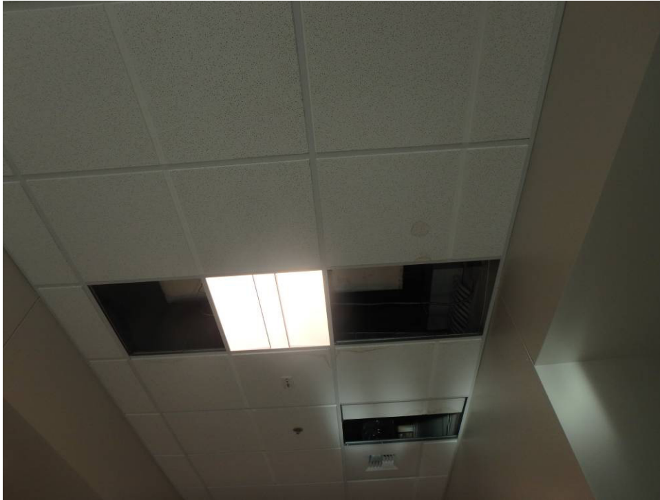
Ceiling panels to be replaced
