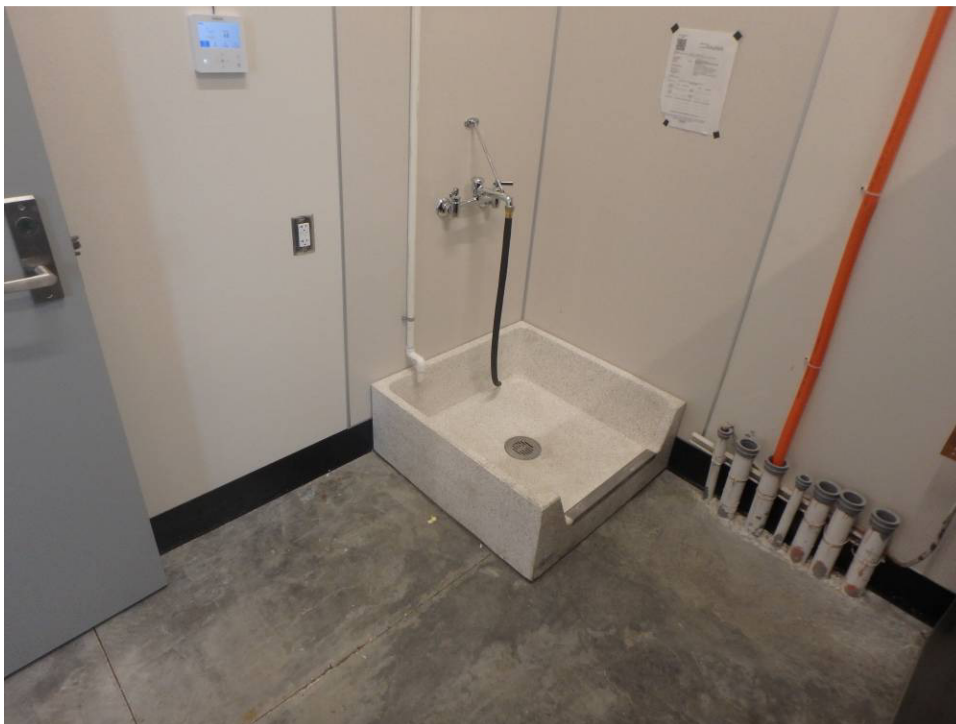
Mechanical Room janitor's sink
