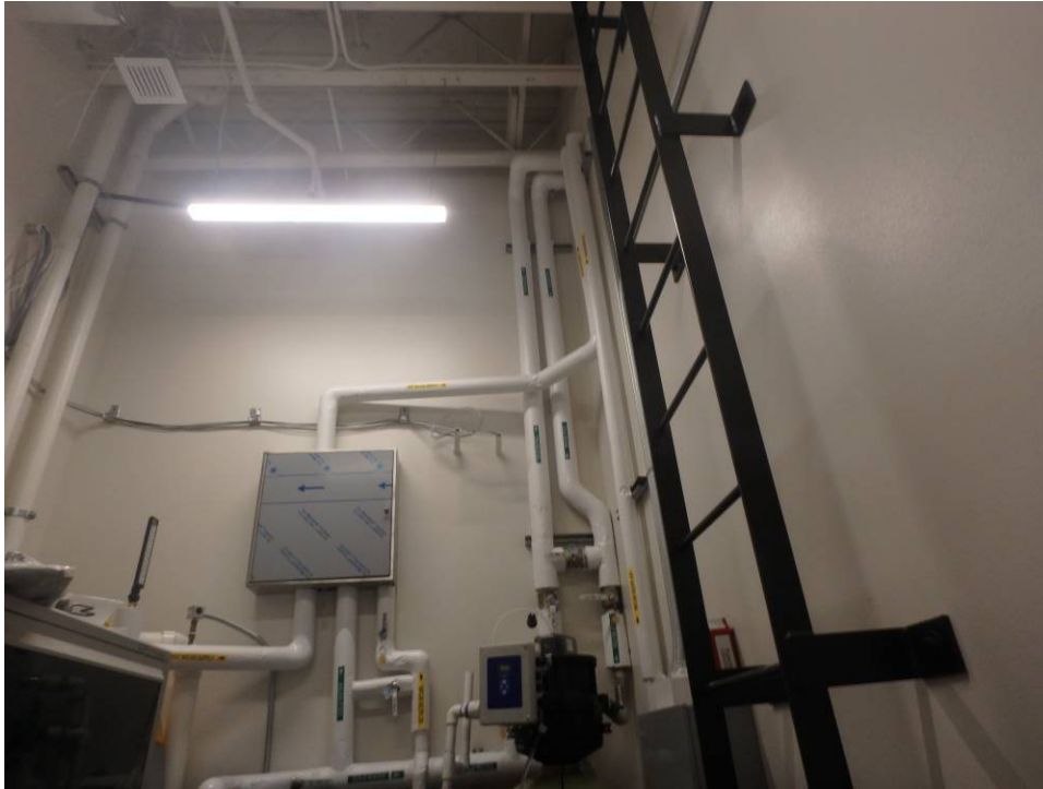
Mechanical Room piping
