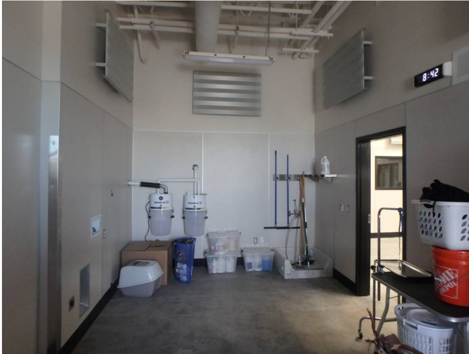
Vacuum in kennel room
