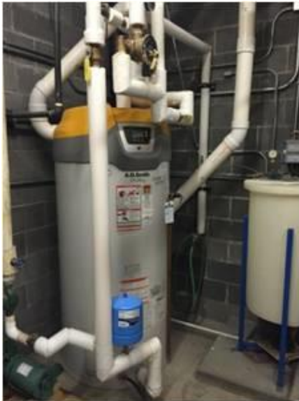
Existing water heater
