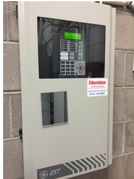
Existing controls panel
