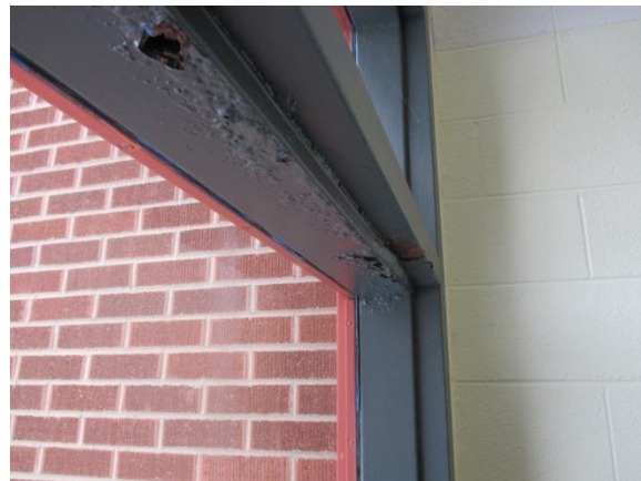
Windows in the 1982 addition are showing signs of rust and deterioration. They are due for replacement
