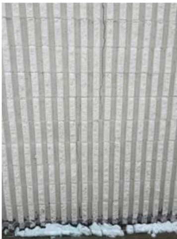
Visible cracking of exterior walls
