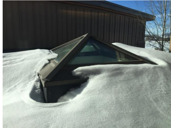
Multiple skylights have leaked since construction.
