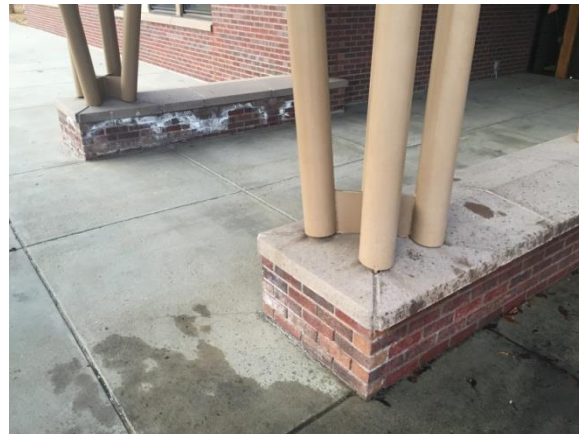
Efflorescence occurring at exterior walls.
