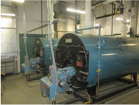
Boilers are original to construction.
