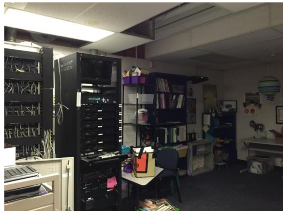
Technology equipment in office/teaching space
