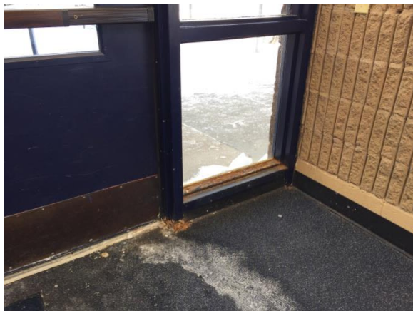
Damage to door frame and floor finishes due to moisture infiltration
