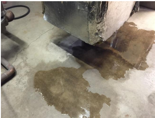
Equipment leak in Mechanical Room
