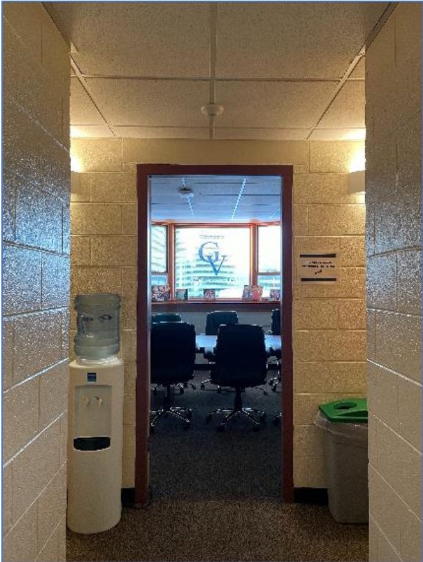
Photo #36: Great Valley School District Office, 1956 addition conference room. 2021. Camera facing northwest.
