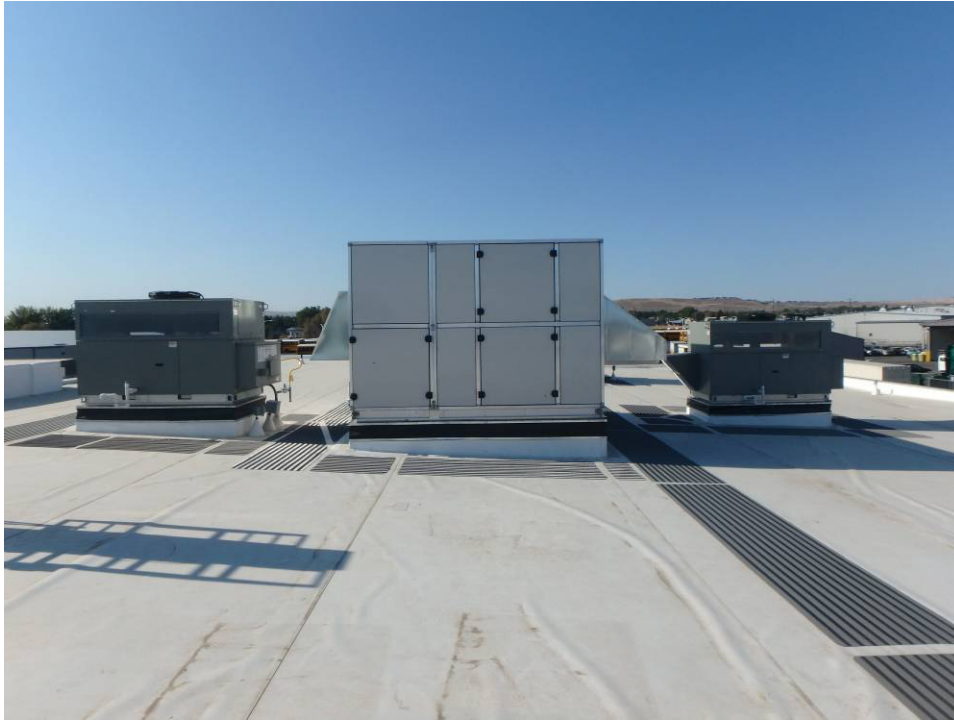
Looking south at the DOAS and two of the RTUs
