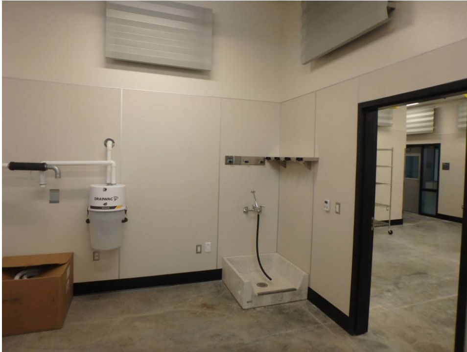
Kennel Room acoustical wall panels, vacuum and janitor sink on the north wall
