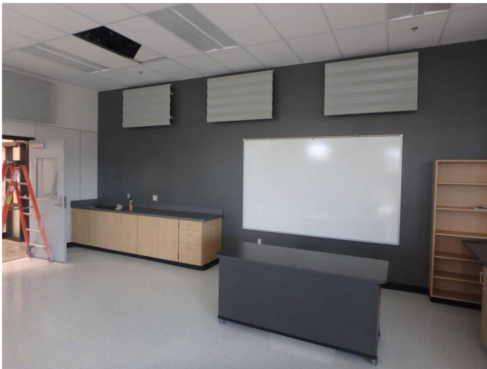
Looking at the acoustical wall panels on the west wall of the south classroom
