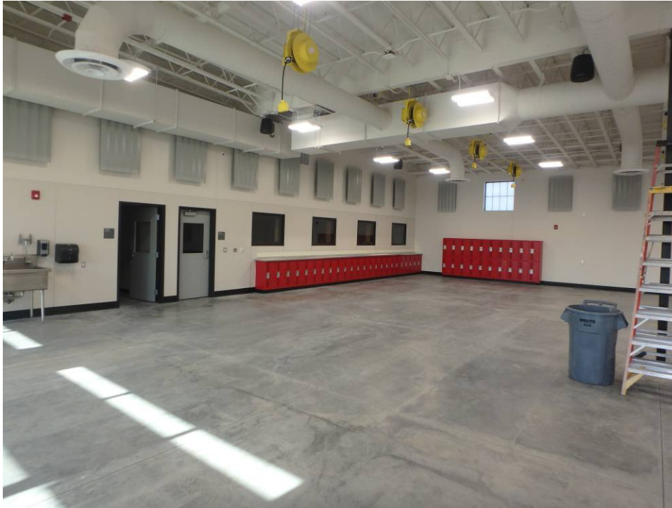
Wiring cord reels in the shop- south half
