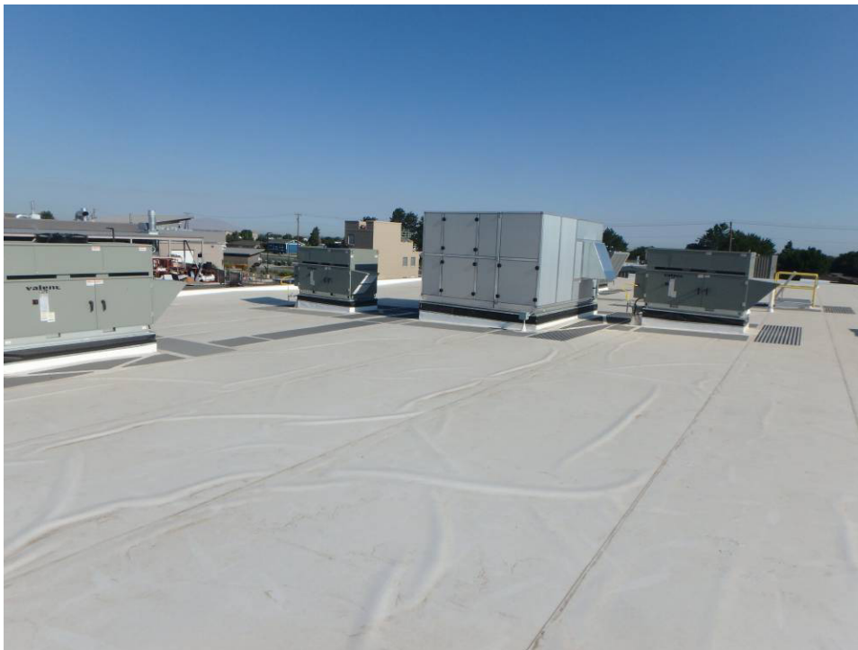
Looking north at the DOAS and three of the RTUs
