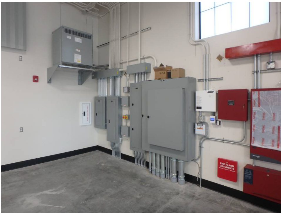
Looking northwest at the electrical panels and transformer mounted on the wall
