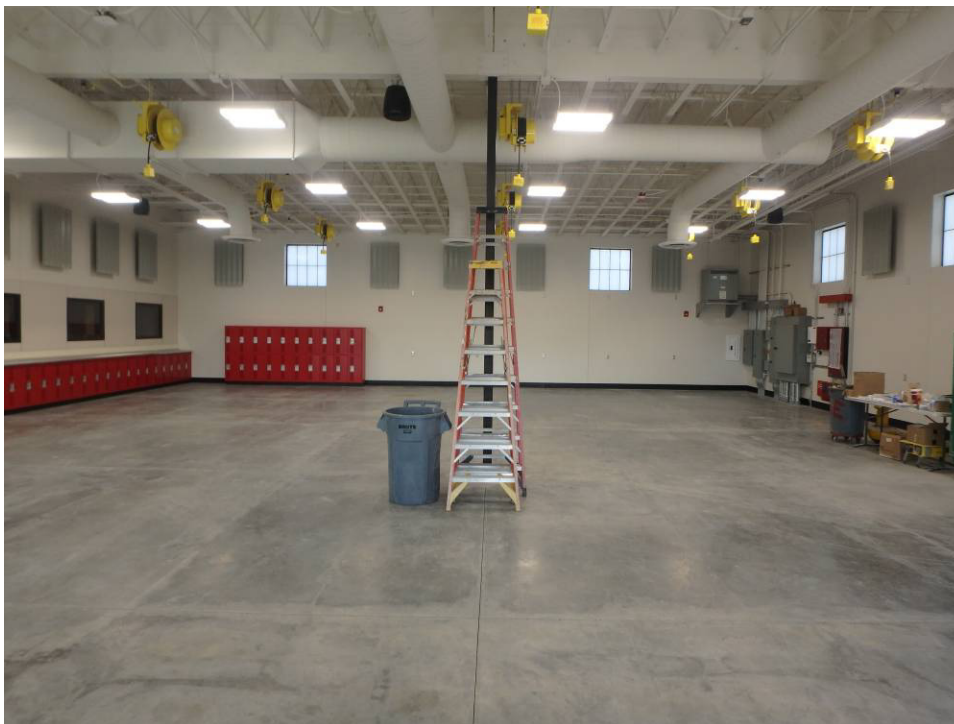
Wiring cord reels in the shop- north half
