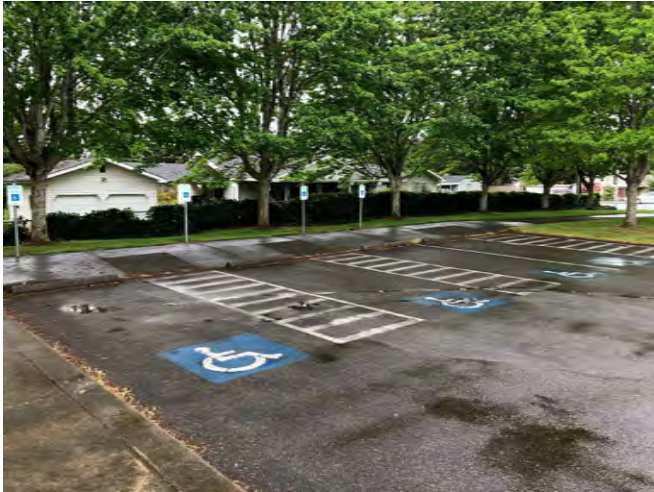
ADA stalls in parking lot. Instead of a curb cut, the sidewalk slopes down to the existing pavement. This does not meet all ADA standards
