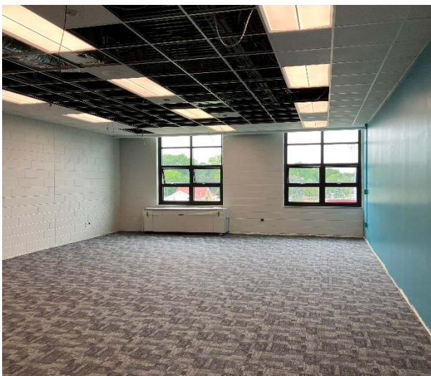
Left: Room 303 with new windows, fresh paint, and new carpet. Once the electrical and mechanical in the ceiling passes inspection, the rest of the ceiling tiles will be installed.
