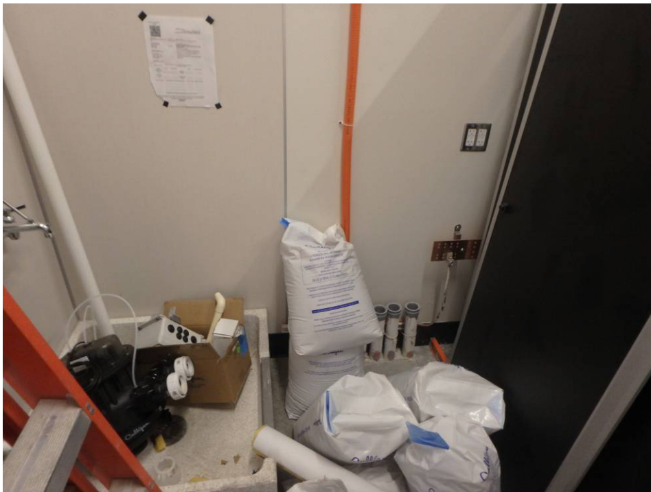
Mechanical room – Janitor's sink
