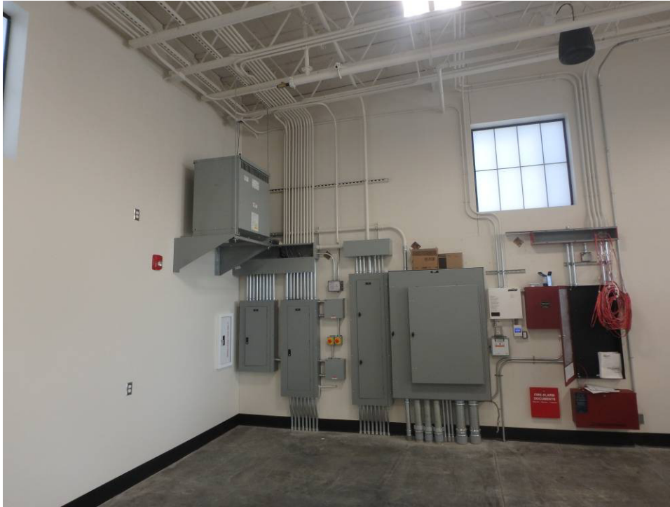
Looking northwest towards the shop's electrical panels and transformer mounted on the wall
