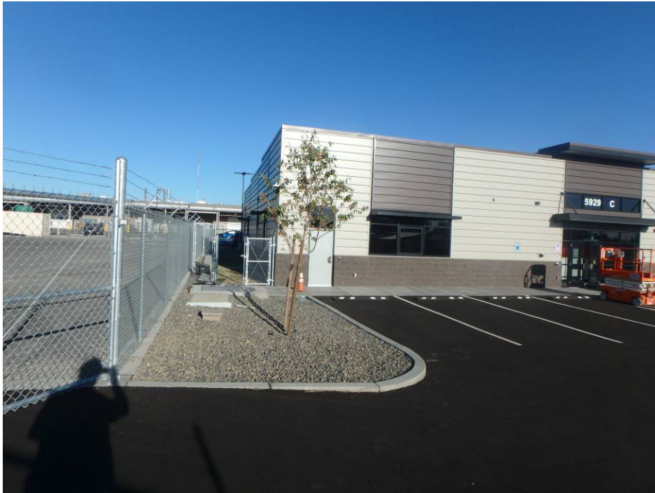
Looking west at the south side of the building and south property line
