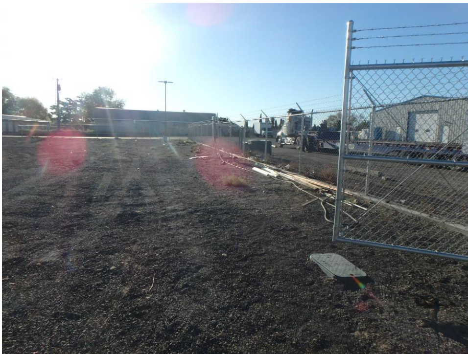
Looking east at the remaining plumbing items along the south property line
