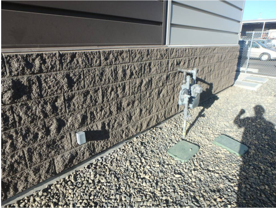
Sender wire mounted at gas meter
