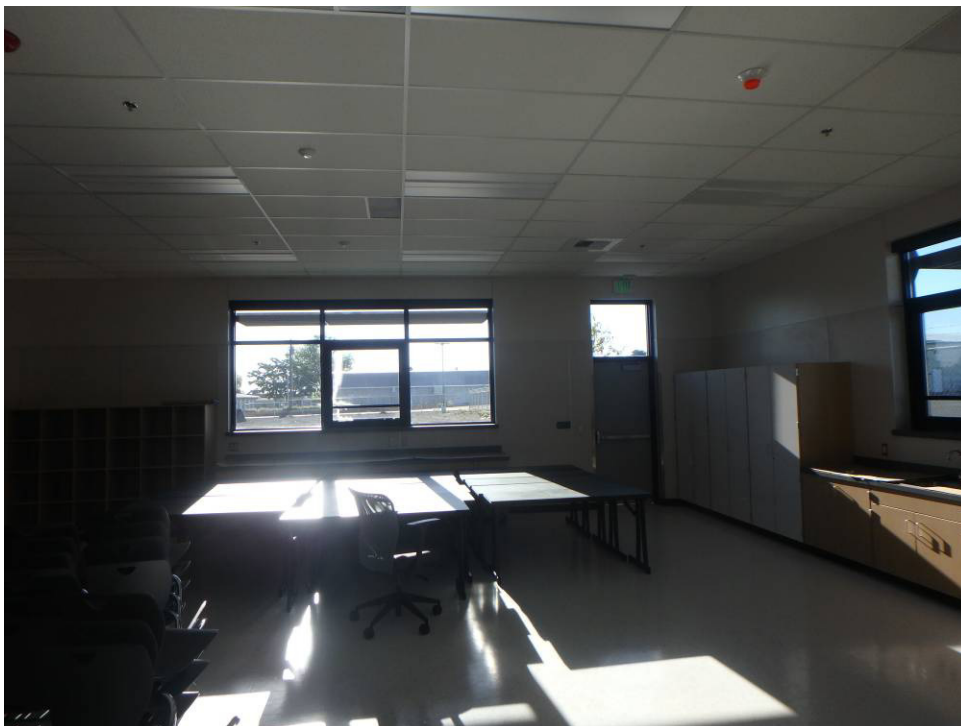
Looking east at the casework on the east and south walls of the south classroom
