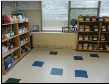
M9 Typical Unit Ventilator (1961 Addition) Replace unit ventilators with central energy recovery unit systems and VRF air conditioning.
