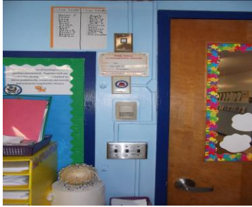
M12 HVAC Controls (1961 Addition) Upgrade existing pneumatic controls to DDC and connect to existing BMS.
