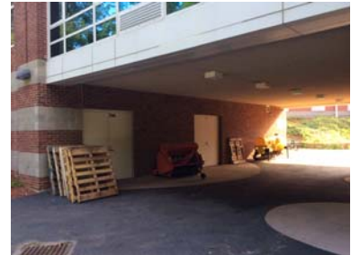
SS 16 Maintenance Equipment Storage Building Power maintenance equipment is stored outside and under the Kindergarten wing, which is a health and safety hazard. A Storage building is needed to house all of the District's equipment in one location.
