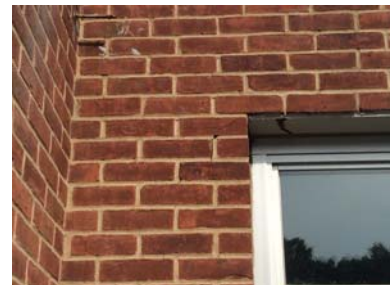
EB 2 Replace Rusted Lintels Lintels at the Gymnasium louvers, custodial office and room 5 are starting to expand due to rusting. Lintels should be replaced before they expand further and crack the brick veneer.
