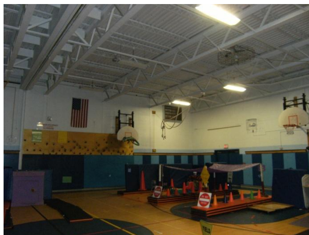
Figure 11: Gymnasium Corner Air Relief Fan
