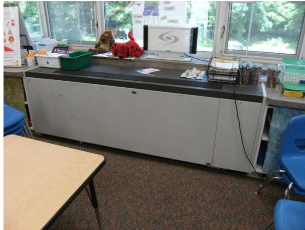
Figure 19: 2003 Wing Unit Ventilator
