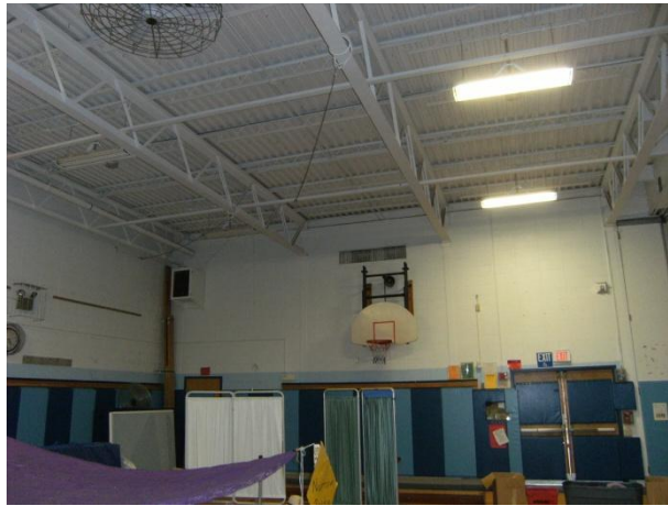
Figure 12: Gymnasium Supply Air Outlet and Corner Return Grille
