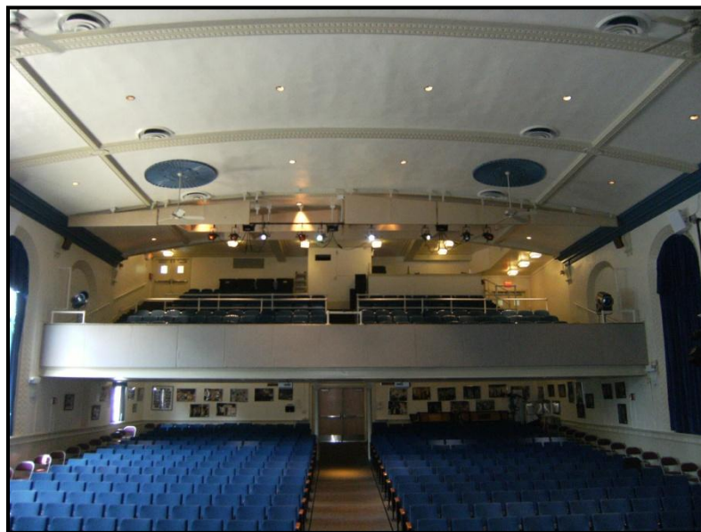
Figure 37: Auditorium Ceiling Diffusers
