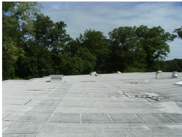
Figure 20: Typical 2003 Wing Roof Relief Hoods
