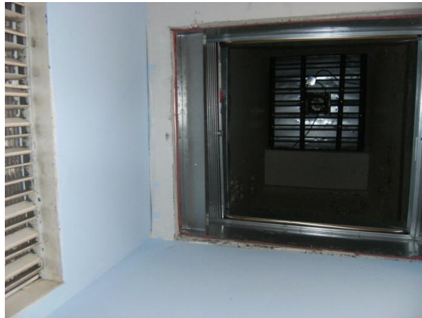
Figure 15: 1961 Wing Exhaust Shaft
