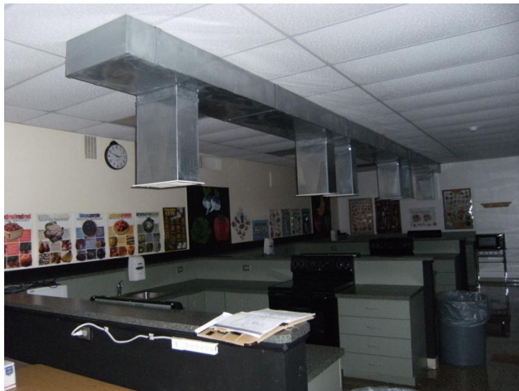
Figure 25: Home and Careers Exhaust Ductwork
