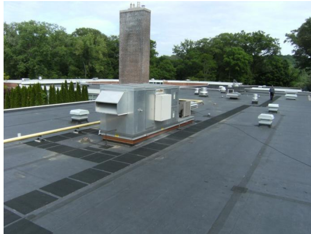
Figure 5: Administration Roof Top Unit
