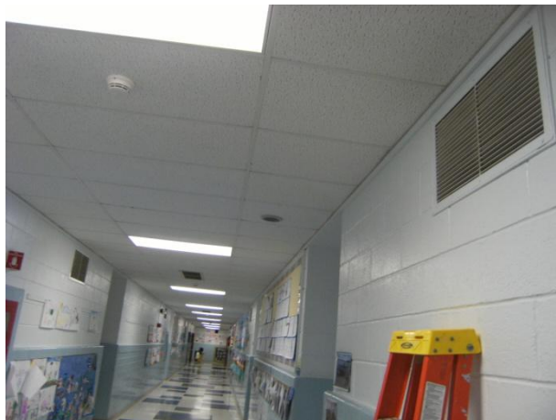
Figure 3: 1954 Wing Classroom - Corridor Air Transfer Grille
