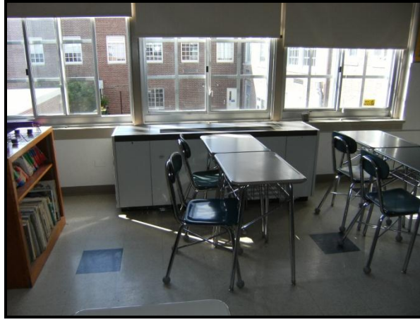
Figure 32: Room 214 Unit Ventilator
