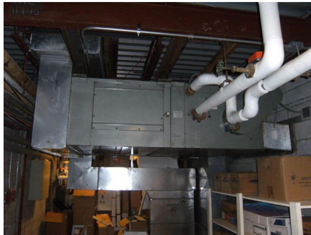
Figure 10: Gymnasium Air Handler
