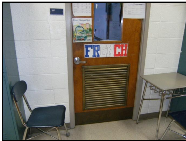
Figure 33: Air Transfer Grille into Corridor
