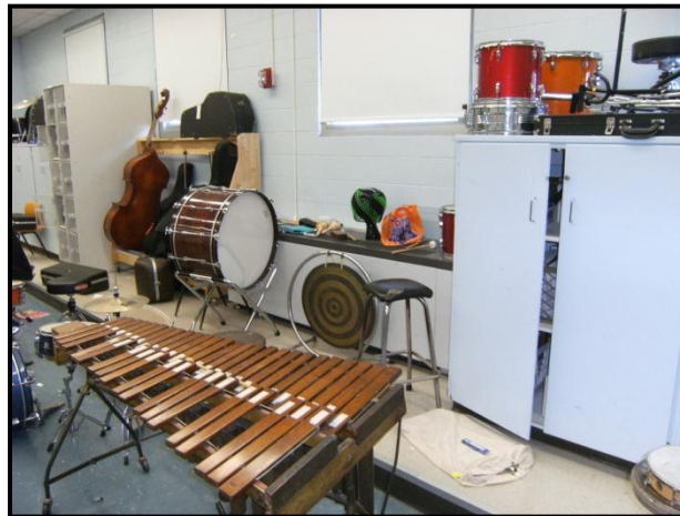
Figure 36: Music/Choral Room Unit Ventilator
