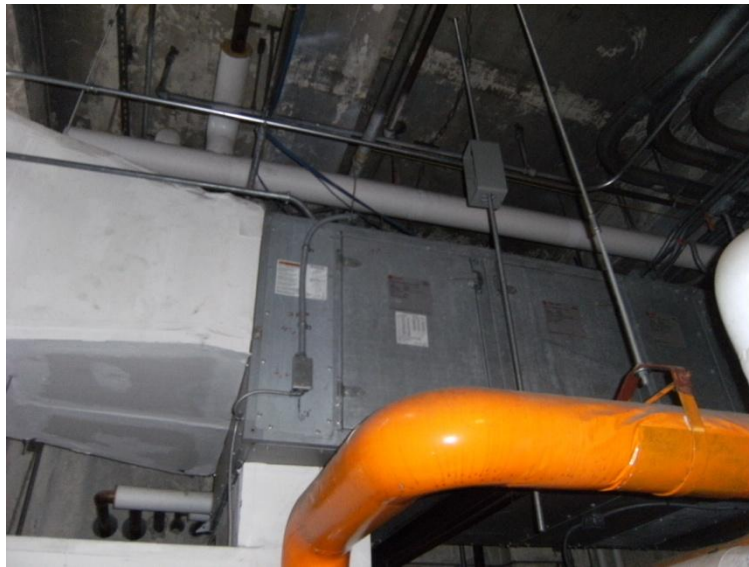
Figure 24: Home and Careers Air Handler
