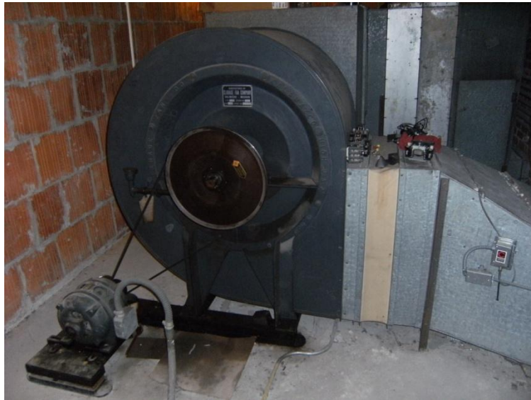
Figure 27: Gym Supply Fan
