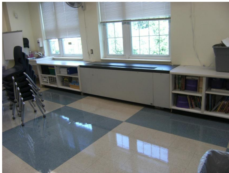
Figure 29: Typical 2004 Addition Classroom Unit Ventilator
