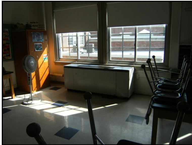
Figure 31: Original Building Typical Unit Ventilator
