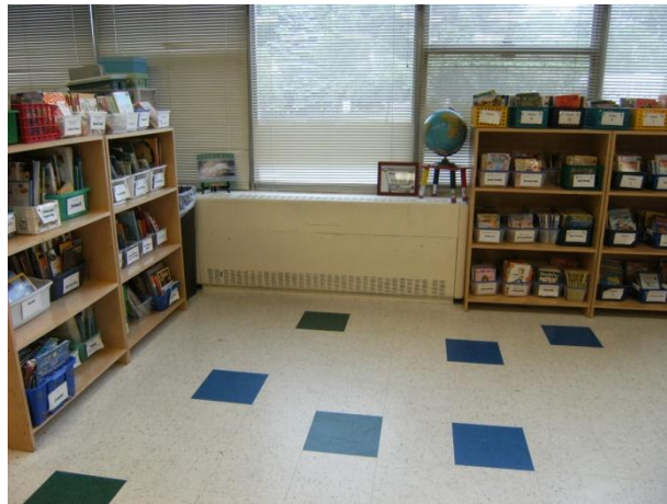
Figure 13: 1961 Wing Unit Ventilator
