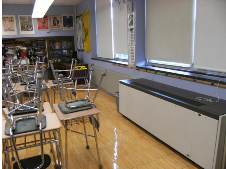
Figure 22: Typical Classroom Unit Ventilator
