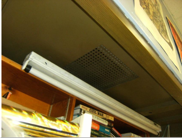
Figure 23: Typical Classroom Closet Exhaust Register
