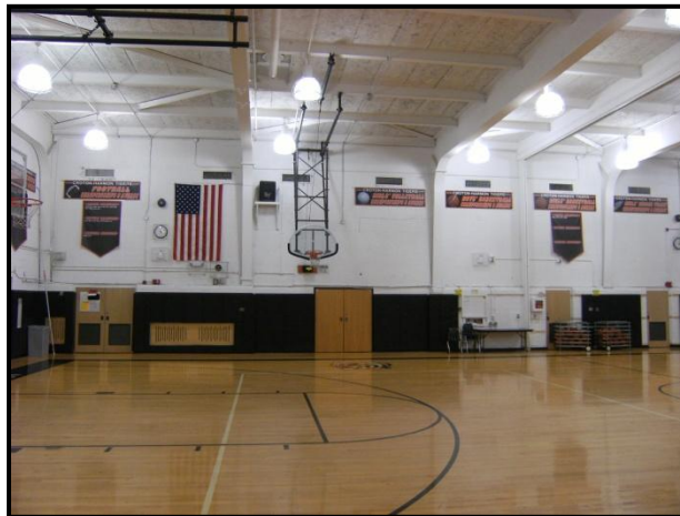
Figure 34: 1960's Gym High Supply Air and Low Return Outlets
