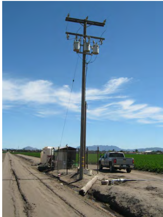
Photograph 5: View of pole-mounted transformers and pumping station adjacent to the south of the site.
