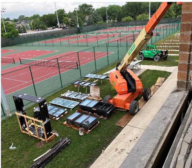
Left: The window installation team continues progressing while dodging this week's storms.
