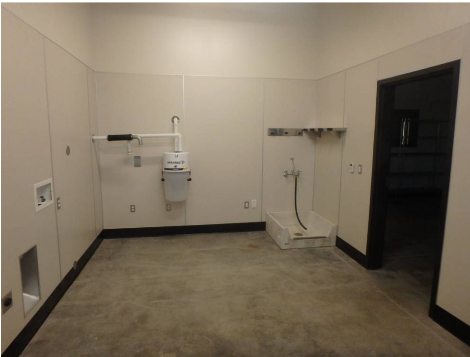
Kennel Room vacuum and janitor sink on the north wall
