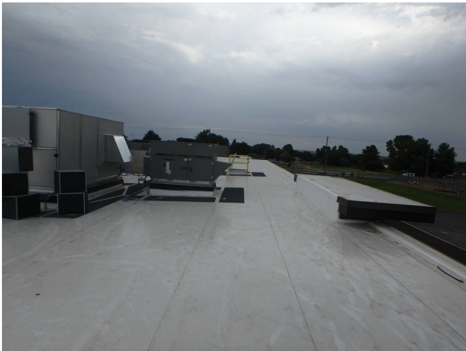
Looking north along the east edge of the roof and hatch beyond (7/10/23)
