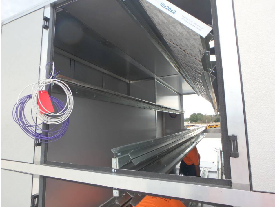
ERV Interior and installing filters (7/10/23)
