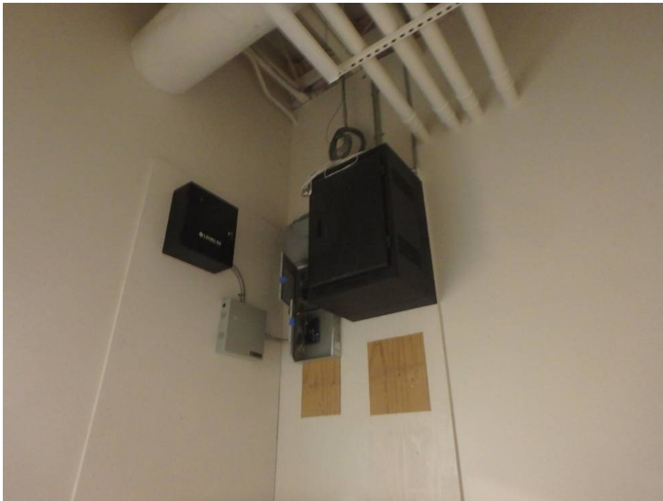
Storage room backboard and equipment, relocated lower panels to north wall - paint
