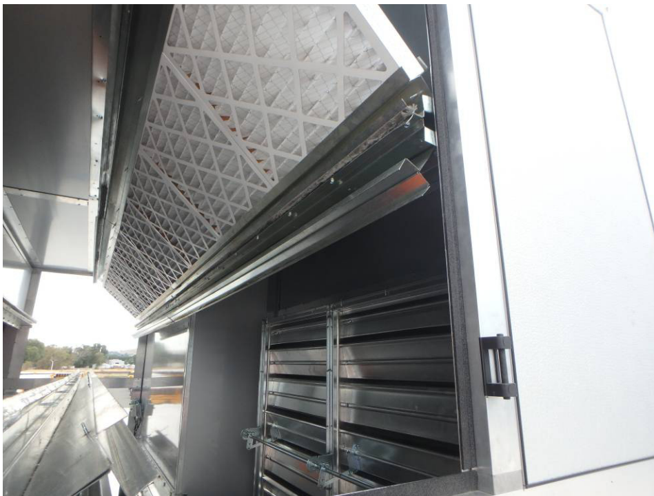
ERV Interior and installing filters (7/10/23)
