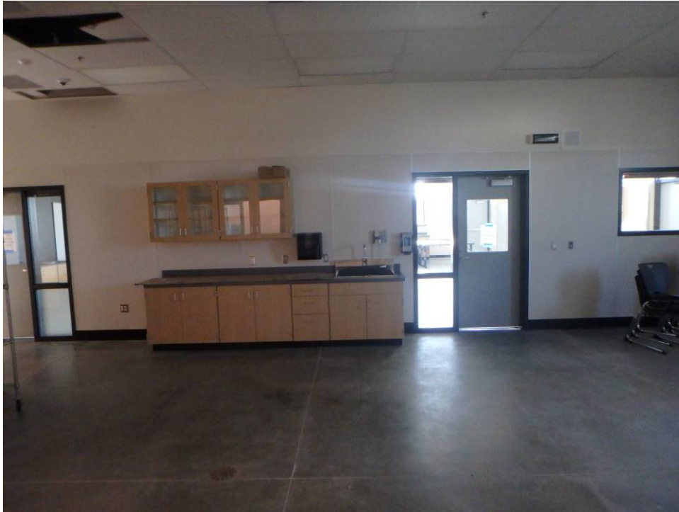
Lab – eyewash station and east wall
