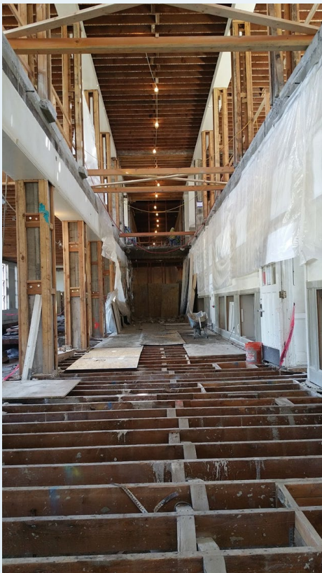
Removal of second floor, due to non-conforming concrete and concrete in columns
