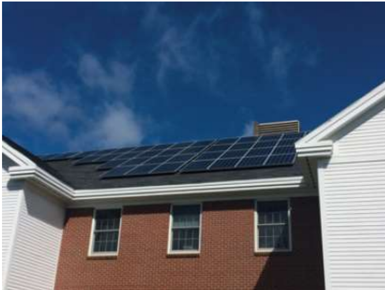
Solar Panels on Ivey Science Center
