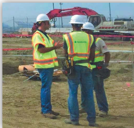
PCI PLA and Labor Compliance Team on the Port of Long Beach Middle Harbor Phase 2 and 3 with local Long Beach apprentices. Top: Juan Alcaraz, Local Resident Apprentice; Rasien Ibanez, PCI PLA & LCP Bottom: Dan Sloan, PCI PLA & LCP, Shawn Wise and Alberto Aaguirre, Local Resident Apprentices.
