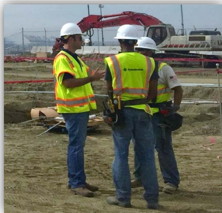
PCI PLA and Labor Compliance Team on the Port of Long Beach Middle Harbor Phase 2 and 3 with local Long Beach apprentices. Top: Juan Alcaraz, Local Resident Apprentice; Rasien Ibanez, PCI PLA & LCP Bottom: Dan Sloan, PCI PLA & LCP, Shawn Wise and Alberto Aaguire, Local Resident Apprentices.
