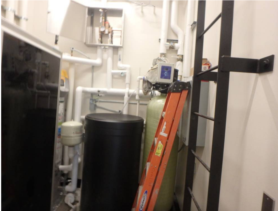
Mechanical room –water softener and brine tank
