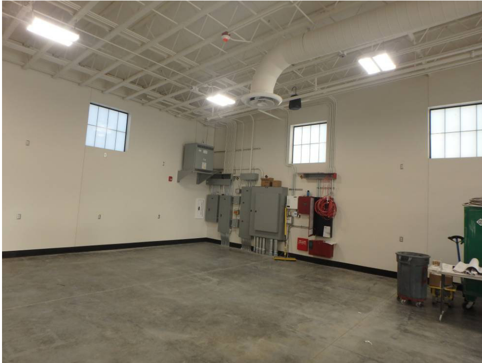
Looking northwest towards the shop's electrical panels and transformer mounted on the wall
