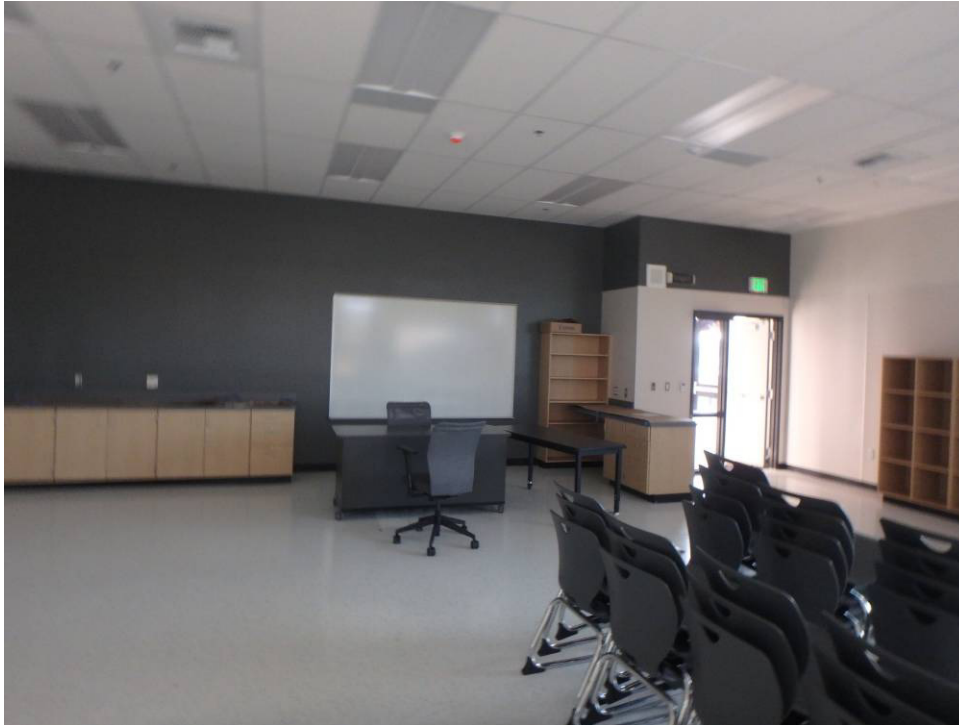
Looking at the casework at the northeast corner of the south classroom
