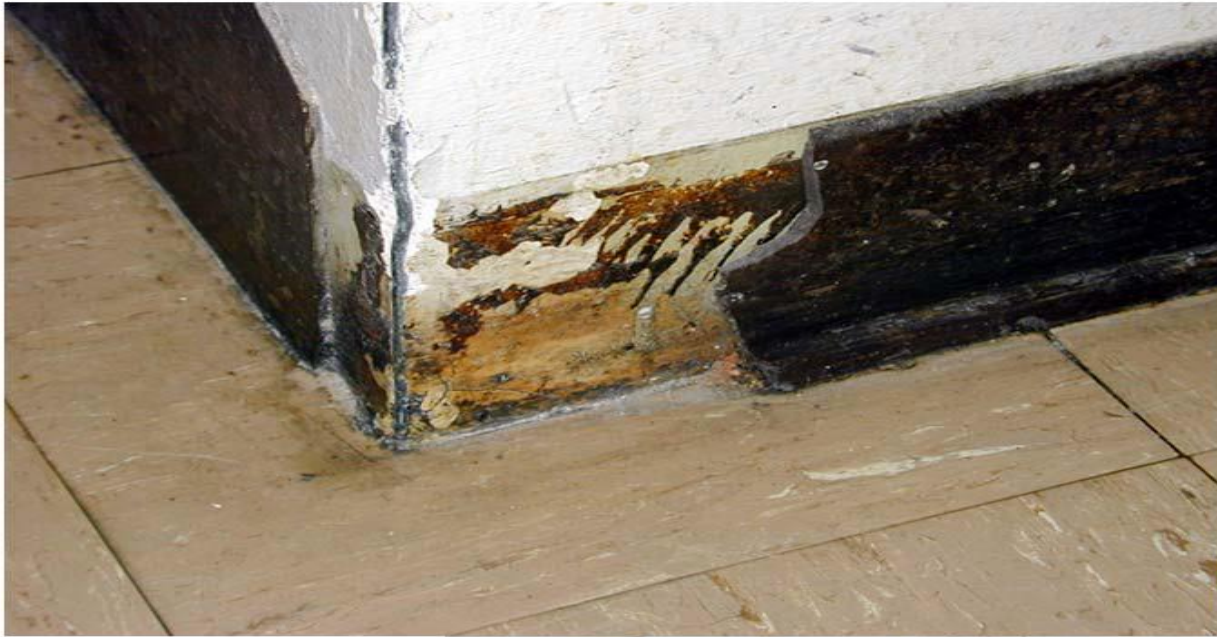
EXPOSED MASTIC UNDER 4" RUBBER WALL BASECOVE
