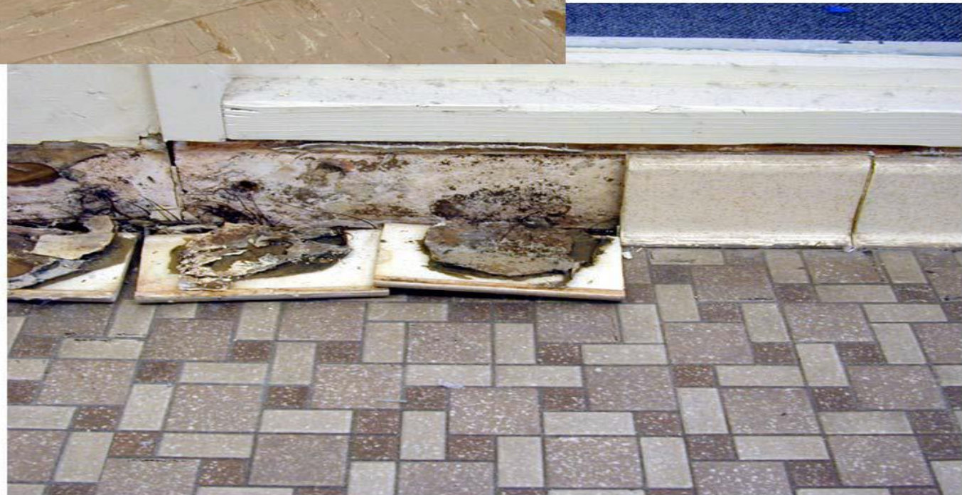
EXPOSED MASTIC UNDER CERAMIC WALL TILE
