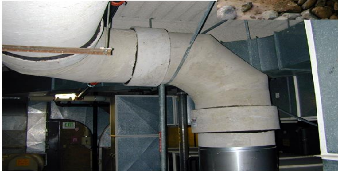
ASBESTOS CEMENT LAB FUME HOOD EXHAUST DUCT
