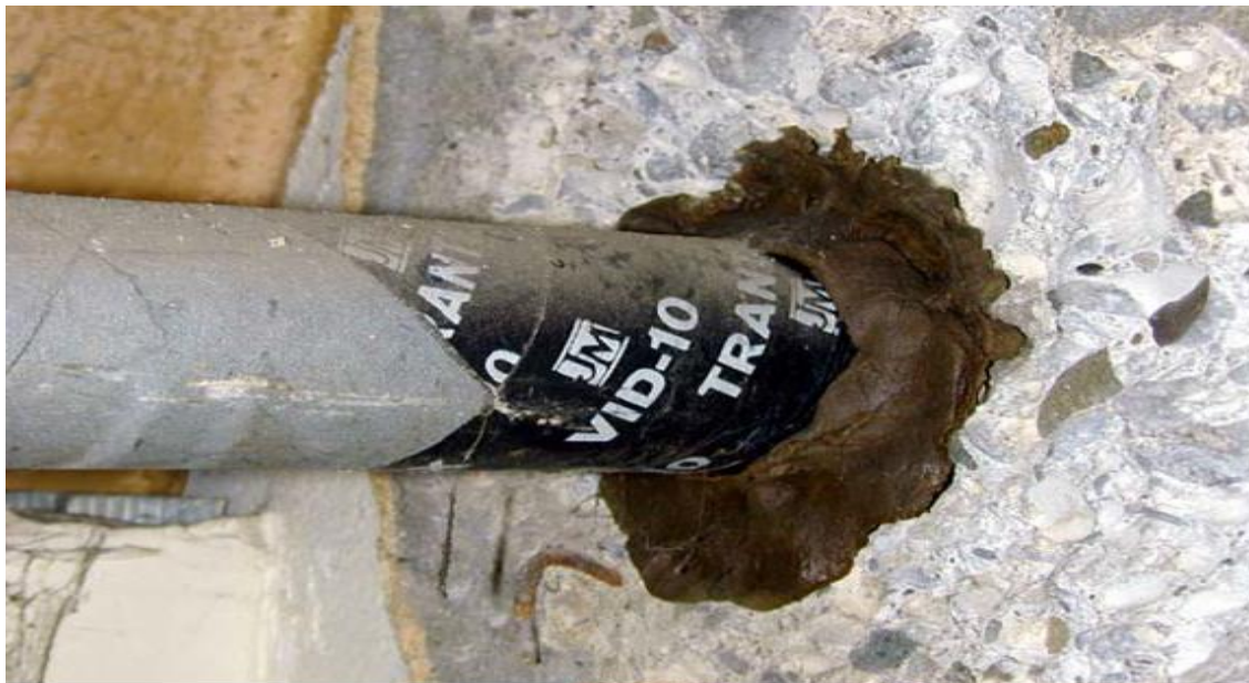
BROWN CAULK AT PIPE PENETRATION
