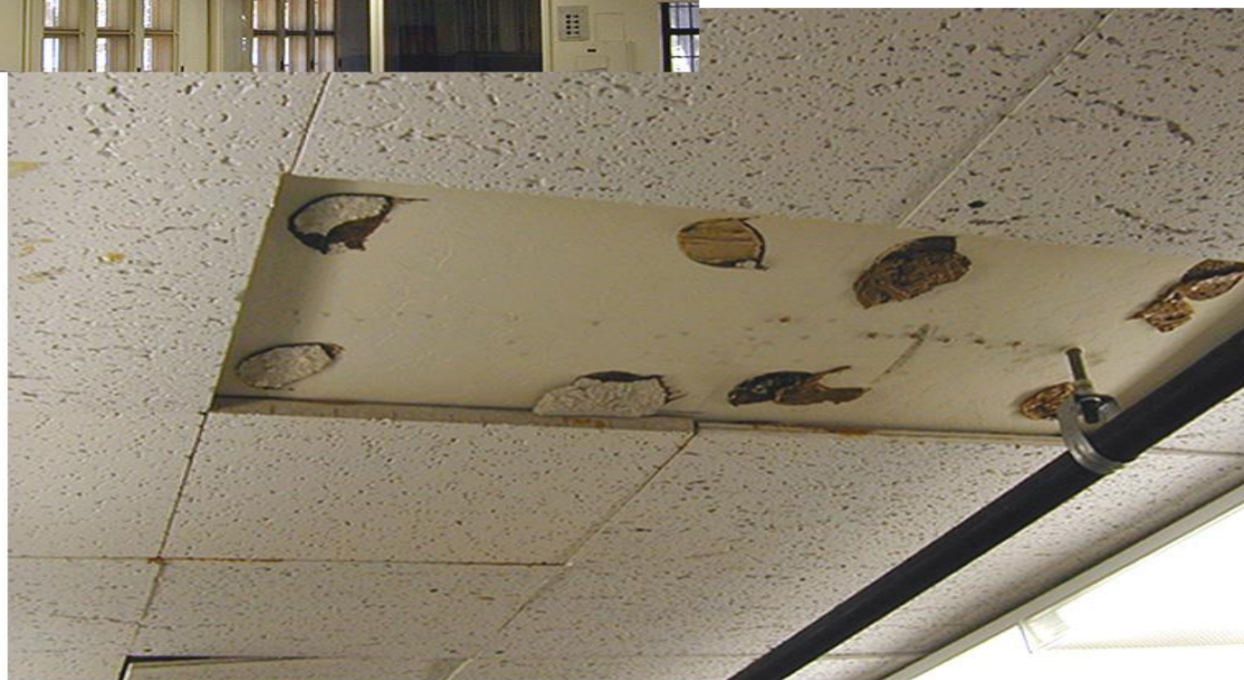
GLUE-ON ACOUSTIC CEILING TILE & EXPOSED BROWN MASTIC
