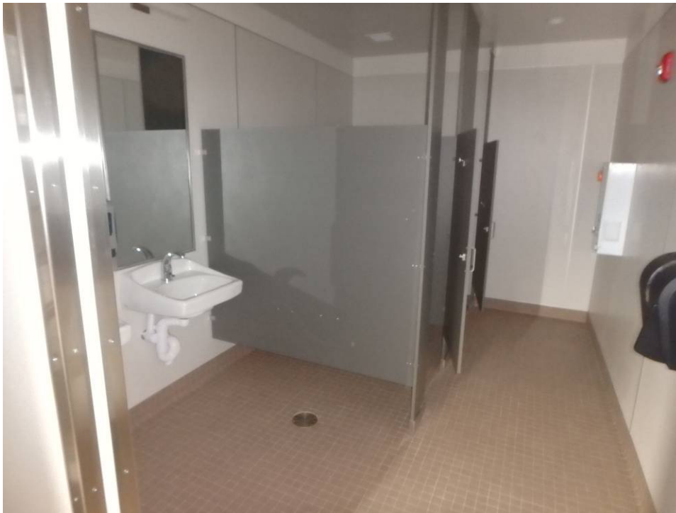
Typical restroom sinks
