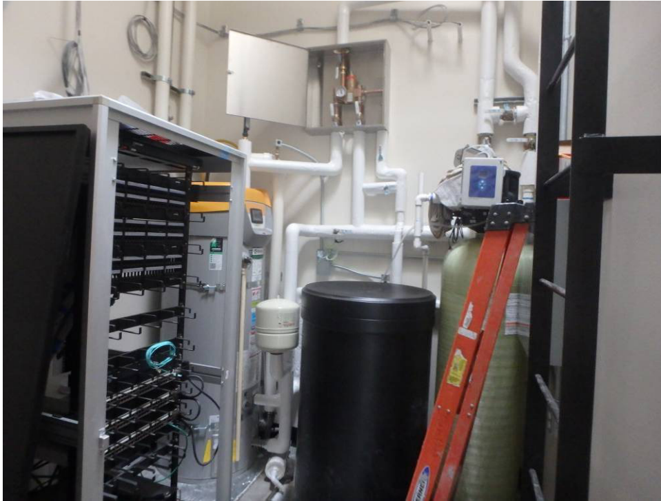
Mechanical room –water softener and brine tank
