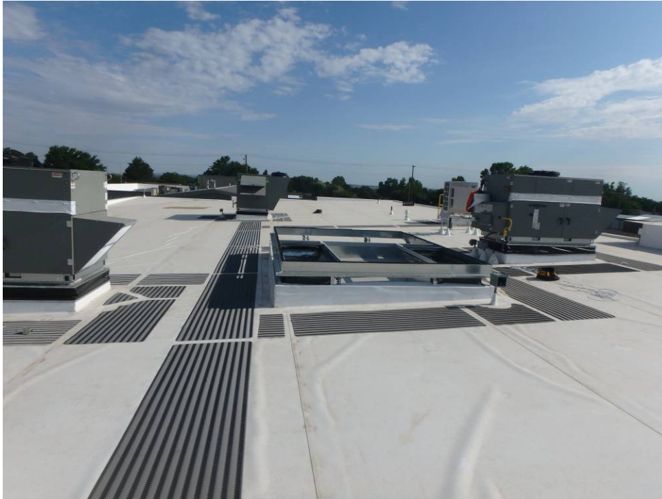
Ready for the DOAS air handler unit (6/27)
