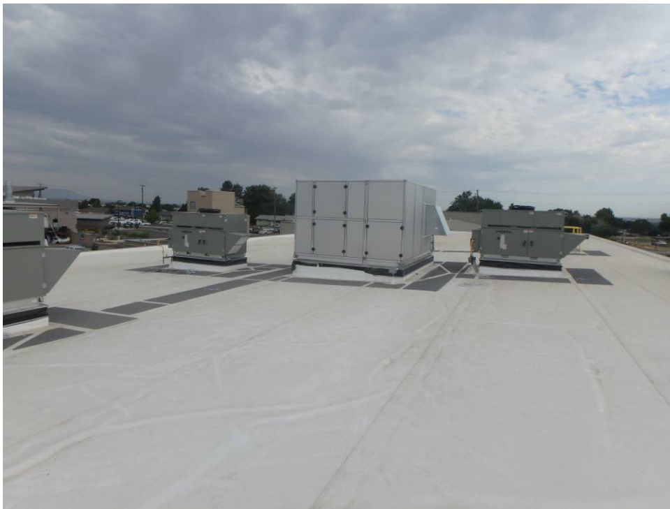
DOAS from the south
