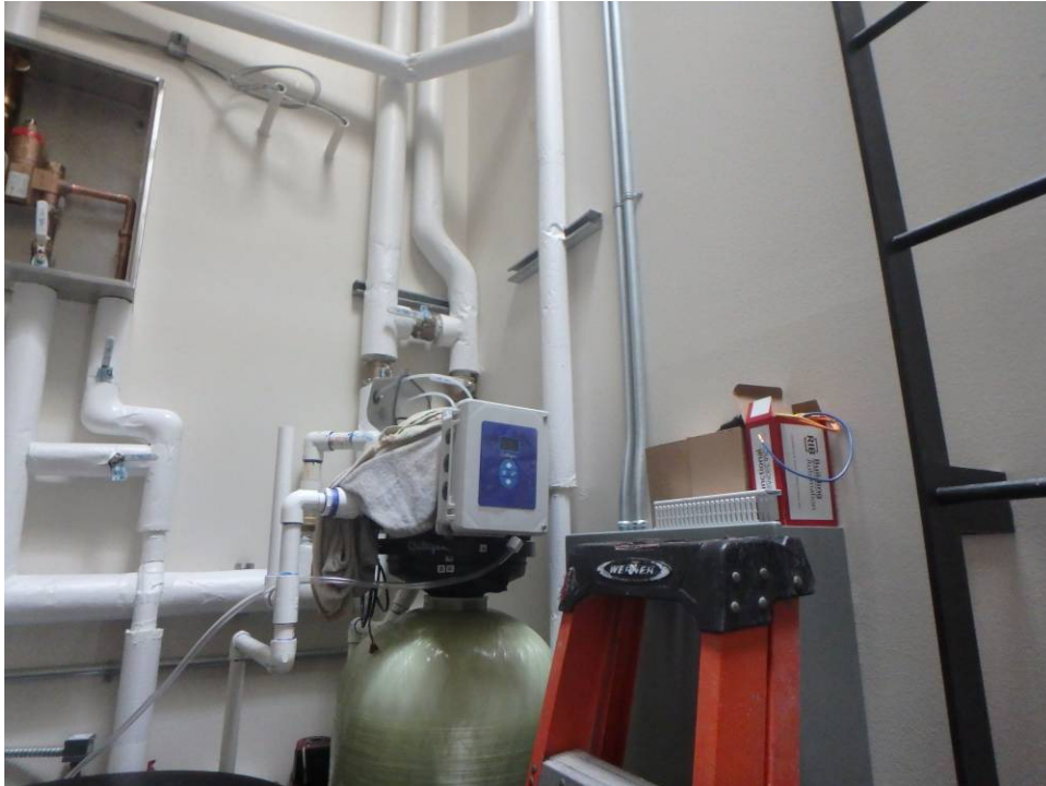
Mechanical room –wall above the water softener and brine tank and ladder
