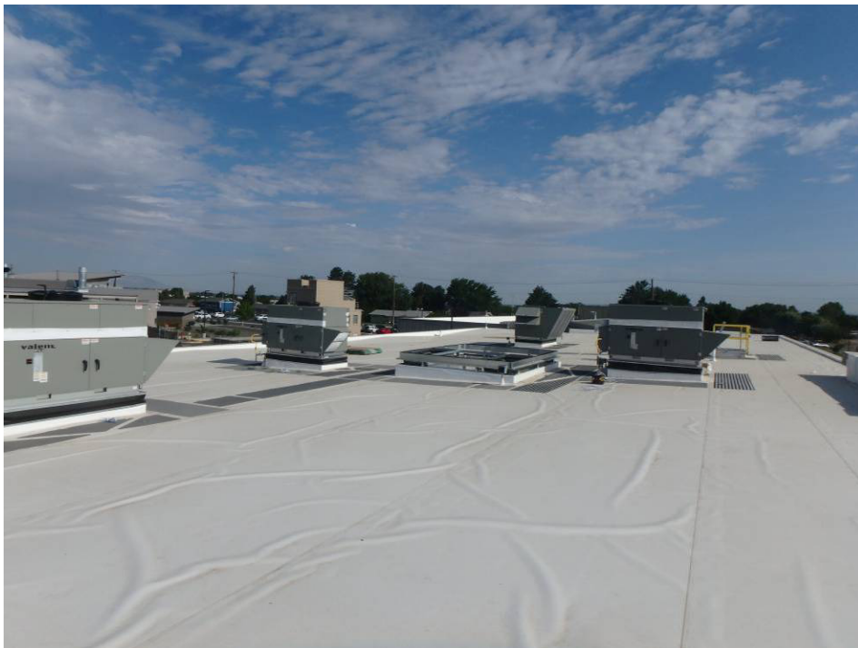
Looking northwest at the DOAS location (6/27)
