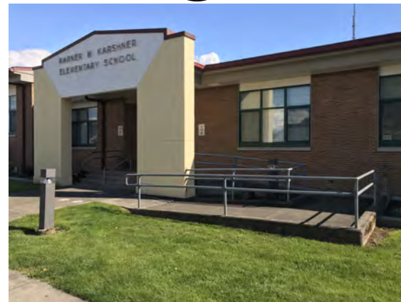
The front door on 8th Ave N.W. is locked during school hours, ring bell to acquire access. Note that the ramp does not meet ADA standards.
