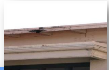
#19 WOOD DETERIORATION AT GYM
