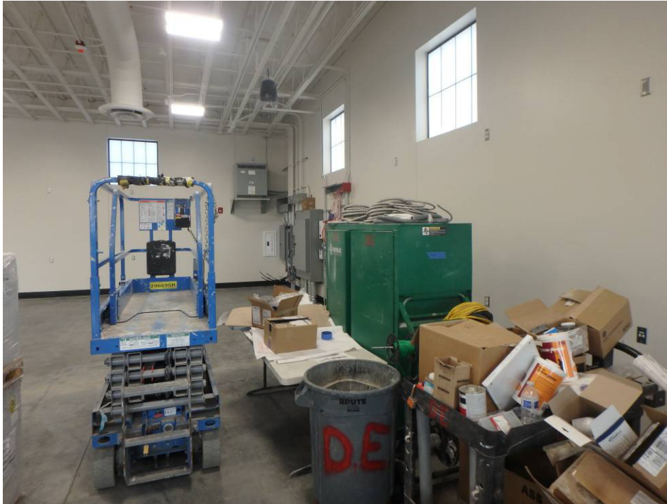
Looking west towards the shop's electrical panels and transformer mounted on the wall
