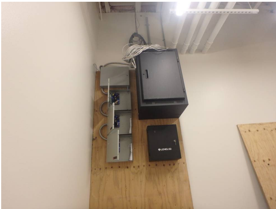
Storage room backboard and equipment, relocate lower panels to north wall, and raise
