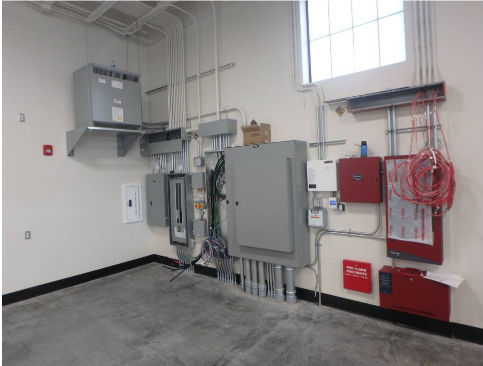
Electrical panels and transformer
