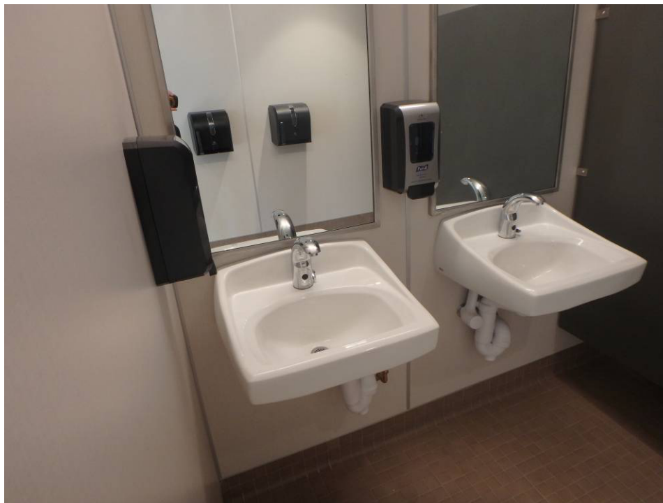
Typical restroom sinks
