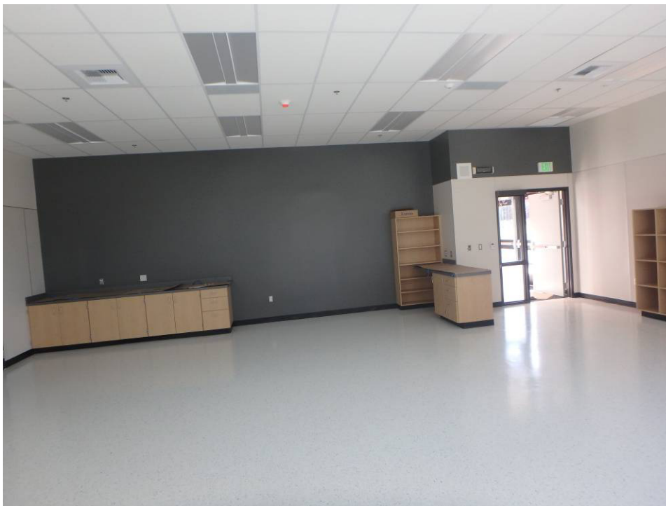
Looking at the casework at the north wall of the south classroom
