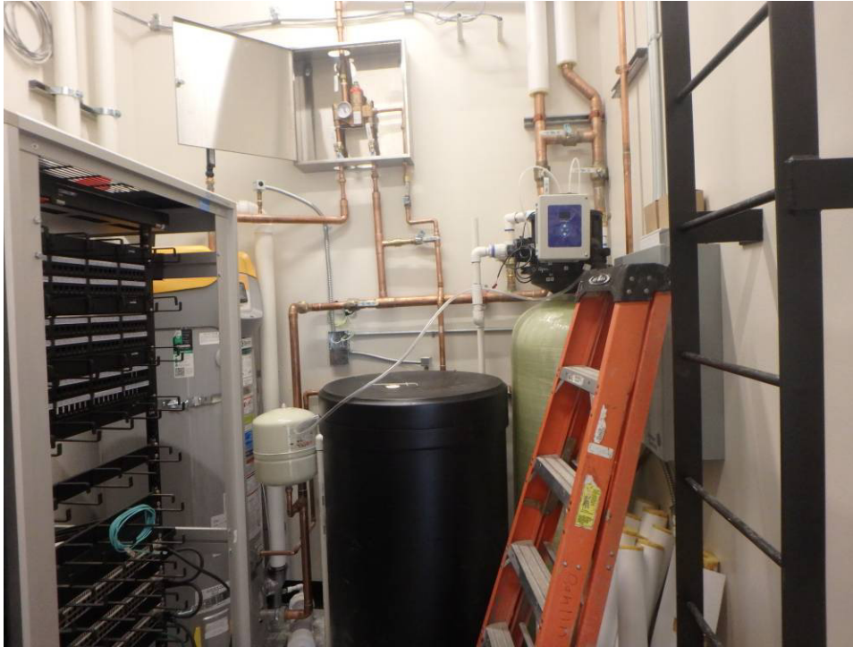
Mechanical room –water softener and brine tank
