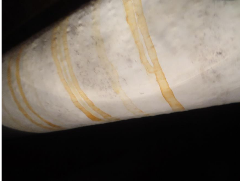
Figure 5: Suspected microbial growth on pipe insulation in tunnel near Classroom #2
