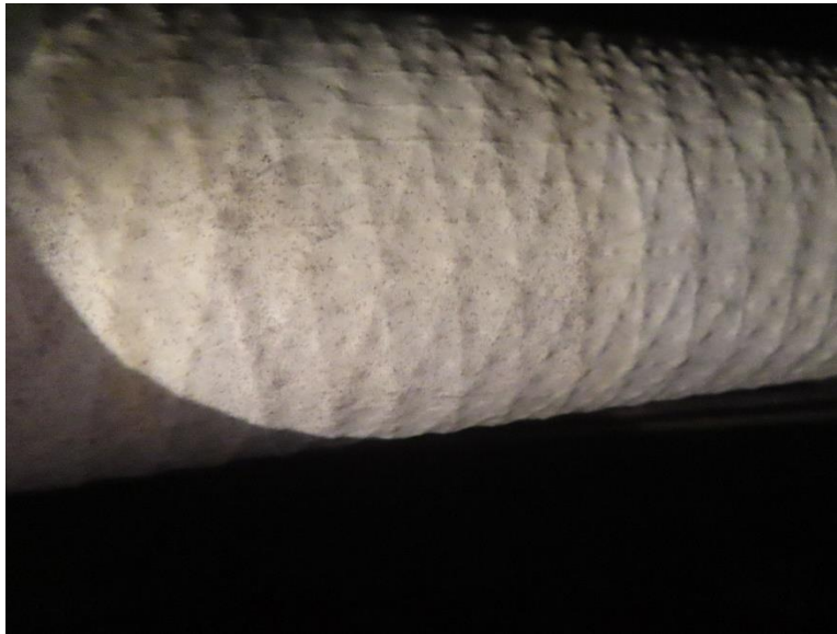
Figure 4: Suspected microbial growth on pipe insulation in tunnel near Classroom #2
