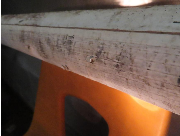
Figure 7: Suspected microbial growth on pipe insulation in tunnel near Classroom #2
