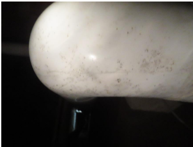
Figure 6: Suspected microbial growth on 90° plastic elbow in tunnel near Classroom #2
