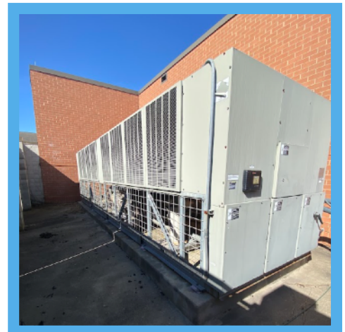
Middle School HVAC system
