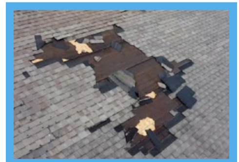
High School Roof Damage on March 30th
