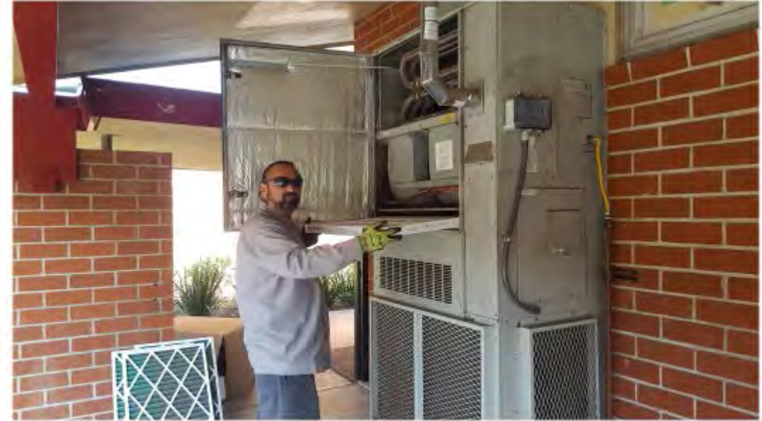
Dale from Facilities ensures the air conditioning is ready for the start of school and the return of students.
