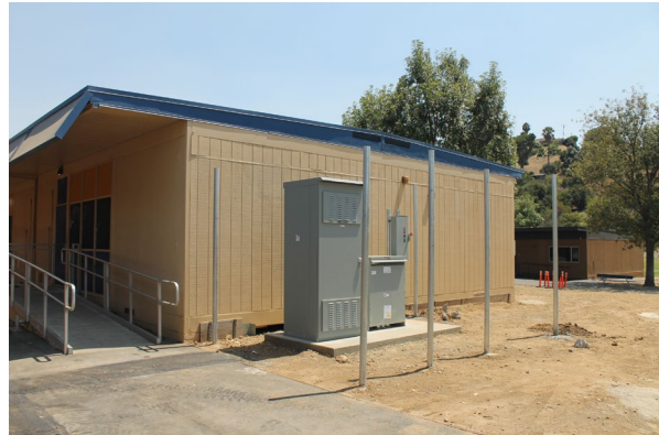
NEW TRANSFORMER & GEAR SET
