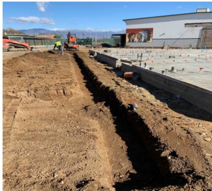
La Puente HS New Kitchen – Digging for New Retaining Wall and Piping
