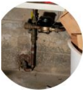
This is an example of a water meter.
