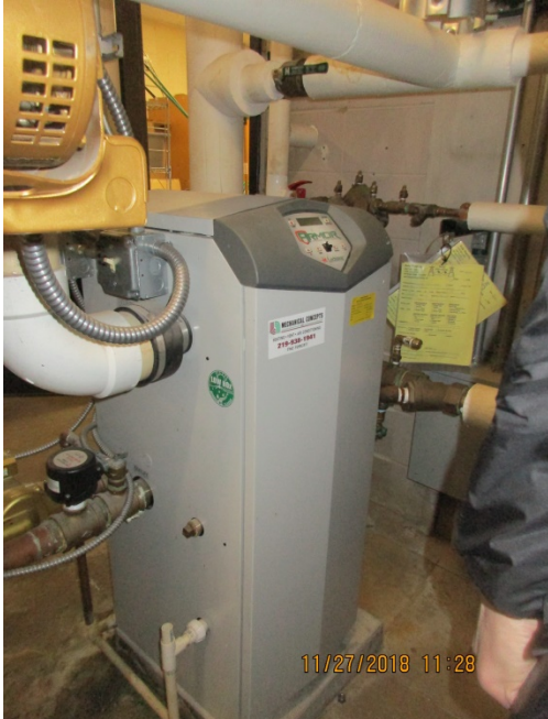
DOMESTIC WATER IS HEATED BY A HIGH EFFICIENCY UNIT
