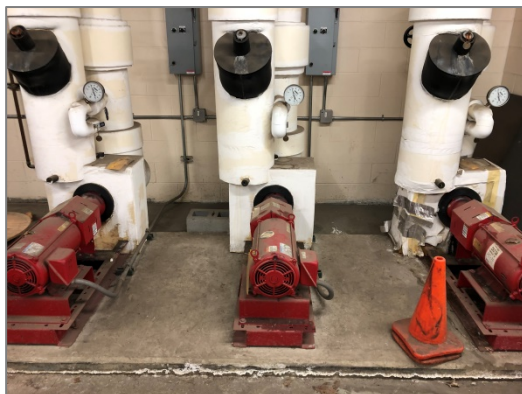
CHILLER DISTRIBUTION PUMPS
