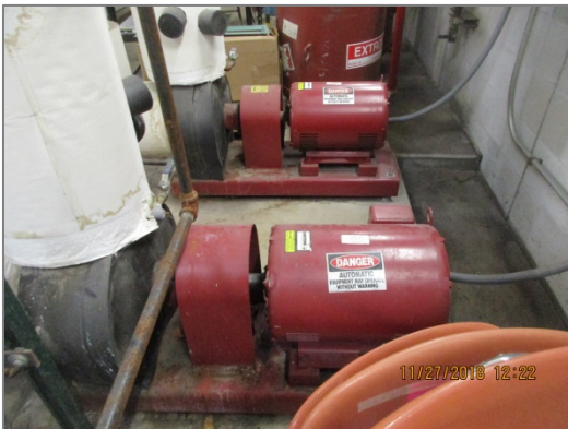
CHILLER DISTRIBUTION PUMPS
