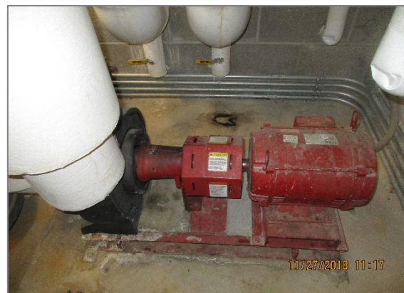
ONE OF 2010 CHILLER DISTRIBUTION PUMPS
