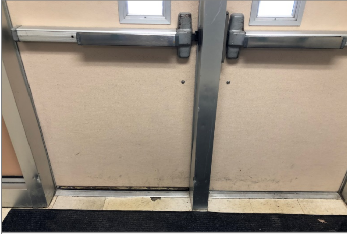
SOME DOOR THRESHOLDS NEED ATTENTION
