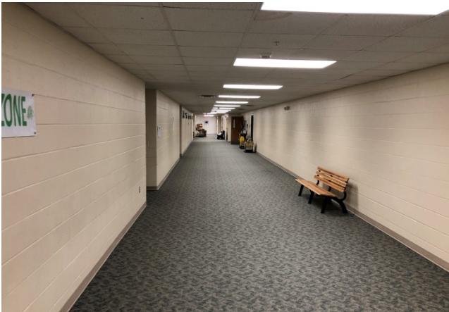
FLUORESCENT LIGHT FIXTURES IN CORRIDOR
