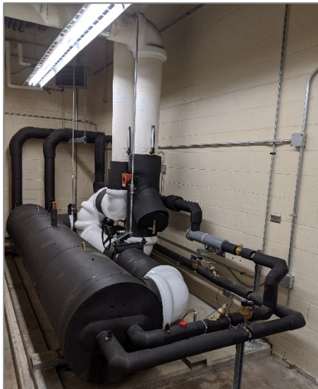
NEW CHILLER INDOOR EVAPORATOR BARREL
