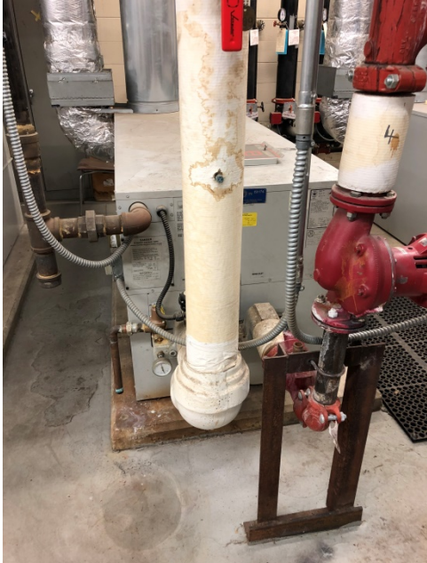
DOMESTIC WATER IS HEATED BY MAIN BOILERS
