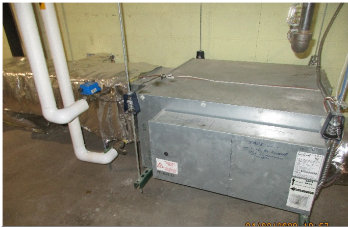
FAN POWERED VAV BOX INSTALLED IN MECHANICAL MEZZANINE
