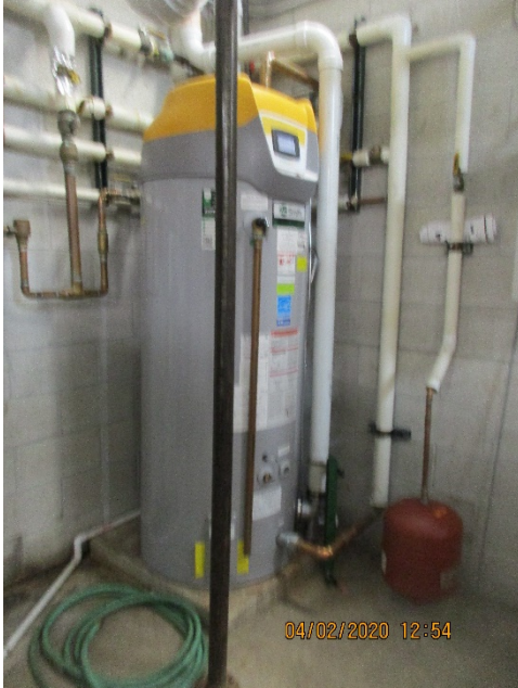
DOMESTIC WATER HEATER
