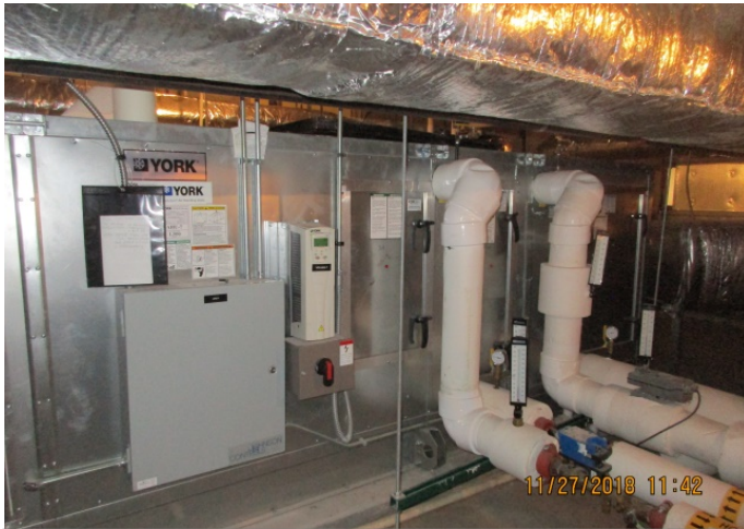
INDOOR YORK AIR HANDLER WITH VFD
