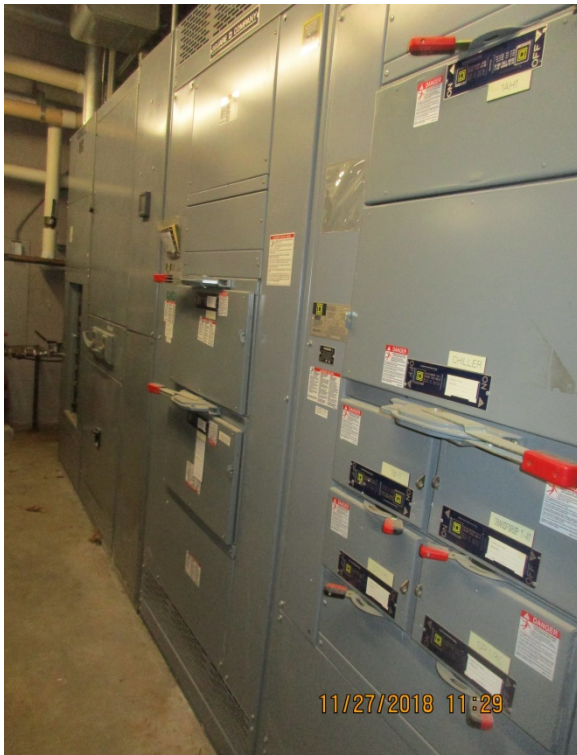
SOME OF THE SWITCHGEAR IS OLDER AND CAUSING OPERATIONAL ISSUES.
