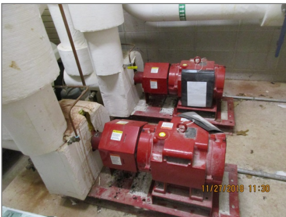
2008 CHILLER DISTRIBUTION PUMPS
