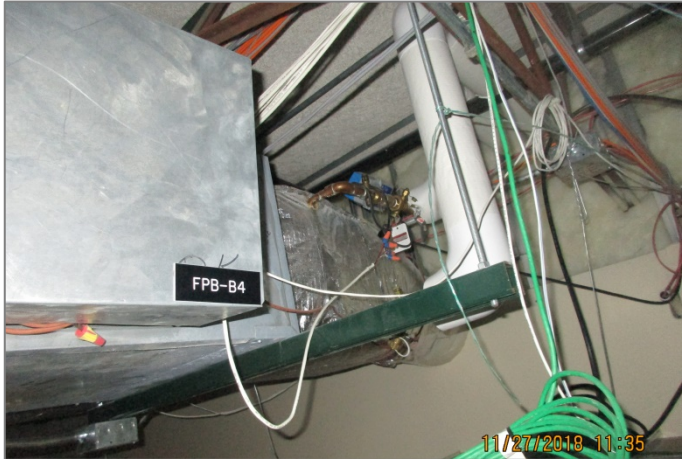
FAN POWERED VAV BOXES ARE INSTALLED ABOVE THE CEILING AND ARE DIFFICULT TO SERVICE (LADDER WORK)
