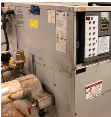
EXISTING BOILER SHOWING SIGNS OF WEAR AND TEAR
