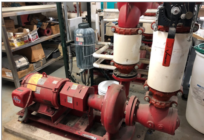
BOILER DISTRIBUTION PUMPS
