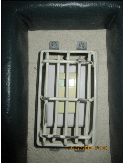
DIGITAL CONTROL SENSOR
