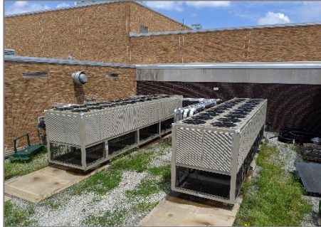
NEW DAIKIN CHILLERS
