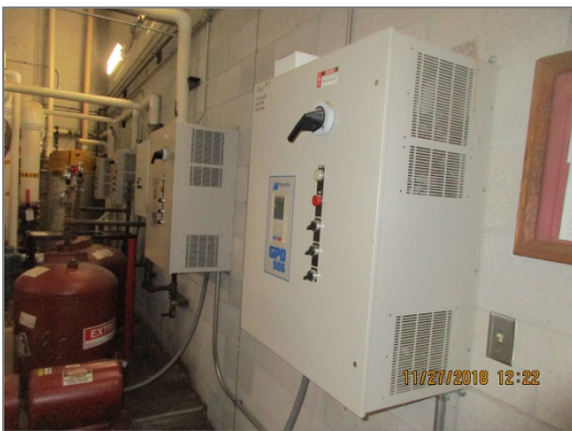
VARIABLE SPEED DRIVES FOR PUMPS
