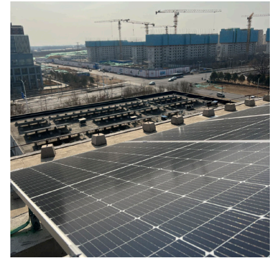
Shunyi Solar Project
