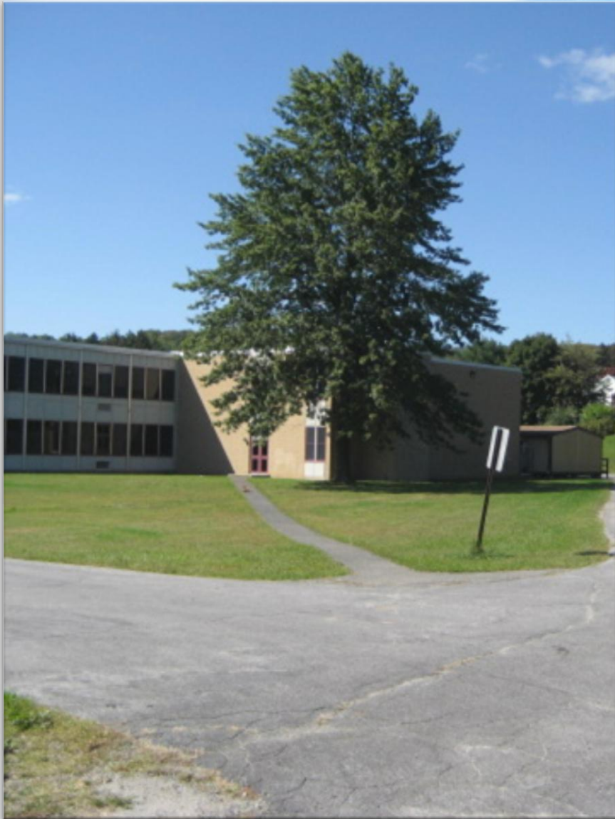
Paving deteriorating in Drives
