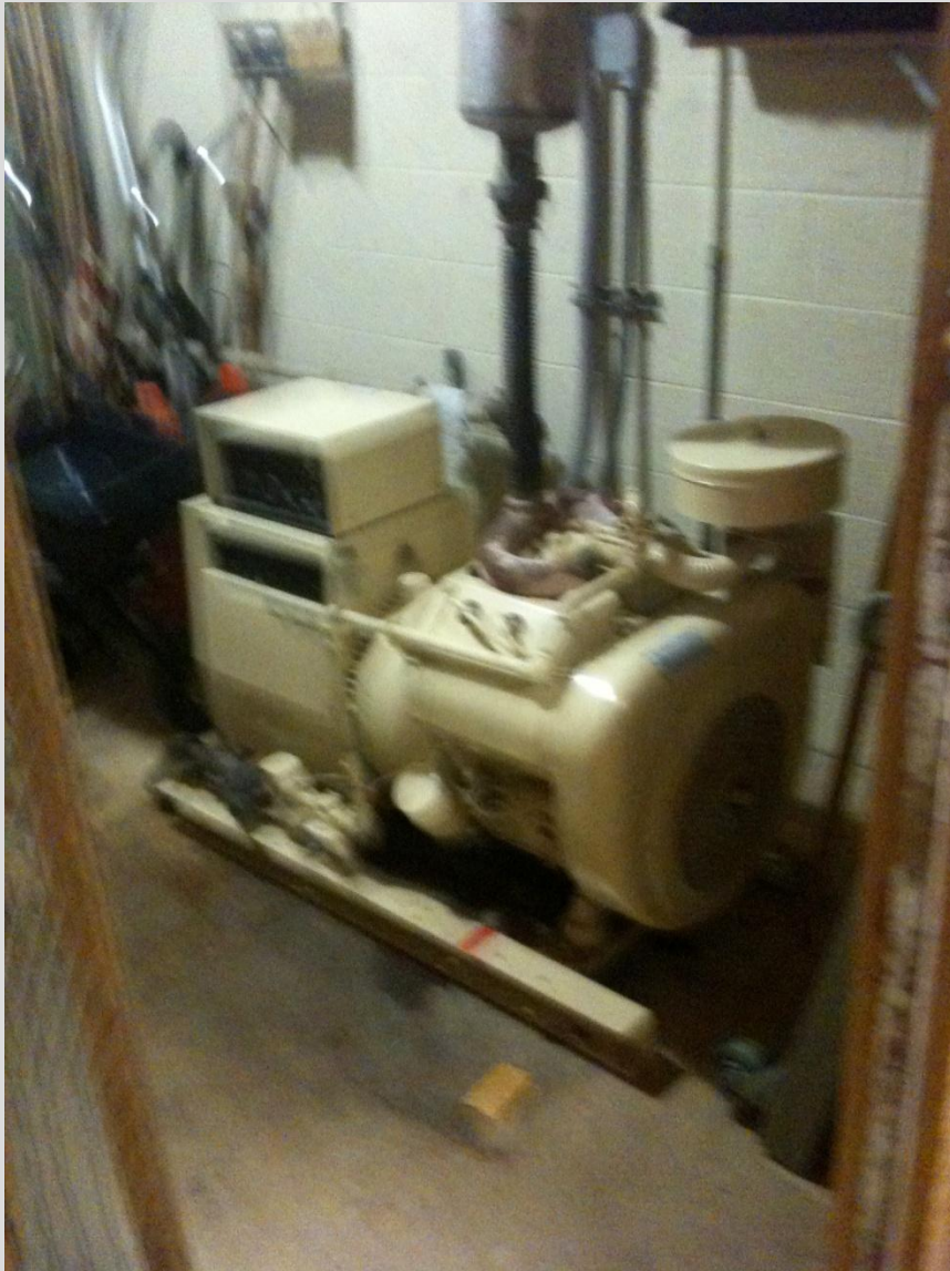
Emergency Generator (Exit Signs and Egress Lighting Only)
