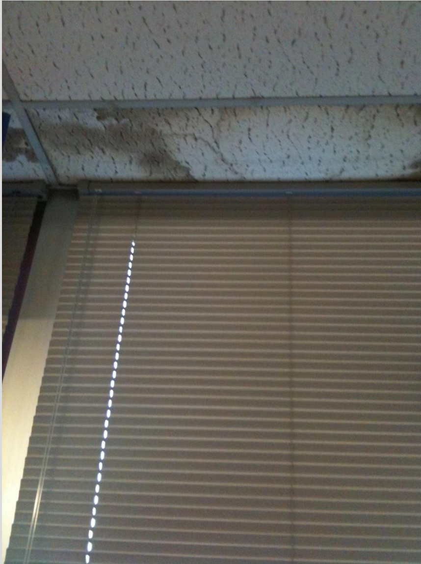
Leaking Curtain Wall System
