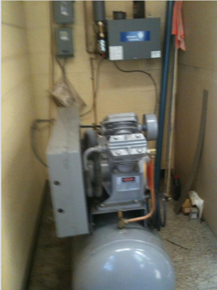
ATC Air Compressor/Air Dryer (pneumatic controls limited outdated technology)
