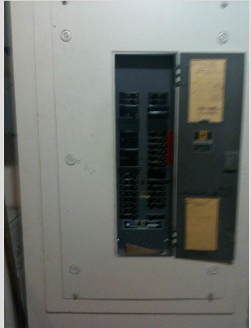
Typical Sub-Main Electrical Distribution Panel (Breakers Overheating Internally)
