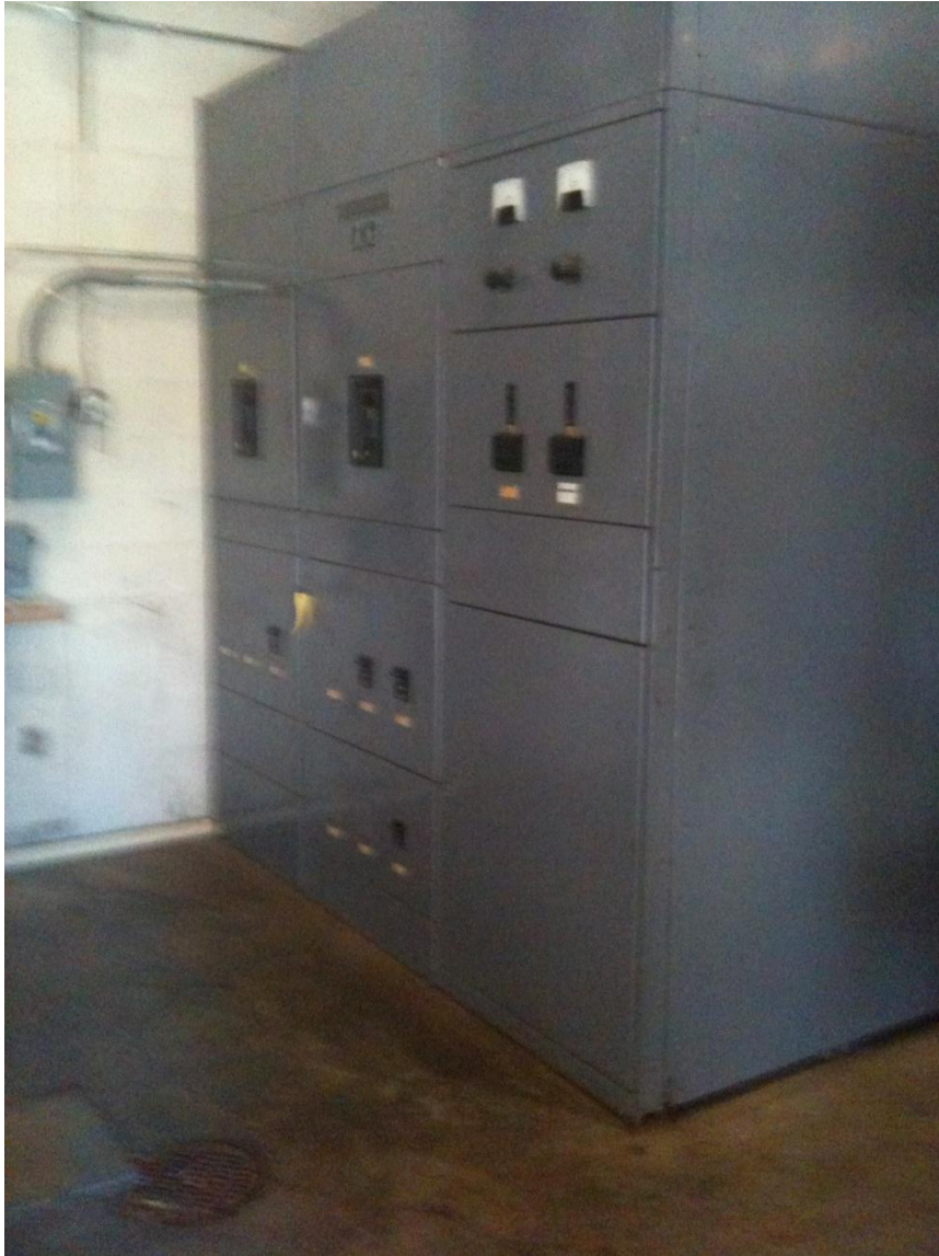
Electrical Main Panel
