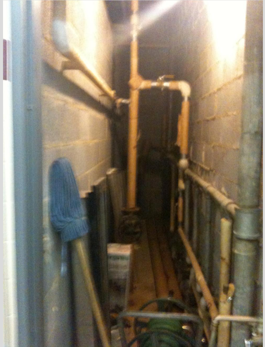
Typical Pipe Chase with Asbestos Insulation
