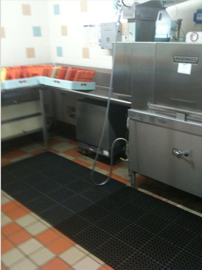
Dishwasher Room (old equipment , floor drain issues through out lower level of building)
