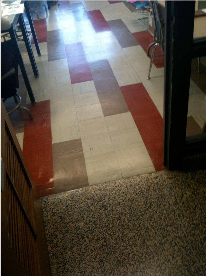
Asbestos Floor Tiles in Classrooms (also underneath carpeted areas)
