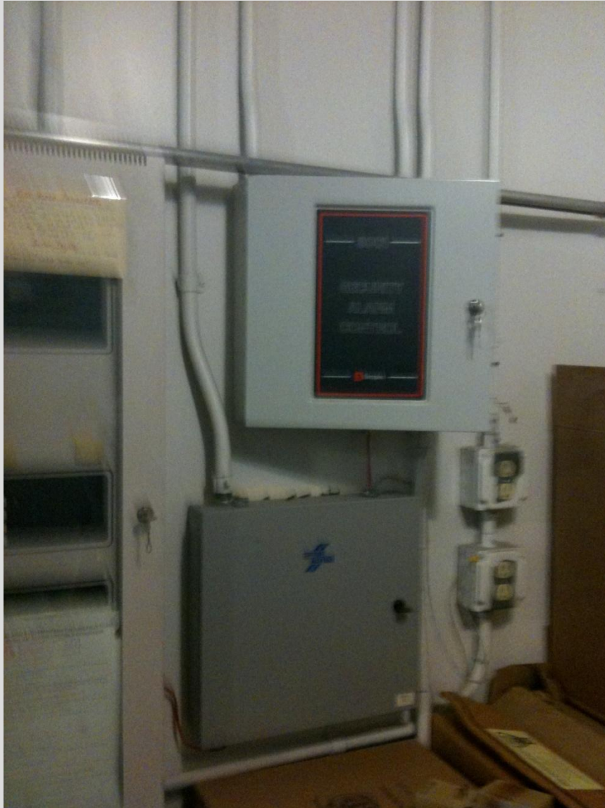
Security Panel (Obsolete Currently to be Replaced)
