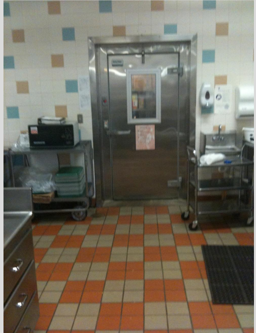
Walk-in Refrigerator/ Freezer (too small)
