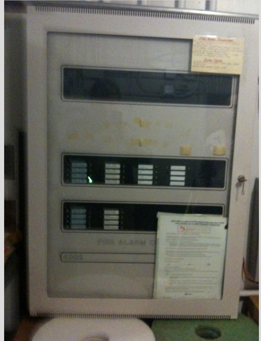
Fire Alarm Panel / Phone Dialer-Non Addressable System (Does Not Meet Current NFPA Code Requirements)
