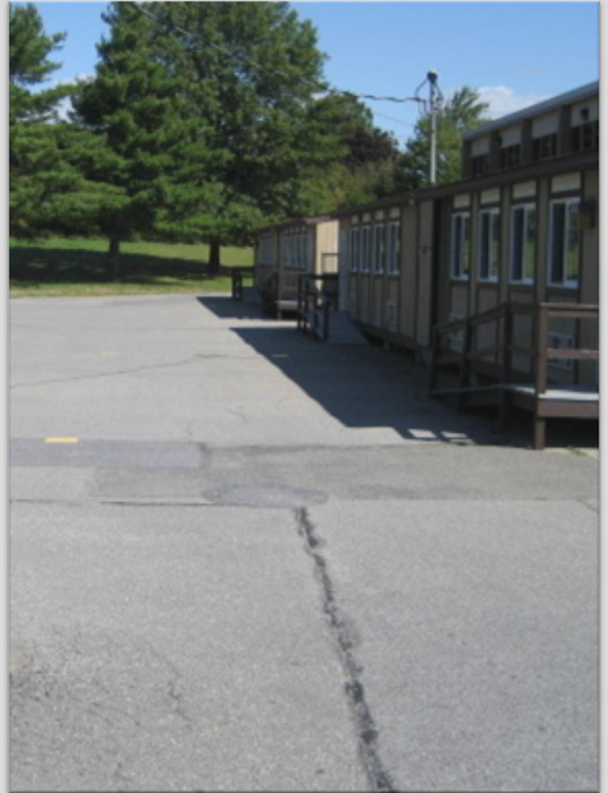
Paving deteriorating in Drives
