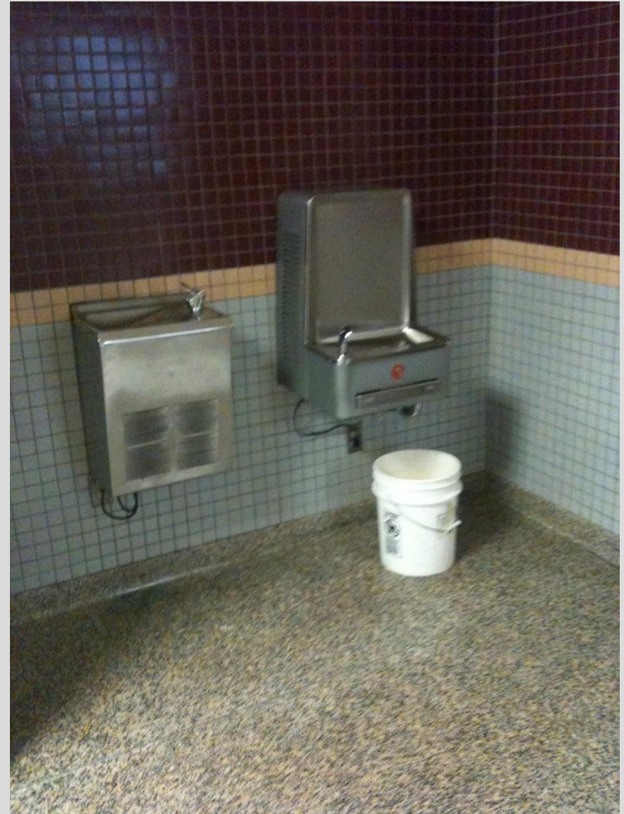
Blocked Drains (in walls and below concrete)
