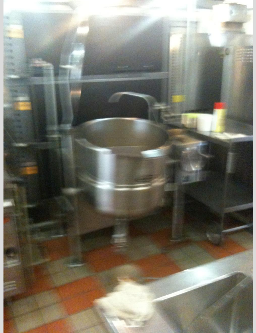
Kitchen Equipment (old)
