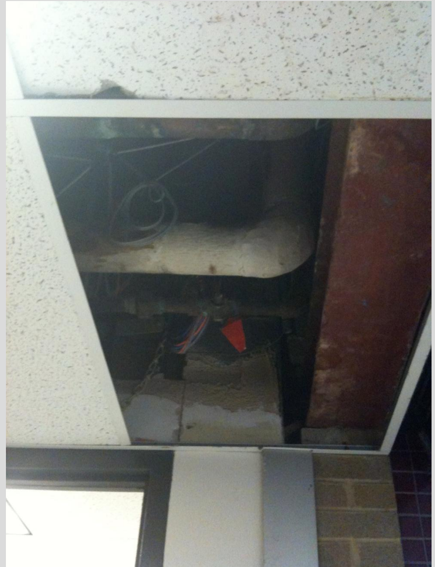
Typical Asbestos Pipe Insulation and Valves Throughout Building (above ceilings etc.) (please note many of the valves leak or are frozen in their current position)
