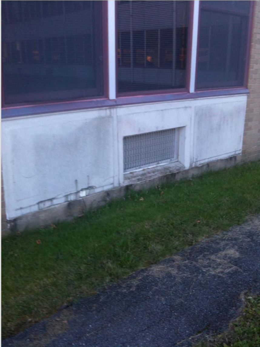
Deterioration of External Dryvit Insulation System and Caulking
