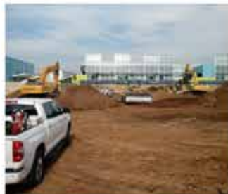
Stormwater Detention System
