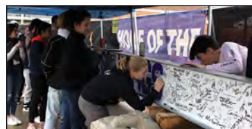
Students signed the last beam before workers lifted it to the top of the two-story structure. The addition will open in fall 2020. More photos: http://bit.ly/LWHSaddition
