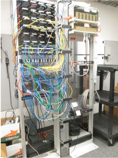
DATA SERVER RACK
