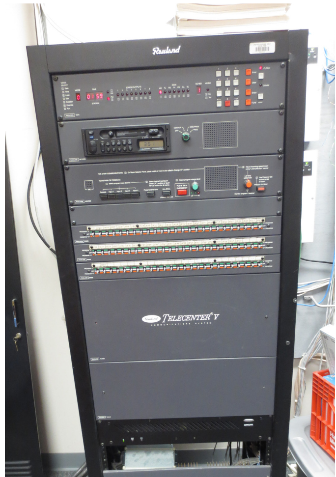
PAGING / BELL CONTROL UNIT
