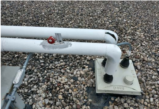
SOLAR ARRAY PIPE INSULATION
