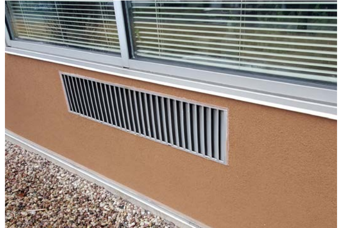
ABANDONED UNIT VENTILATOR OUTSIDE AIR LOUVER
