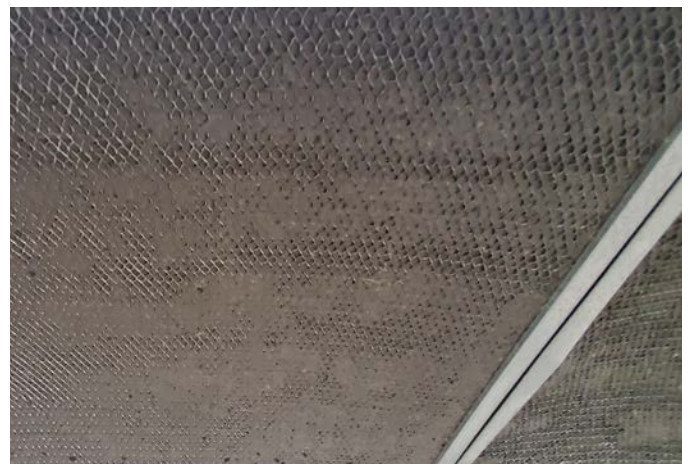
CLOGGED OUTSIDE AIR INTAKE ON DOAU
