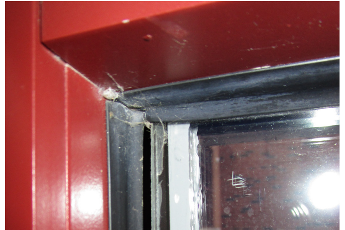
GLAZING PANEL SHIFTED IN WINDOW FRAME
