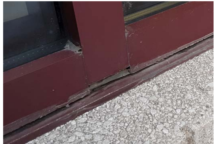
BROKEN SEALANT TRYING TO SEAL WINDOW FRAME
