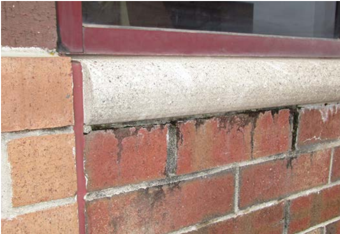
CRACKED MORTAR AT THE EXTERIOR WALL OF THE SOLARIUM
