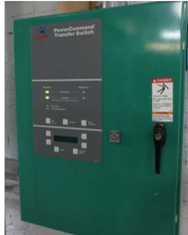
GENERATOR TRANSFER SWITCH
