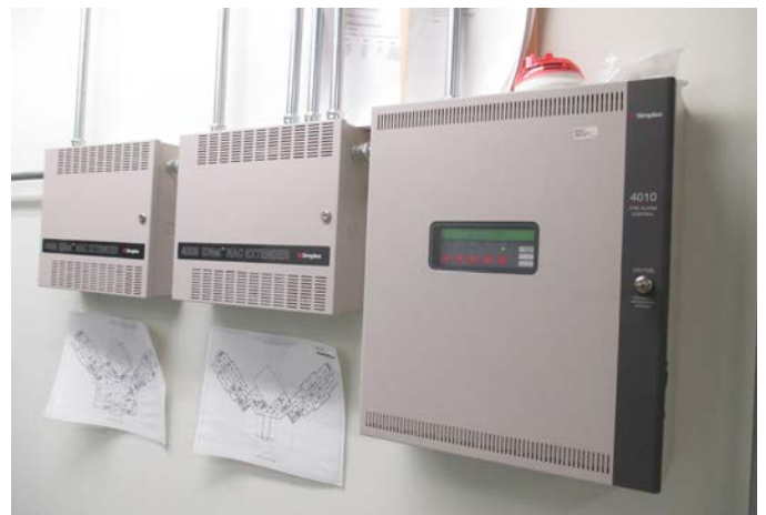
FIRE ALARM CONTROL PANEL AND EXTENDER PANELS
