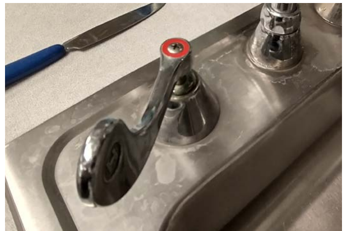
CLASSROOM SINK CALCIUM DEPOSIT
