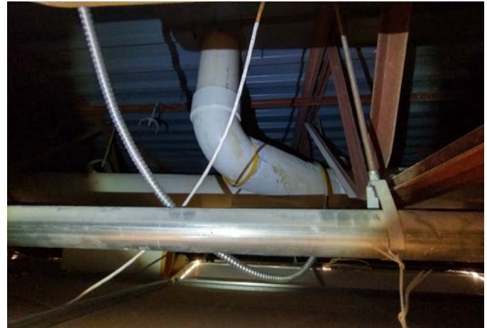
LEAKING ROOF DRAIN
