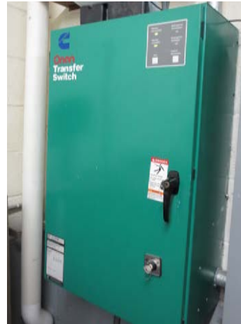
GENERATOR TRANSFER SWITCH
