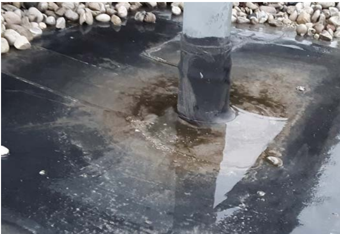
RECESSED ROOFING AT HVAC PENETRATION
