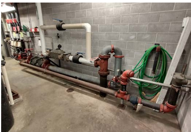
WATER SERVICE ENTRANCE
