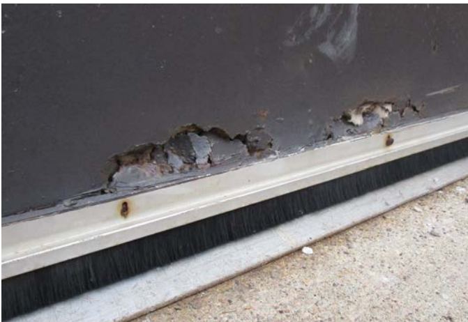
RUSTING HOLLOW METAL DOOR - EXTERIOR
