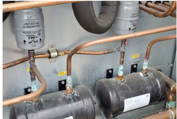
DOAU UNIT DETERIORATION AT MULTIPLE COMPONENTS
