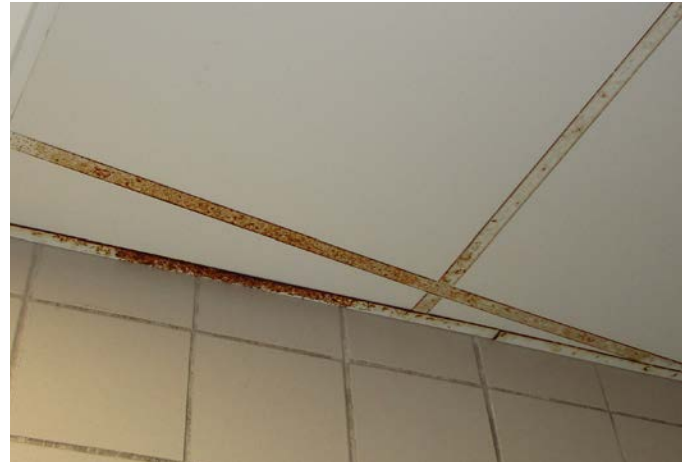
RUSTY LAY-IN CEILING GRID
