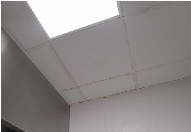
RUSTING DISH ROOM CEILING GRID
