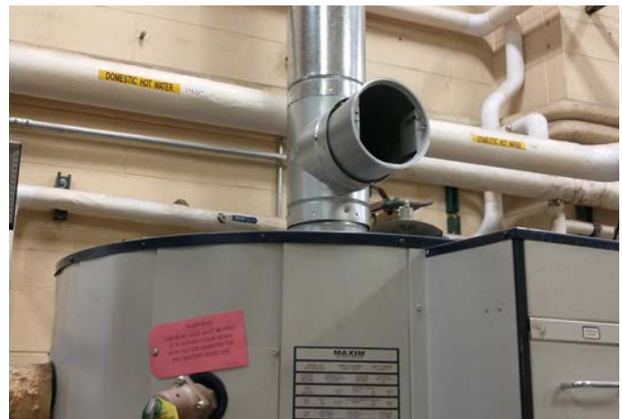
MISSING BAROMETRIC DAMPER
