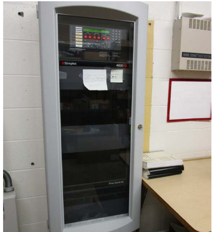
FIRE ALARM CONTROL PANEL
