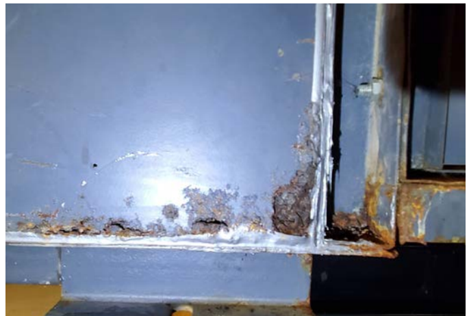
DETERIORATION OF 1976 AHU
