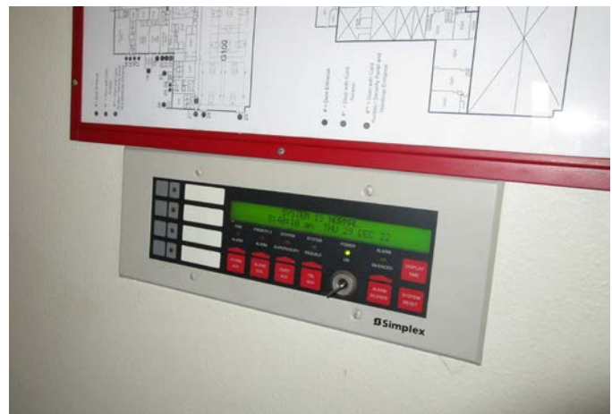
FIRE ALARM ANNUNCIATOR PANEL
