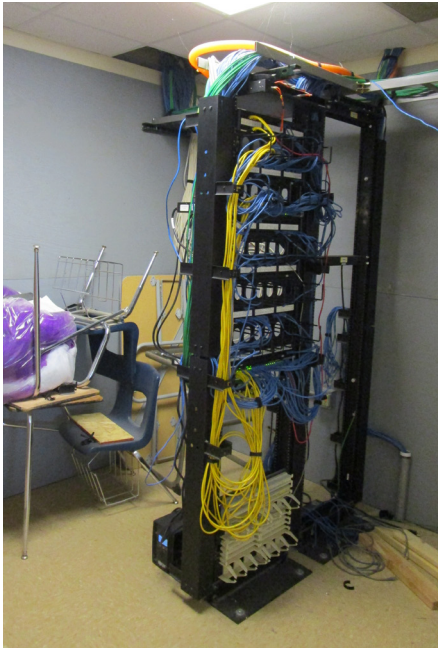
DATA SERVER RACK
