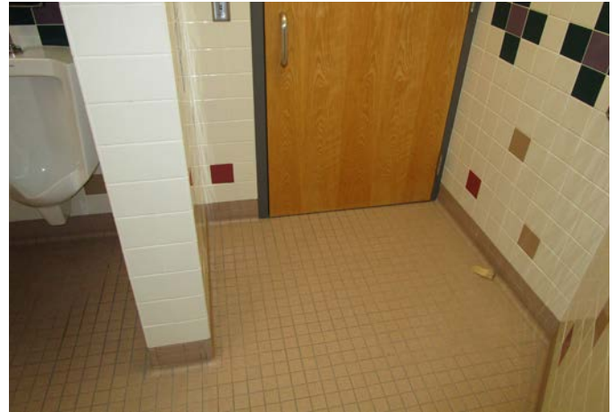
RESTROOM WITHOUT THE REQUIRED PULL SIDE DOOR CLEARANCE
