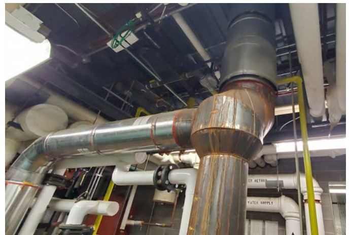
CONDENSATION AT FLUE FOR BOILERS
