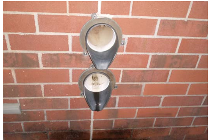
MAIN DRAIN CAUSING DISCOLORATION
