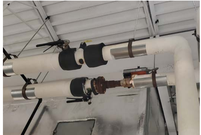
MISSING PIPE INSULATION AT REPAIR LOCATION
