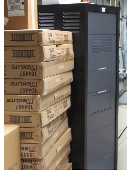
MAIN CLOCK / PAGING CONTROL UNIT
