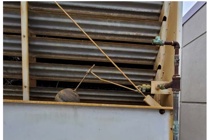
COOLING TOWER FILL VALVE IN NEED OF REPAIR
