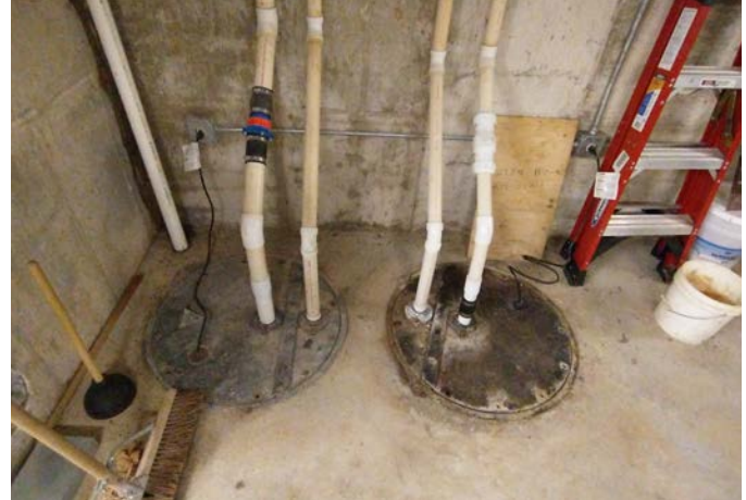
2001 SUMP PUMP/SEWAGE EJECTOR
