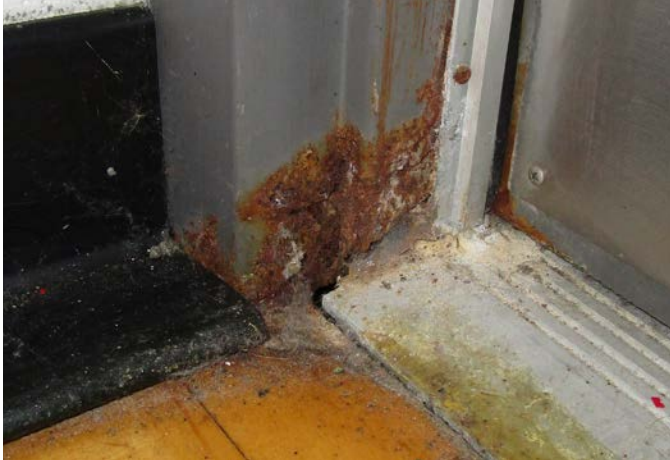
INTERIOR SIDE OF RUSTING DOOR FRAMES
