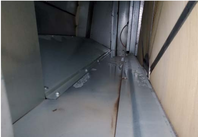
WATER INFILTRATION INTO DOAU CABINET
