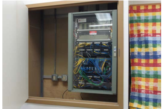
DATA SERVER RACK IN CLASSROOM
