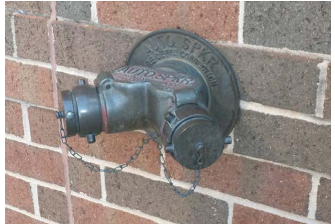
FIRE DEPARTMENT CONNECTION
