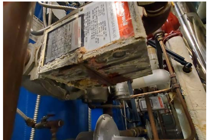
BOILER COMPONENTS IN POOR CONDITION
