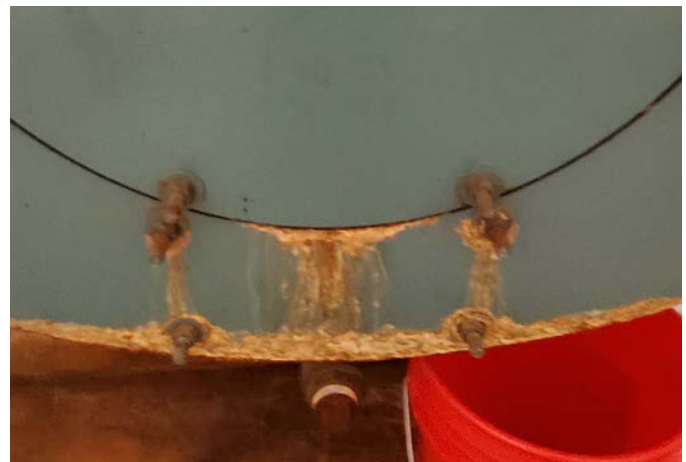
EVIDENCE OF PRIOR BOILER LEAKAGE
