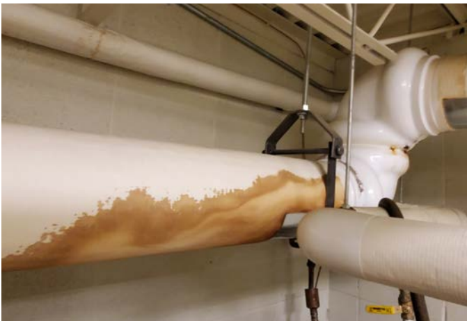
CONDENSATION ON CHILLED WATER PIPING
