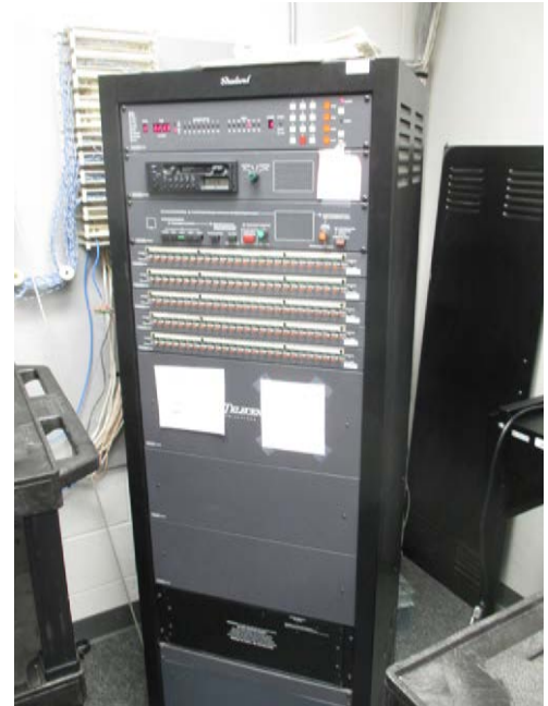
EXISTING CONTROL UNIT
