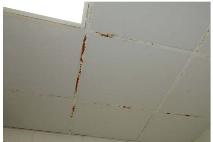
RUSTING CEILING GRID
