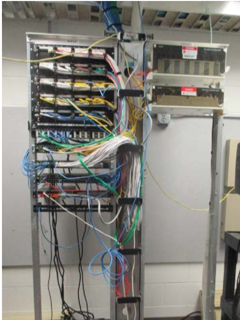
MAIN DISTRIBUTION FRAME
