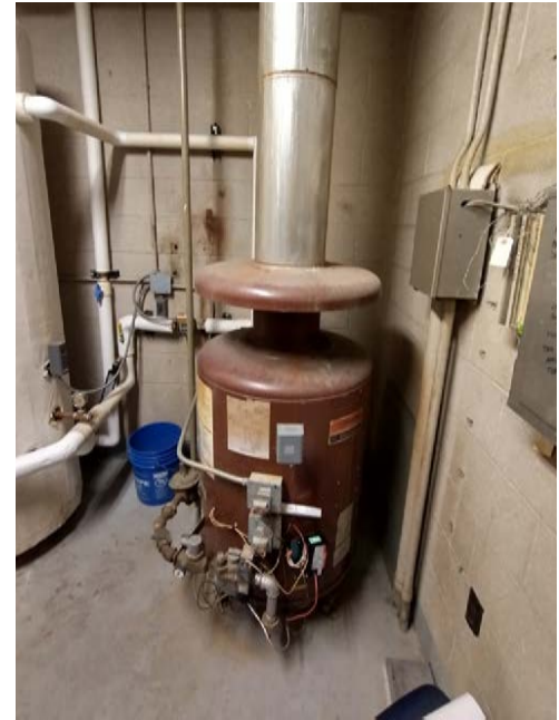
NORTH WATER HEATER
