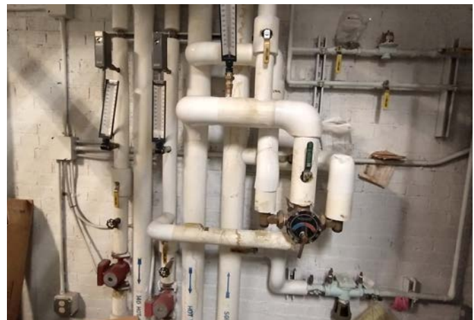
THERMOSTATIC MIXING VALVE AND RECIRCULATION PUMPS
