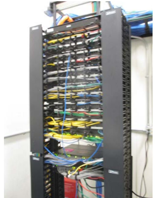
DATA SERVER RACK
