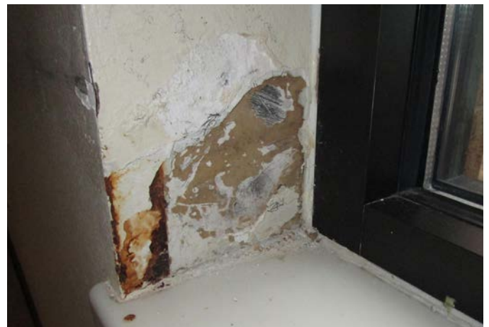
WATER DAMAGE AT DRYWALL WINDOW JAMB
