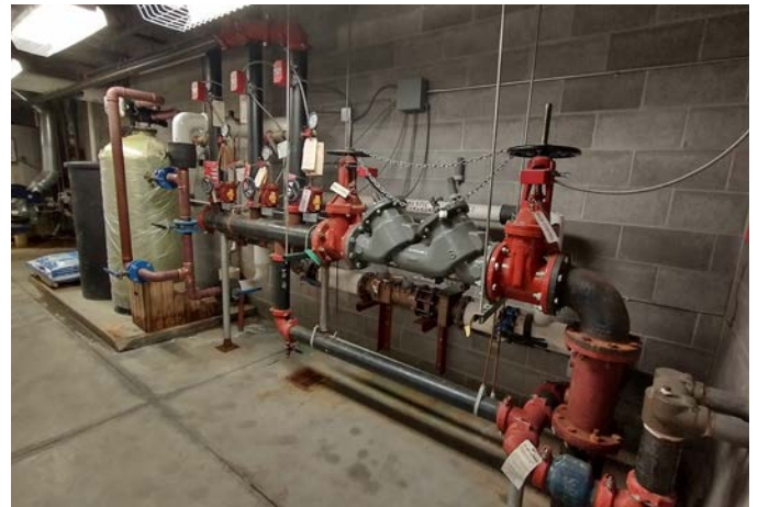
WATER SERVICE ENTRANCE
