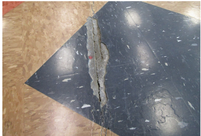
VCT FLOORING CRACKED OVER CONCRETE JOINT
