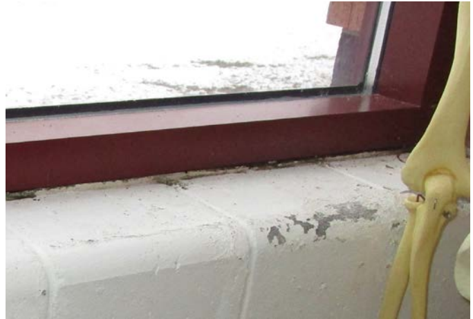
BUBBLED AND MISSING PAINT AT THE INTERIOR SILL
