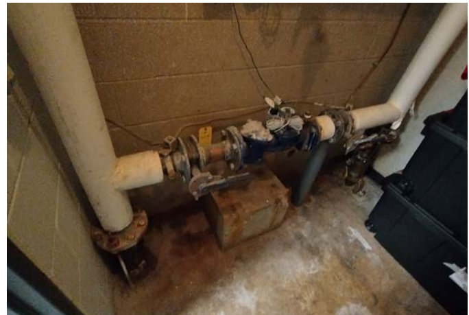
WATER SERVICE ENTRANCE
