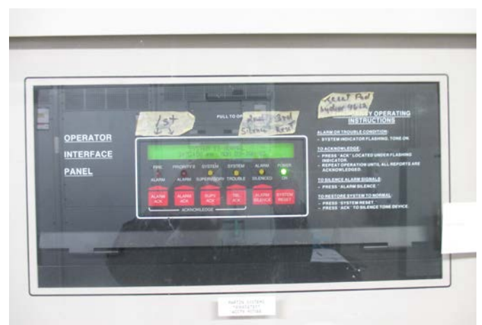
FIRE ALARM ANNUNCIATOR PANEL
