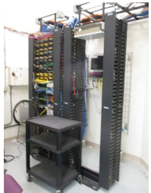
DATA SERVER RACK
