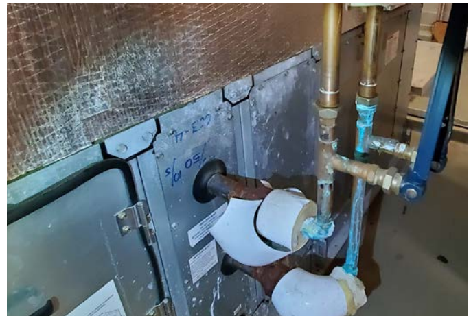
EVIDENCE OF CORROSIVE WATER LEAK
