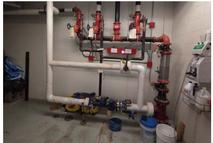
WATER SERVICE ENTRANCE
