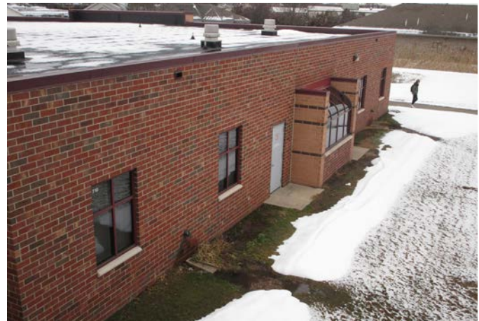
EXIT DOORS WITH NO CONNECTING SIDEWALKS
