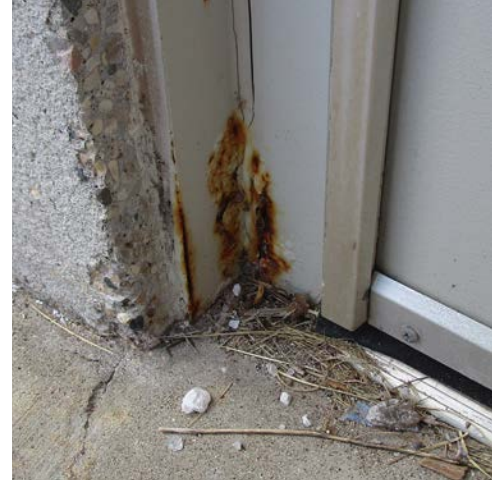
RUST AT EXTERIOR HOLLOW METAL DOOR FRAME
