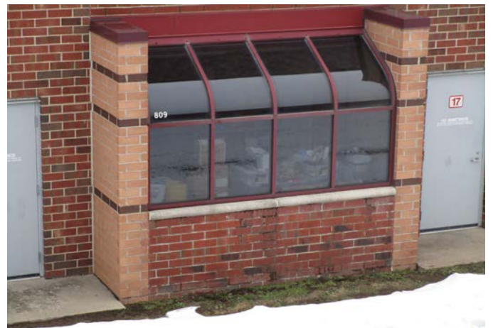
DISCOLORED MORTAR AT SOLARIUM
