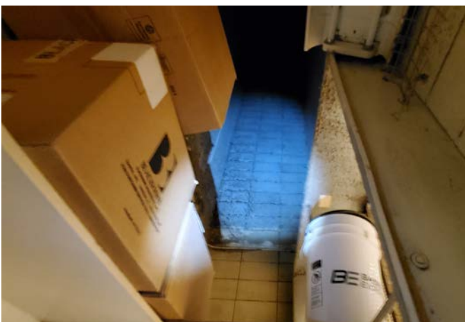
FLAMABLE MATERIALS STORED WITHIN RETURN AIR PLENUM
