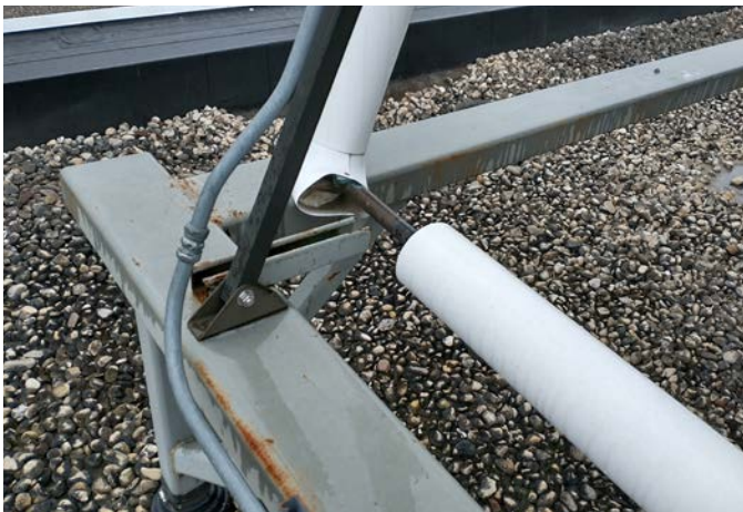
SOLAR ARRAY PIPING
