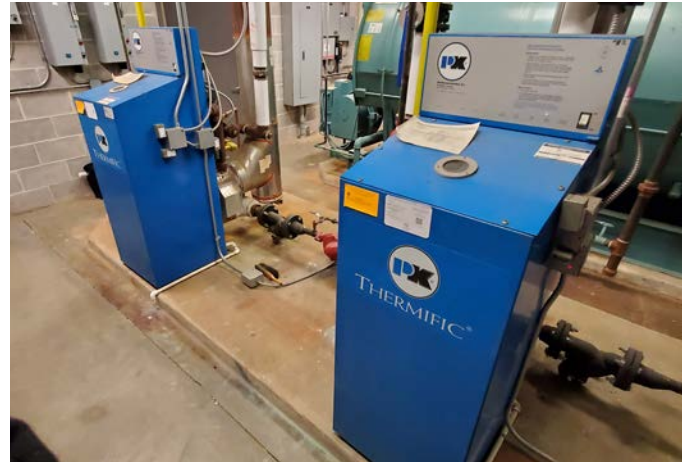
UNDERSIZED SUPPLEMENTARY BOILERS
