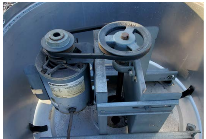
WORN BELT AT ROOF FAN
