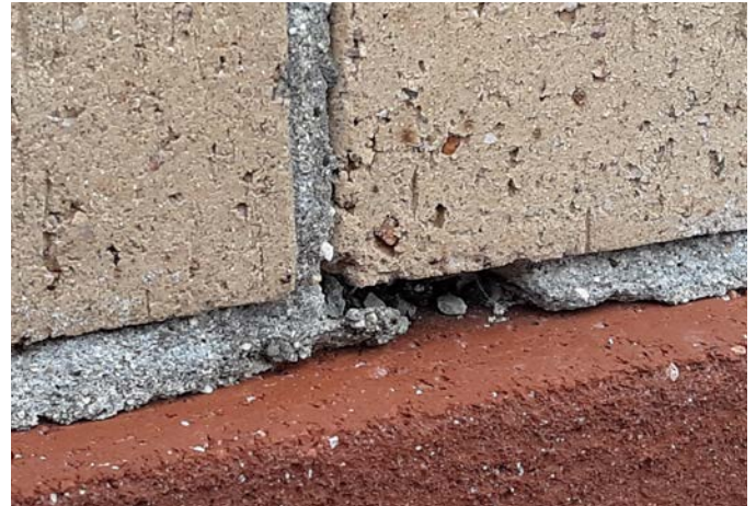
CRACKED MORTAR AT BRICK SETBACK
