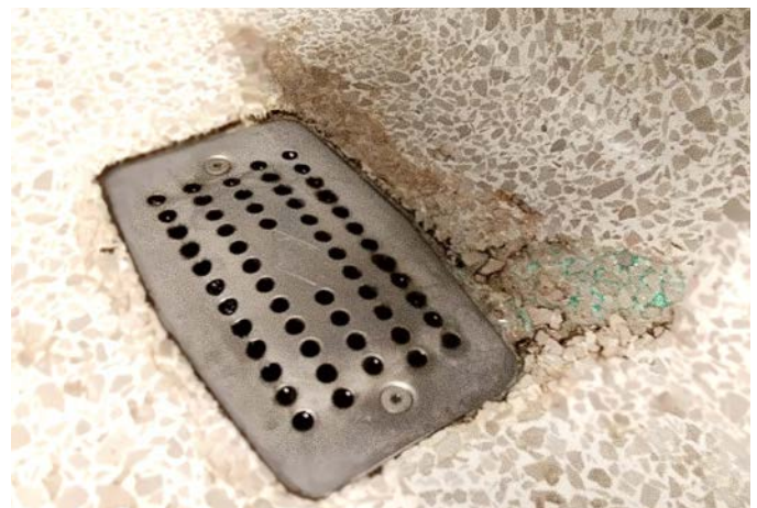
WASH STATION CORROSION
