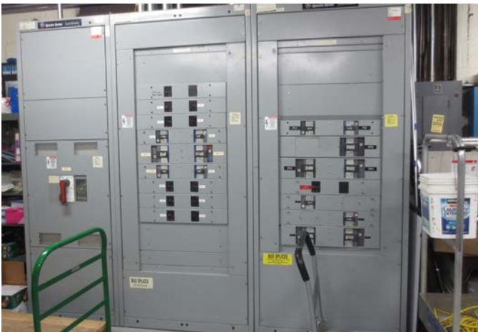
MAIN DISTRIBUTION PANEL
