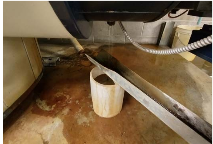
WATER HEATER LEAK
