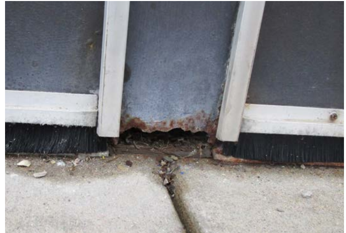
RUSTING HOLLOW METAL DOOR FRAME - EXTERIOR
