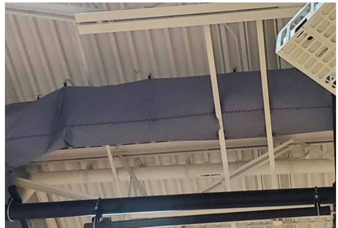
TORN FABRIC DUCT AT GYMNASIUM
