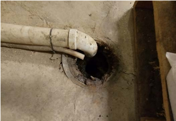
WATER SOFTENER DRAIN
