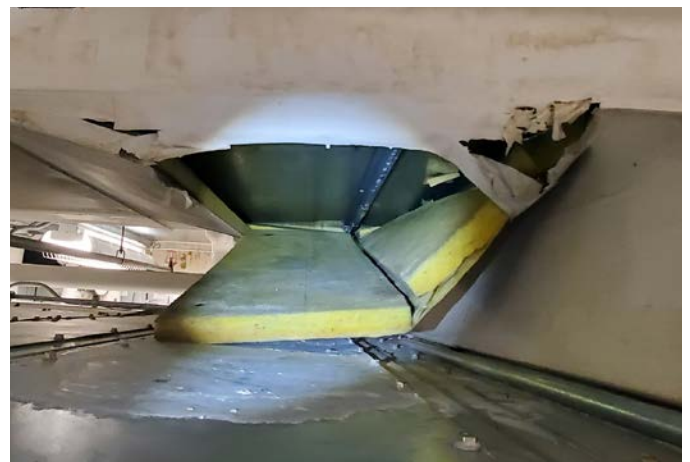
DUCT INSULATION DAMAGE
