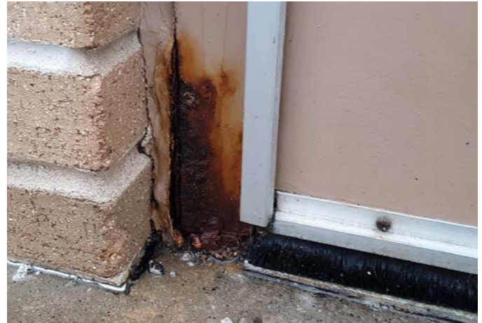
RUST AT HOLLOW METAL DOOR FRAMES
