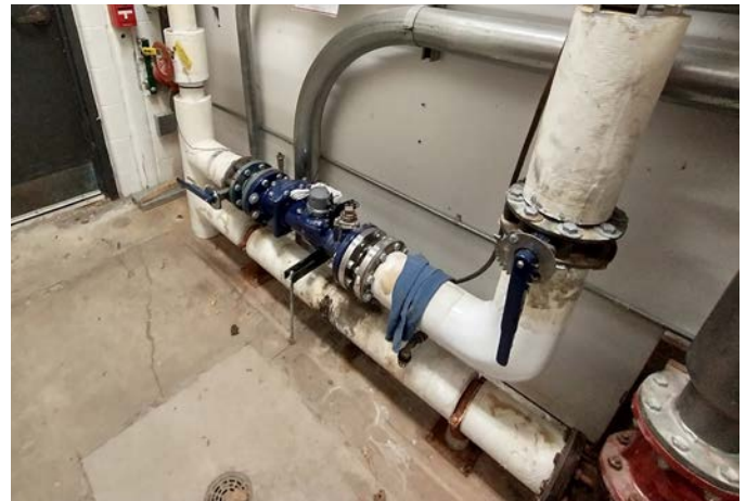
WATER SERVICE ENTRANCE
