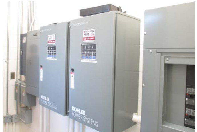
GENERATOR TRANSFER SWITCHES
