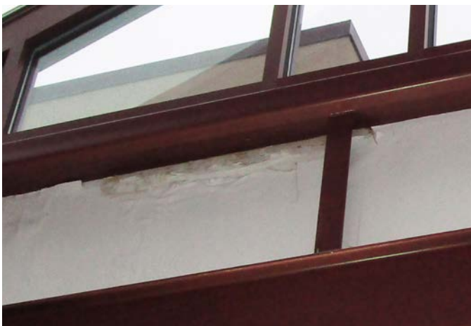
WATER DAMAGE UNDER SKYLIGHT
