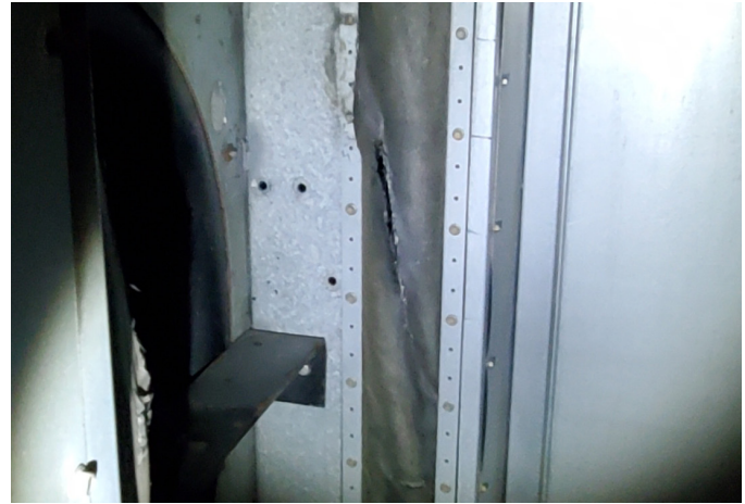
TORN FLEXIBLE CANVAS CONNECTION AT SUPPLY FAN
