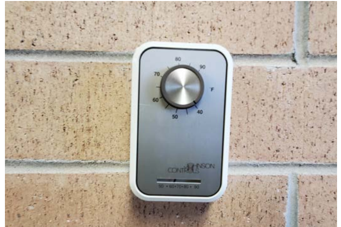
LOW THERMOSTAT SETPOINT LEADS TO FREEZE RISK
