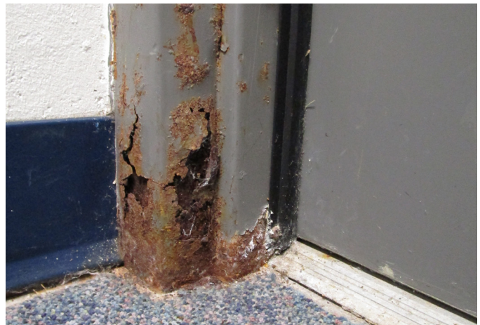
RUSTED HOLLOW METAL INTERIOR DOOR FRAME
