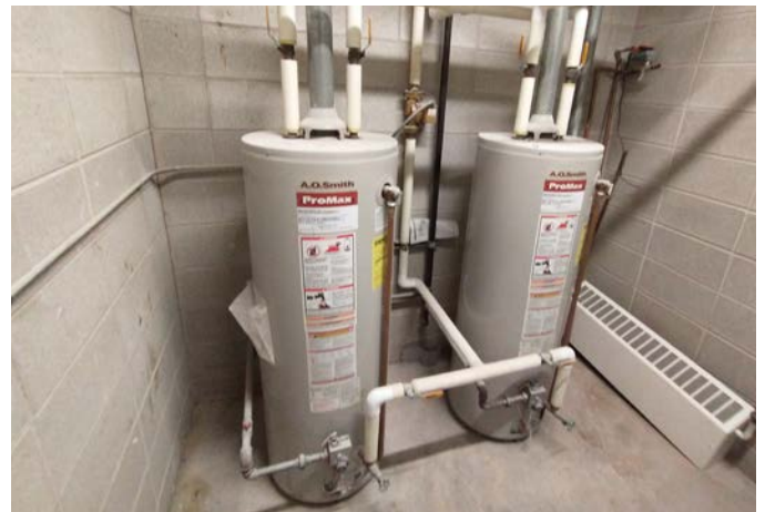
SOUTH WATER HEATERS
