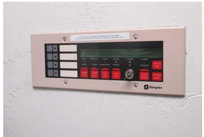
FIRE ALARM ANNUNCIATOR PANEL
