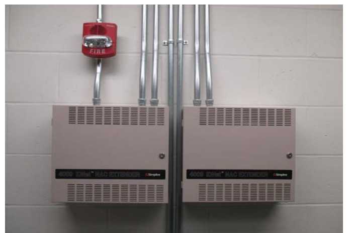
FIRE ALARM EXTENDER PANELS
