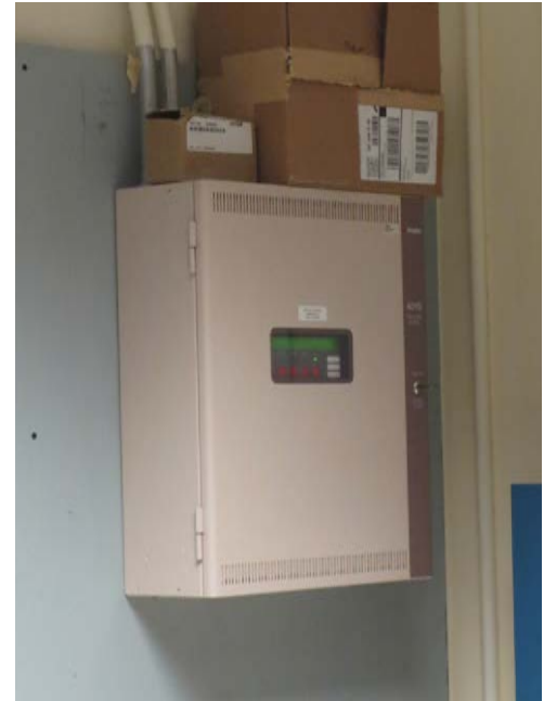
FIRE ALARM CONTROL PANEL
