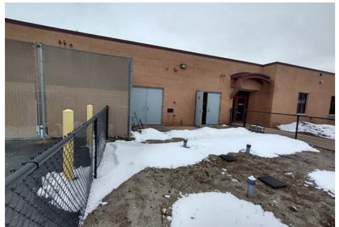
FIRE DEPARTMENT CONNECTION
