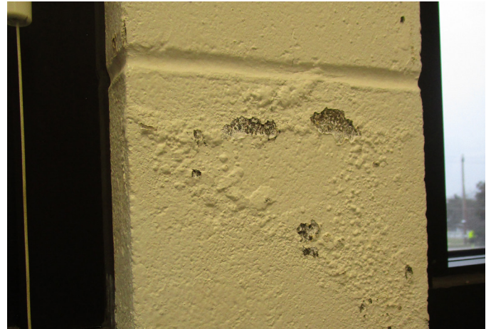
INTERIOR DAMAGE FROM WATER INTRUSION BEHIND THE PAINT
