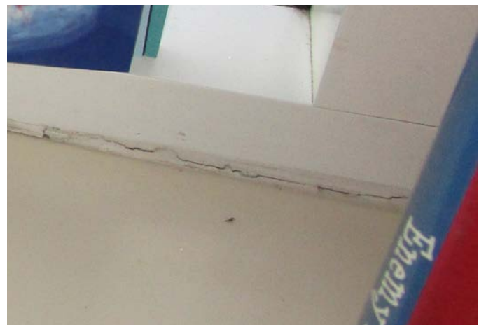
CRACKED CAULKING AT INTERIOR WINDOW FRAMES
