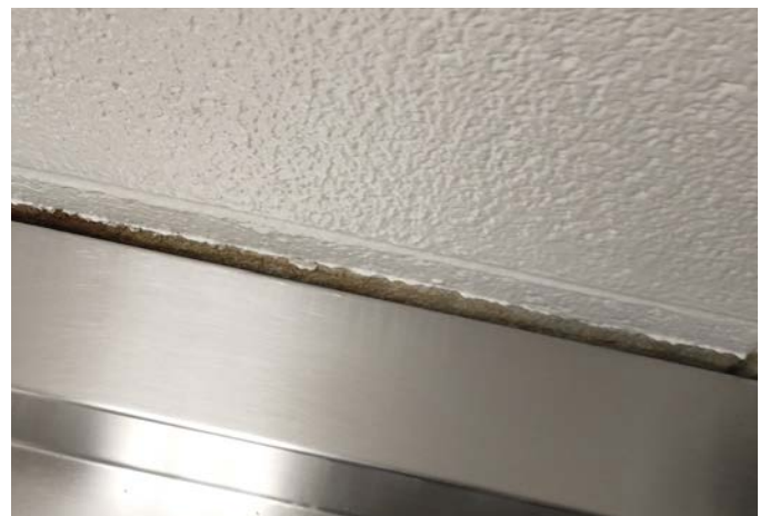
WALL AT CLASSROOM SINK
