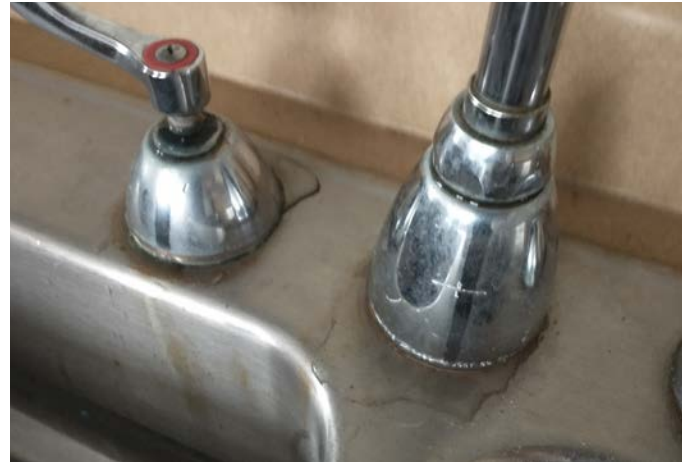
CALCIUM DEPOSIT AT BASE OF FAUCET
