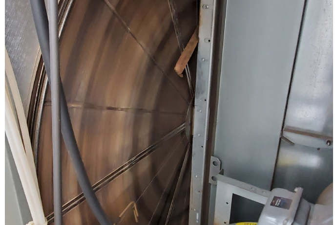
HEAT WHEEL IN METALS AIR HANDLING UNIT
