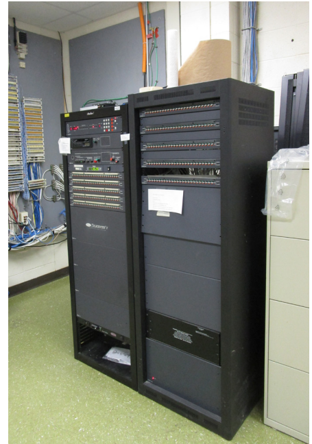
MAIN BELL / PAGING CONTROLS
