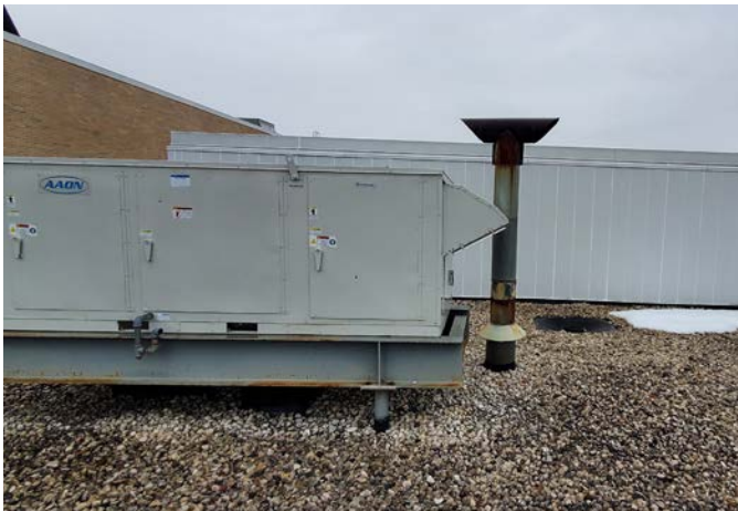
FLUE LOCATED NEAR OUTSIDE AIR INTAKE
