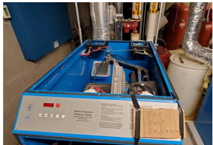
FAILED BOILER B-1
