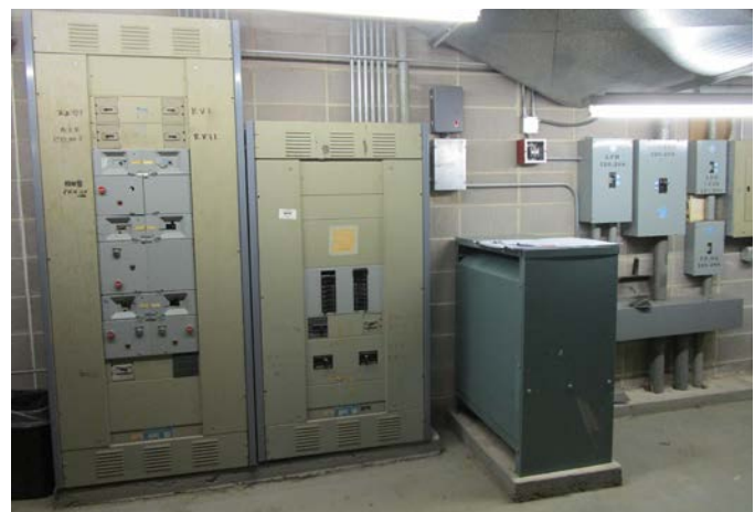
OUTDATED I.T.E DISTRIBUTION PANEL
