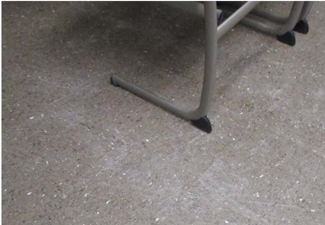
SCRATCHED ON FLOOR FROM PLASTIC FOOT PAD
