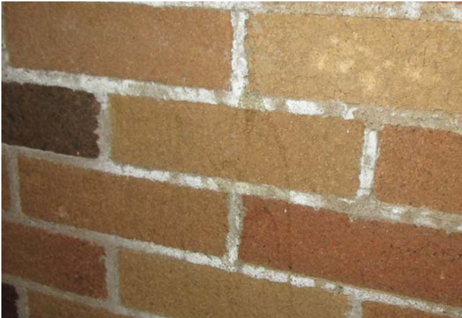
EFFLORESCENCE ON THE INTERIOR OF THE AUDITORIUM
