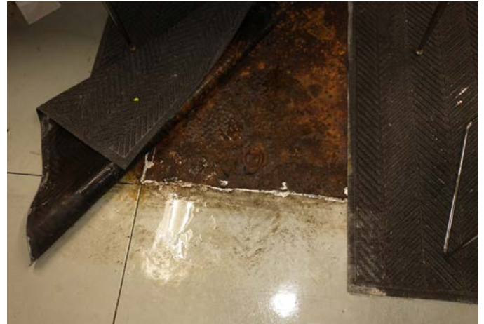
GREASE INTERCEPTOR COVER
