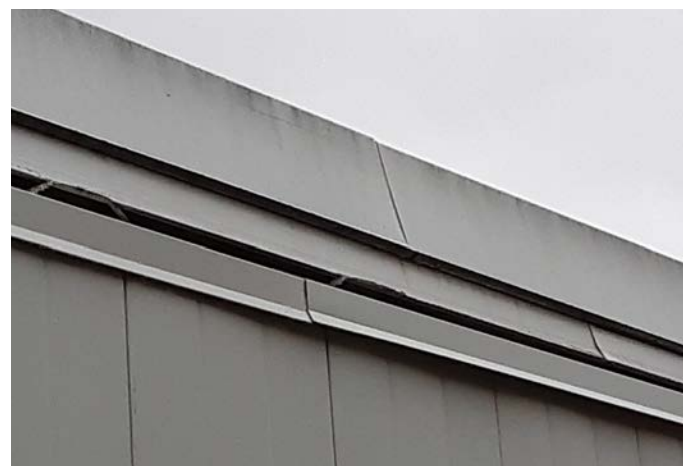
SUCCESSIVE LAYERS OF ROOF COPING TRIM WITH VISIBLE GAPS
