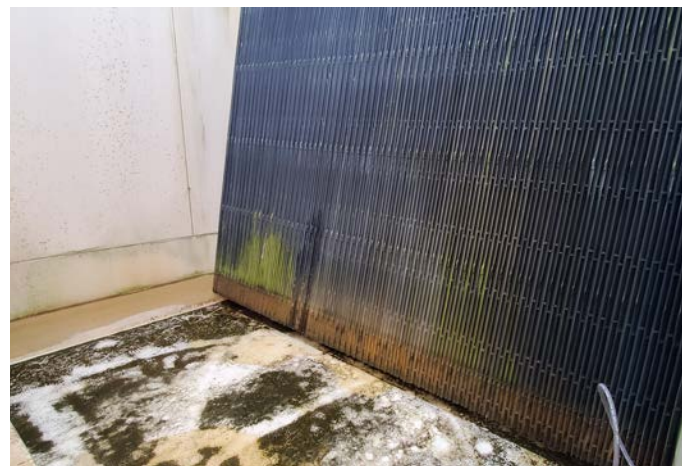
ALGAE GROWTH WITHIN COOLING TOWER MEDIA
