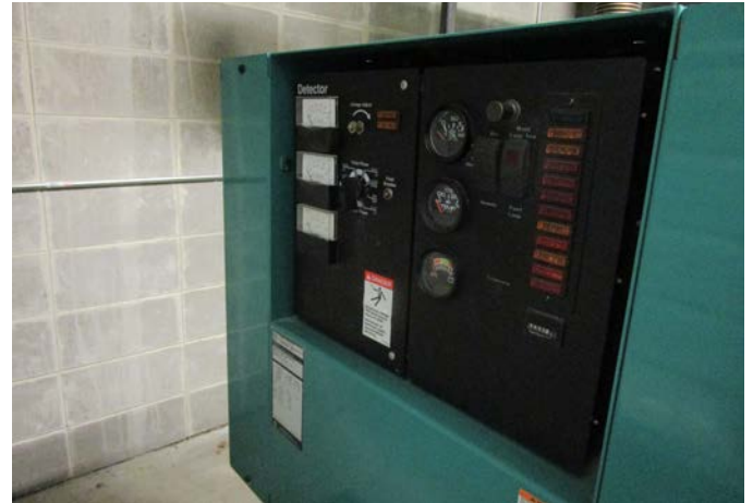
EXISTING GENERATOR CONTROLS
