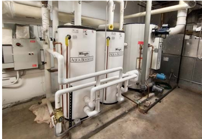
HEAT EXCHANGER AND STORAGE TANKS
