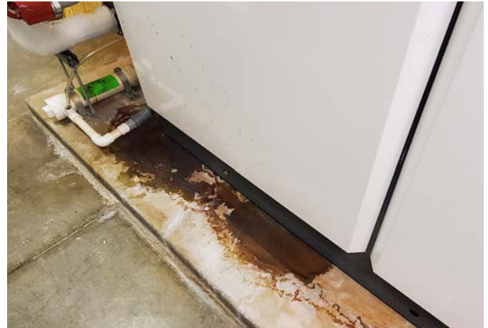
CONDENSATE LEAKING FROM BOILER
