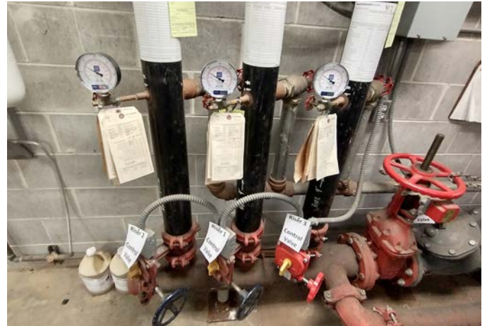
FIRE PROTECTION RISER
