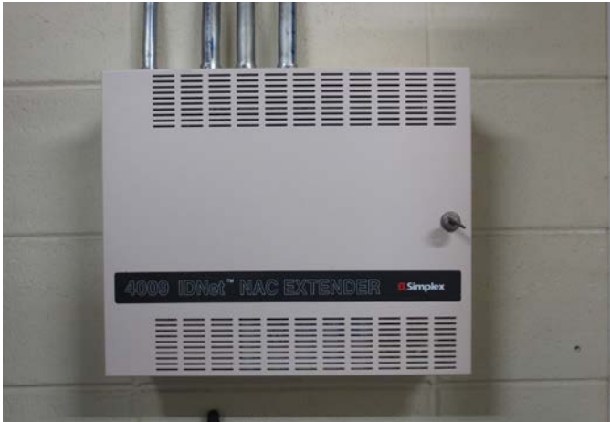
FIRE ALARM EXTENDER PANEL
