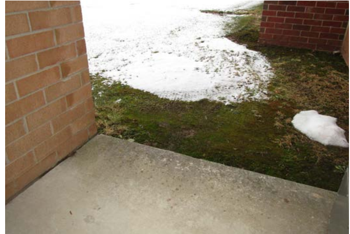
EXIT DOOR WITH NO CONNECTING SIDEWALKS
