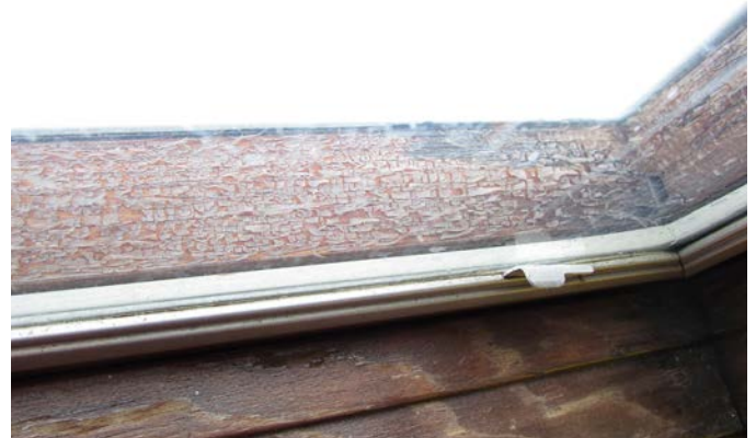
WOOD WINDOW FRAME WITH DELAMINATED POLYURETHANE FINISH IN THE CAVITY BEHIND THE STORM GLASS
