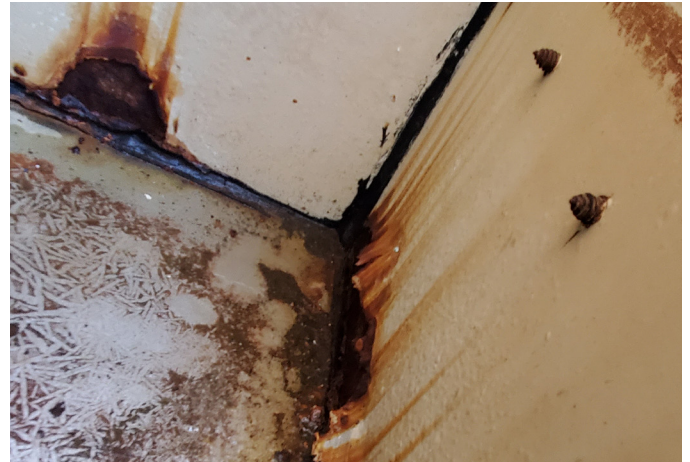
DETERIORATING COOLING TOWER SUMP
