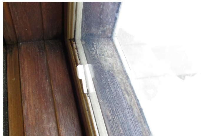
VIEW OF MOLD WITHIN THE CAVITY
