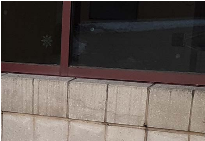
CRACKED MORTAR AT WINDOW SILL
