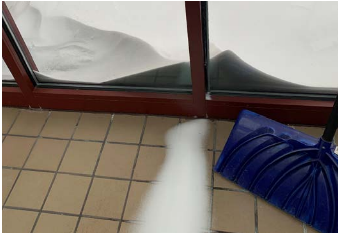
GAP IN GLAZING PANEL
