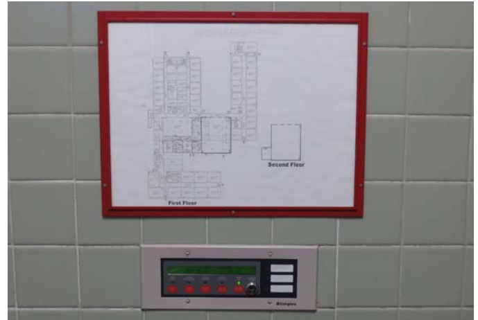
FIRE ALARM ANNUNCIATION PANEL
