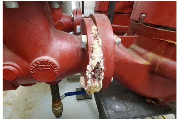
PRIOR LEAK AT HEATING PUMP
