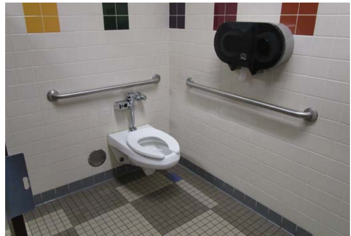
ADA TOILET MISSING VERTICAL GRAB BAR
