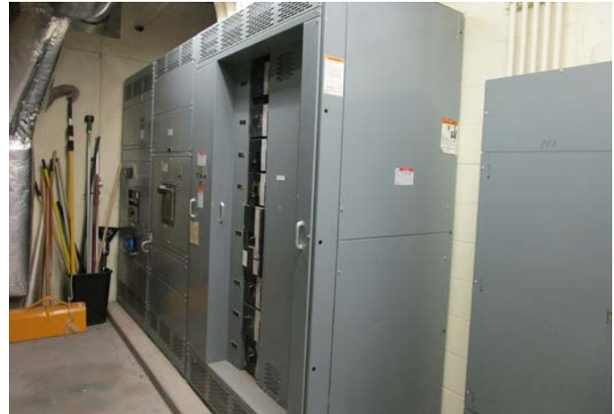
MAIN DISTRIBUTION PANEL
