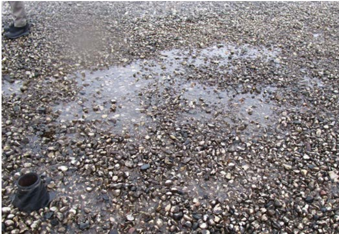
EXCESSIVE PONDING WATER NOT REACHING A DRAIN
