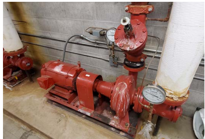
TYPICAL PUMP CONDITION
