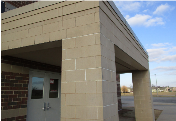
EFFLORESCENCE IN BLOCK COLUMN
