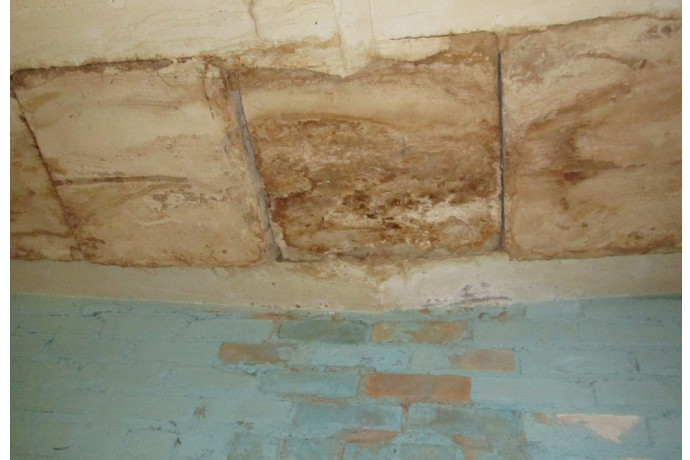
PROLONGED WATER INFILTRATION ON THE CEILING
