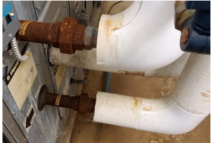
PIPE CORROSION DUE TO LACK OF INSULATION
