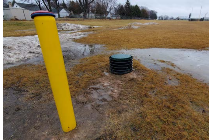
GEOTHERMAL FIELD VAULT ACCESS MANHOLE
