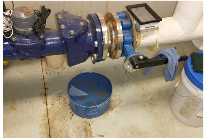
WATER METER LEAK
