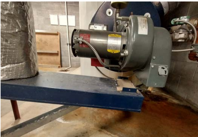
COMBUSTION AIR DUCTWORK DISCONNECTED
