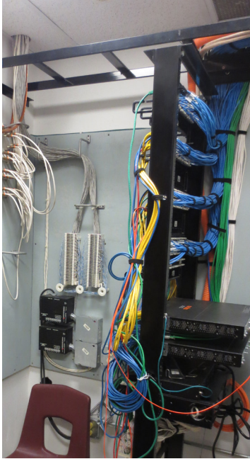
DATA SERVER RACK
