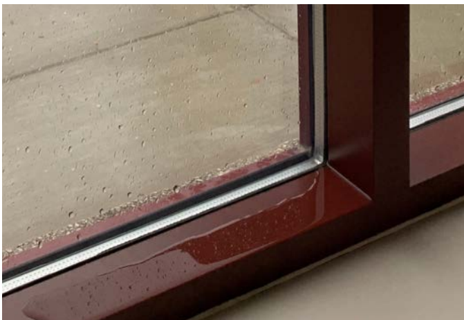
WATER LEAKING FROM GLAZING PANEL GASKETS
