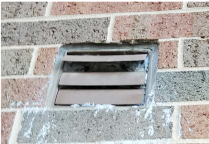
DRYER EXHAUST REQUIRES CLEANING
