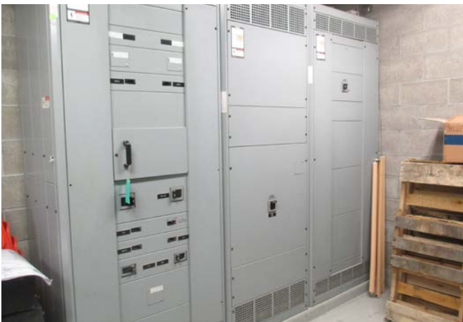
MAIN DISTRIBUTION PANEL
