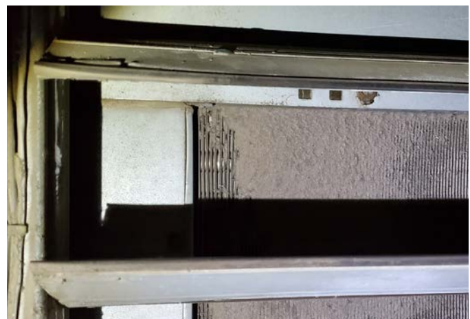
DIRTY AHU COIL FROM LEAKING FILTER RACK
