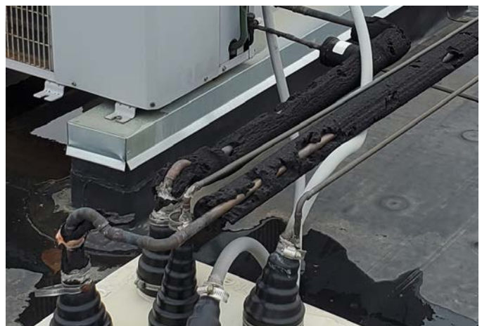
DETERIORATED PIPE INSULATION ON ROOF
