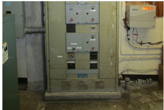
OUTDATED I.T.E DISTRIBUTION PANEL
