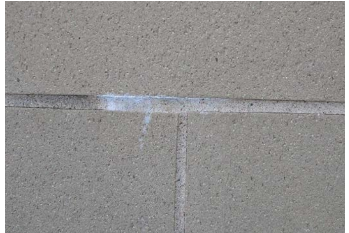
CLOSE UP OF EFFLORESCENCE
