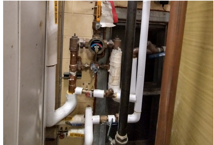
THERMOSTATIC MIXING VALVE AND RECIRCULATION PUMPS
