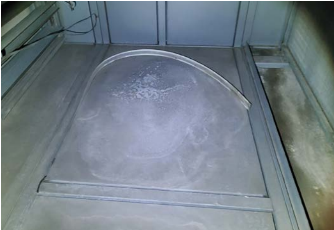
DETERIORATING SEAL AT AIR HANDLING UNIT CASING
