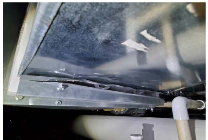
TYPICAL DUCT LEAKAGE AT SEAMS
