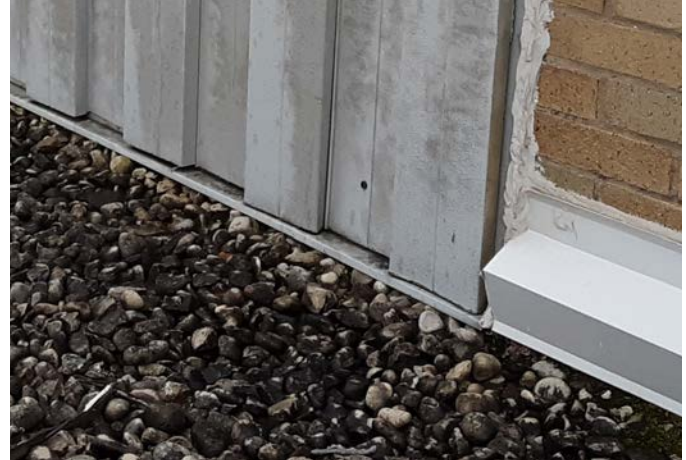
METAL WALL PANELS TOO CLOSE TO THE ROOF
