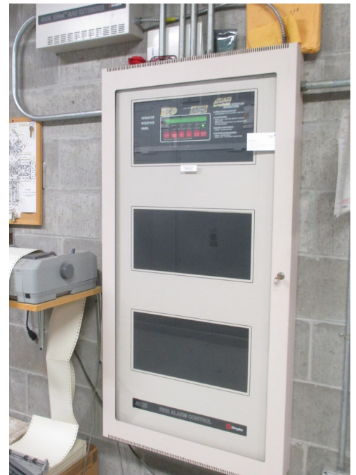
FIRE ALARM CONTROL PANEL
