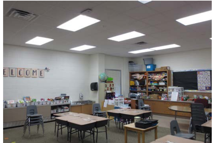
TYPICAL CLASSROOM LIGHTING
