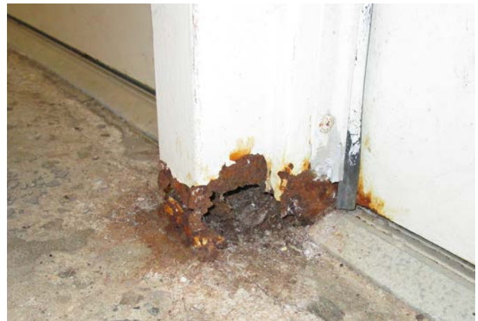
RUSTING HOLLOW METAL DOOR FRAME – INTERIOR
