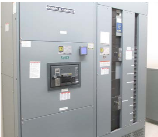
MAIN DISTRIBUTION PANEL
