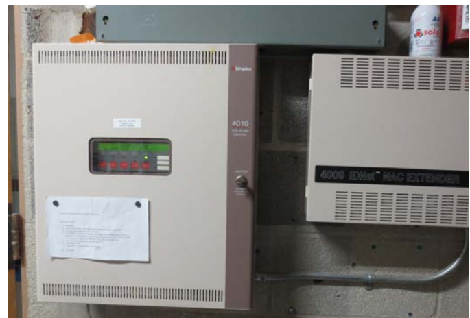
FIRE ALARM CONTROL PANEL
