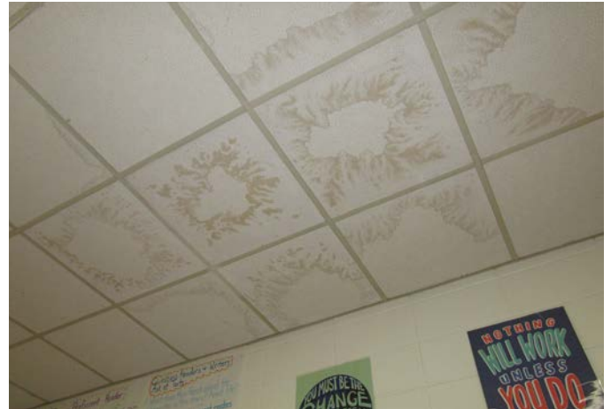
ROOF LEAK STAINS ON YELLOWING CEILING TILES
