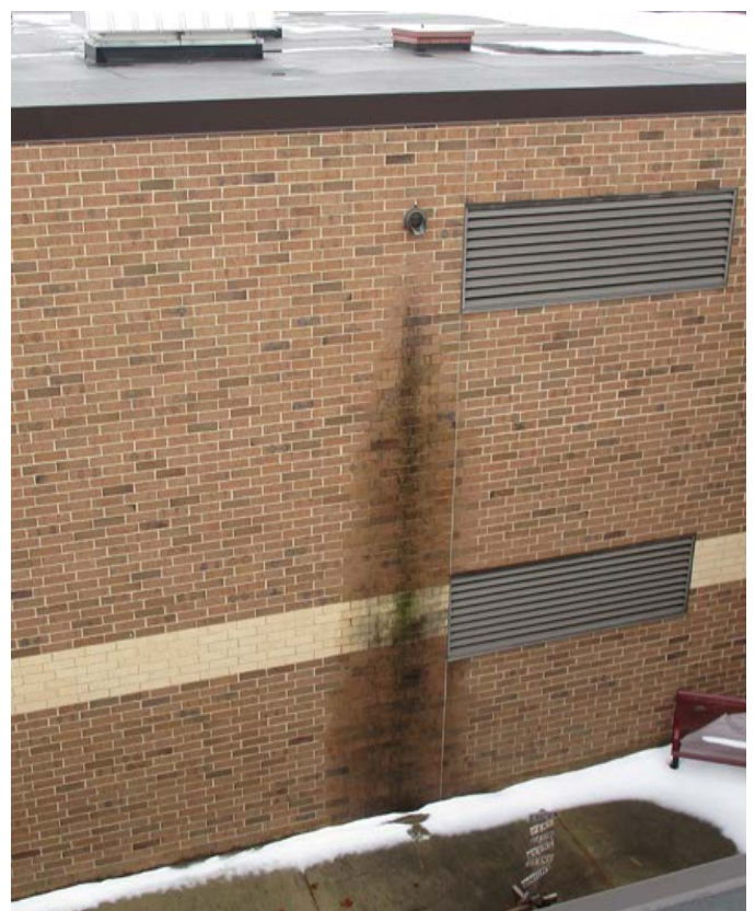
ACTIVE RELIEF ROOF DRAINS STAINING EXTERIOR WALLS
