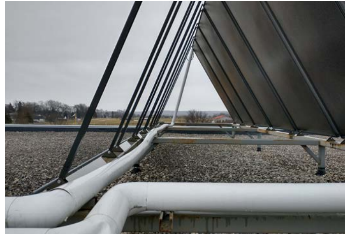
SOLAR ARRAY PIPE SUPPORT
