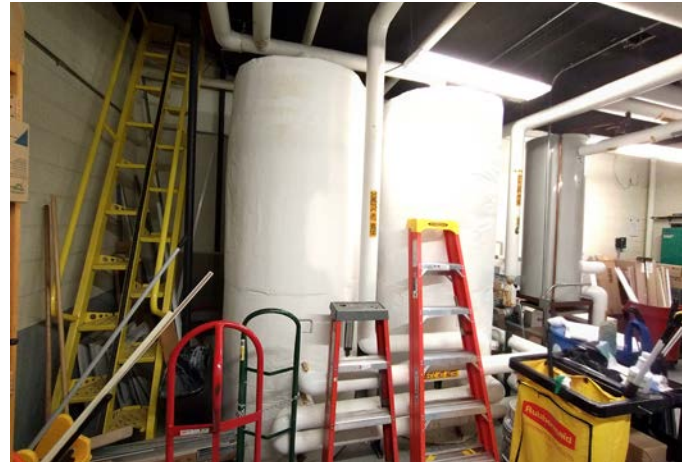
SOLAR THERMAL STORAGE TANKS
