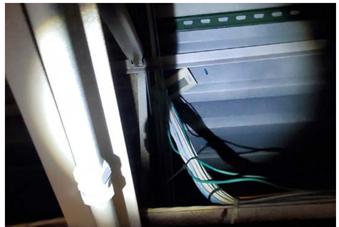
THERMOSTAT INSTALLED ABOVE FINISHED CEILING
