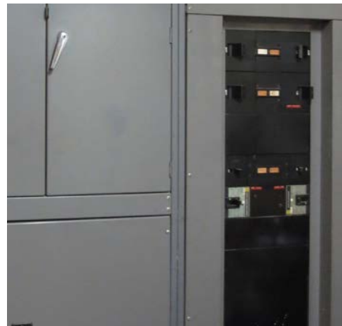
ORIGINAL MAIN DISTRIBUTION PANEL
