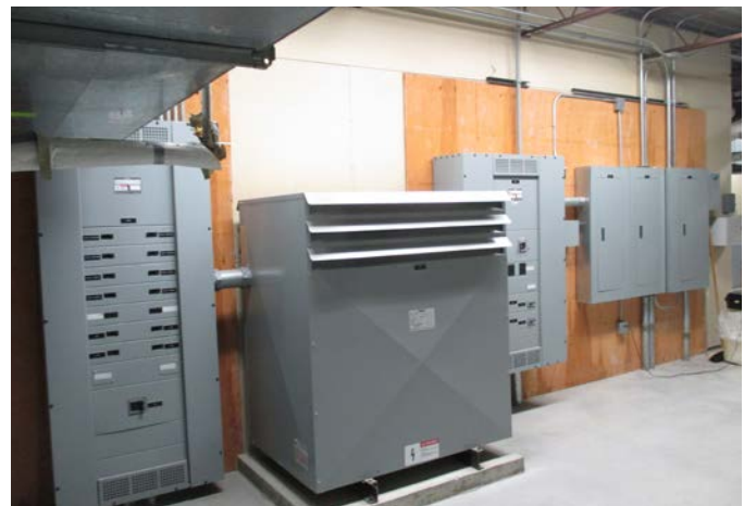
SUB DISTRIBUTION PANELS
