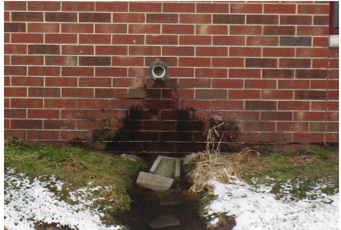
EROSION UNDER ROOF DRAIN OUTLET
