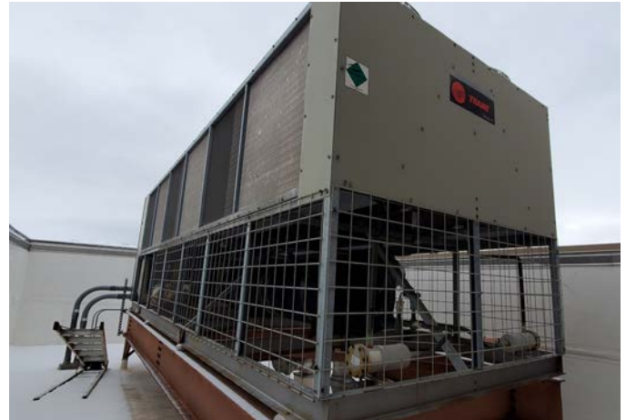
AIR-COOLED CHILLER HAS EXPERIENCED MULTIPLE FAILURES
