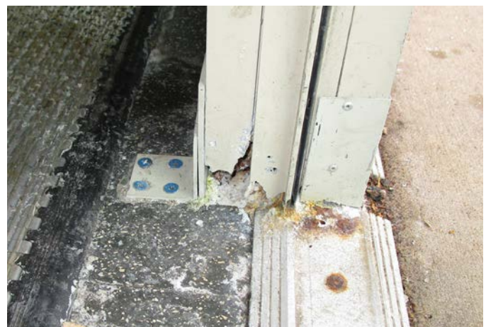
ATTEMPTS HAVE BEEN MADE TO FIX THE FRAMES
