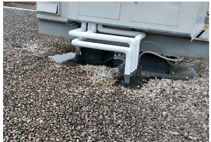
WATER PONDING NEAR ROOF DRAIN
