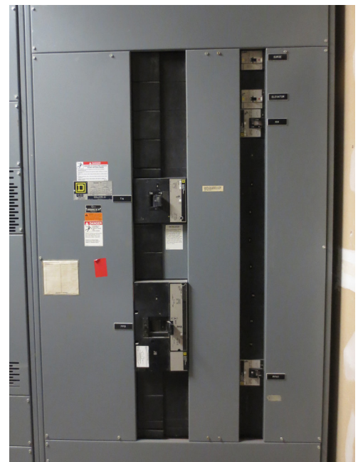
MAIN DISTRIBUTION PANEL
