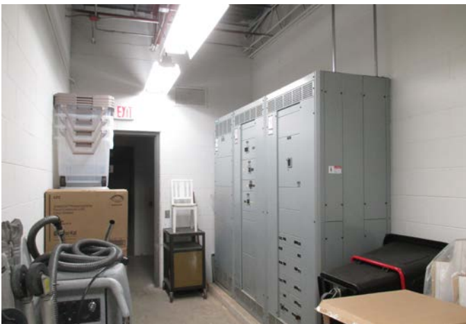
MAIN DISTRIBUTION PANEL
