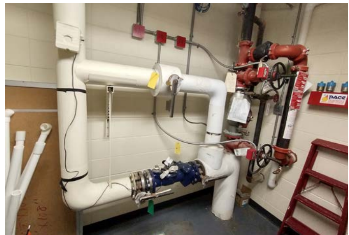
WATER SERVICE ENTRANCE
