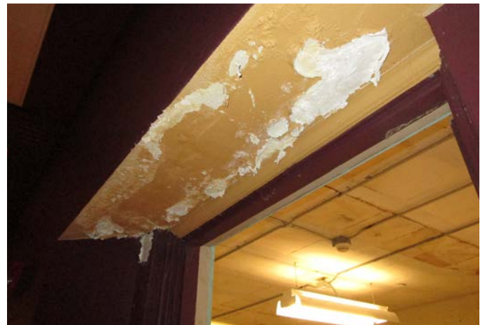
WATER INFILTRATION BEHIND THE PAINT
