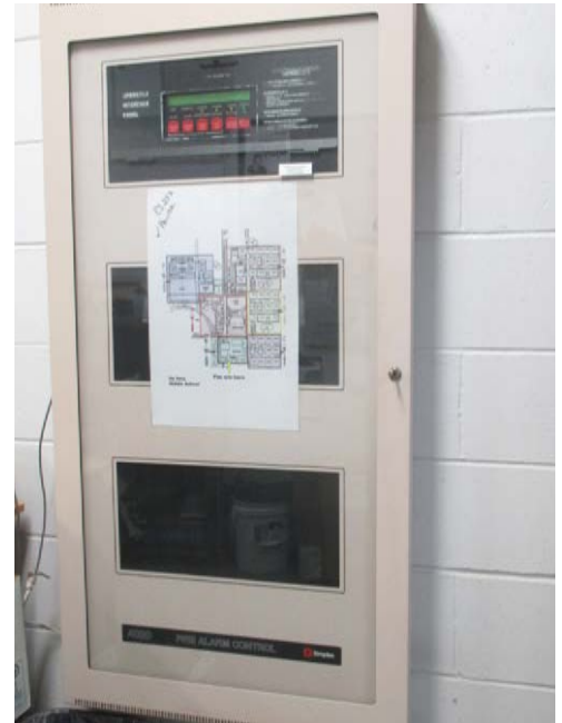
FIRE ALARM CONTROL PANEL
