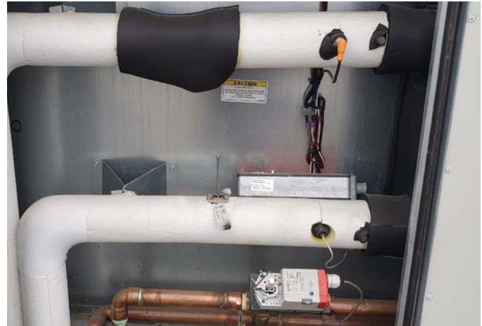
DOAU UNIT WITH GEOTHERMAL VALVE LOCKED OPEN
