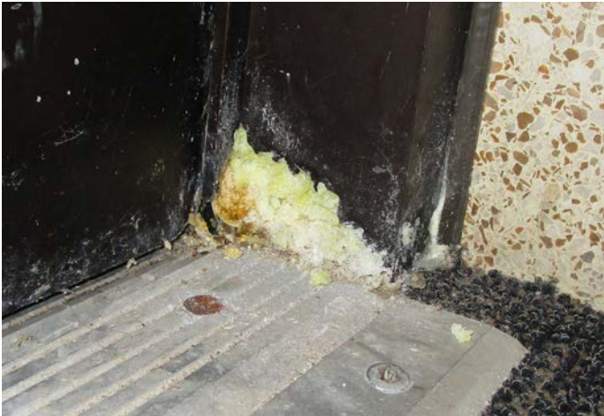
ALUMINUM DOOR FRAME DETERIORATION – INTERIOR
