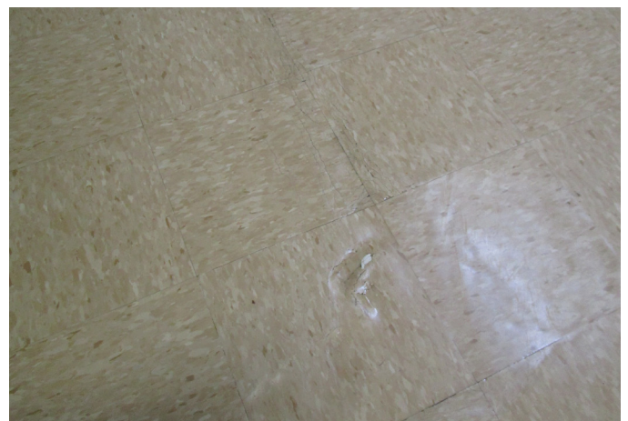
VCT DEPRESSED INTO FLOOR JOINT IN SLAB
