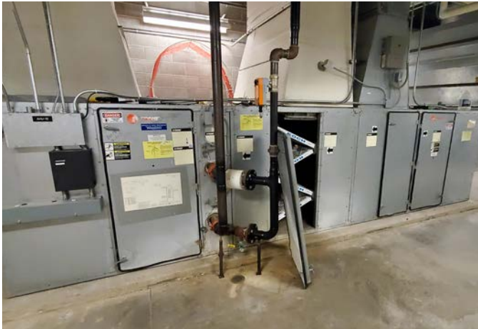
AHU-15 DOOR IS REMOVED
