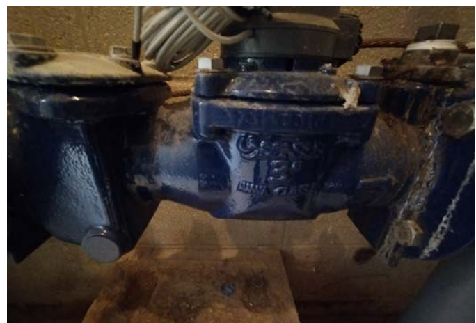
WATER METER LEAK
