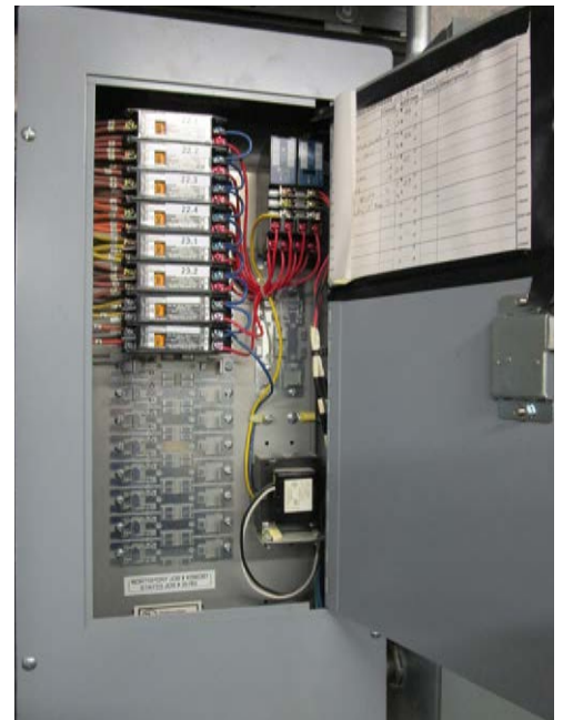
LIGHTING CONTROL SUB-PANEL
