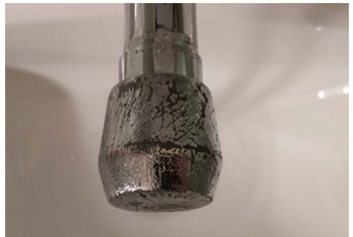
LAVATORY FAUCET DELAMINATING
