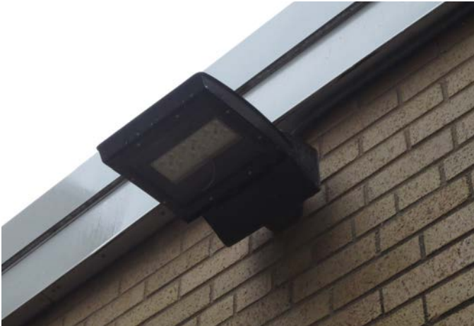
EXTERIOR LIGHTING FIXTURE
