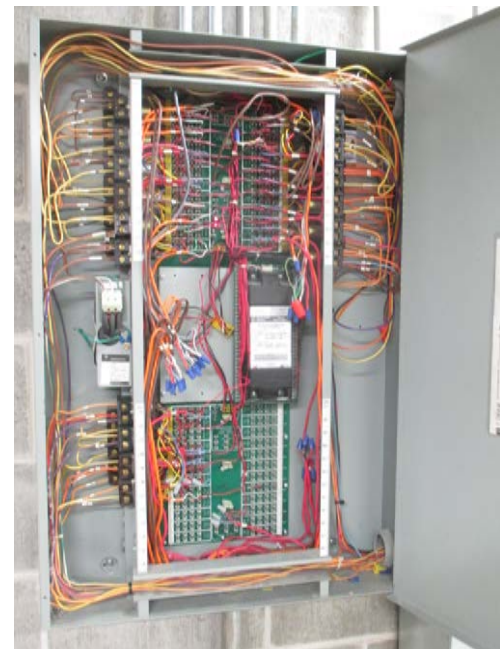
LIGHTING CONTROL PANEL
