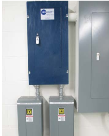
LIGHTING CONTROL PANEL
