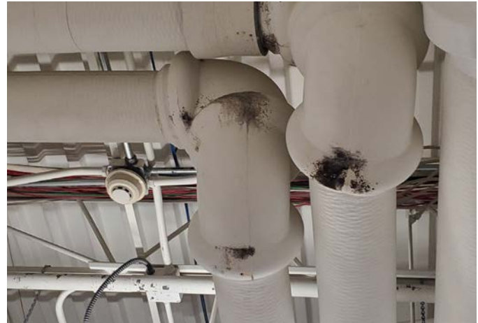
TYPICAL MOLD ON CHILLED WATER INSULATION
