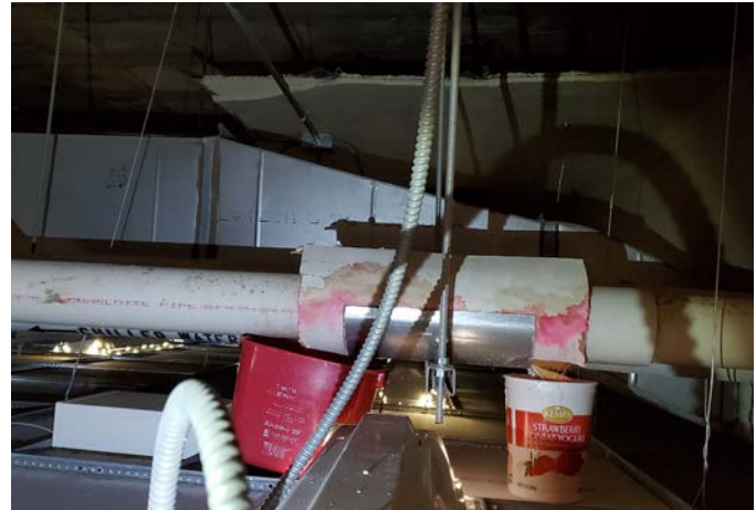
CHILLED WATER PIPE LEAK
