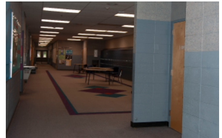
IMS 100/200 Building: Lack of natural light
