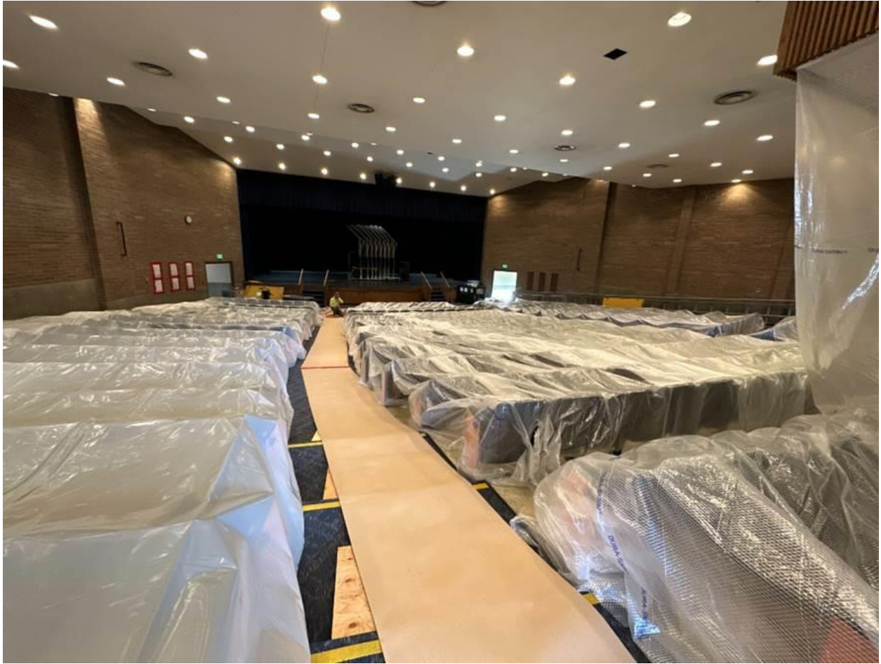
The PAC Auditorium seating and flooring are covered to protect it during seismic upgrade work
