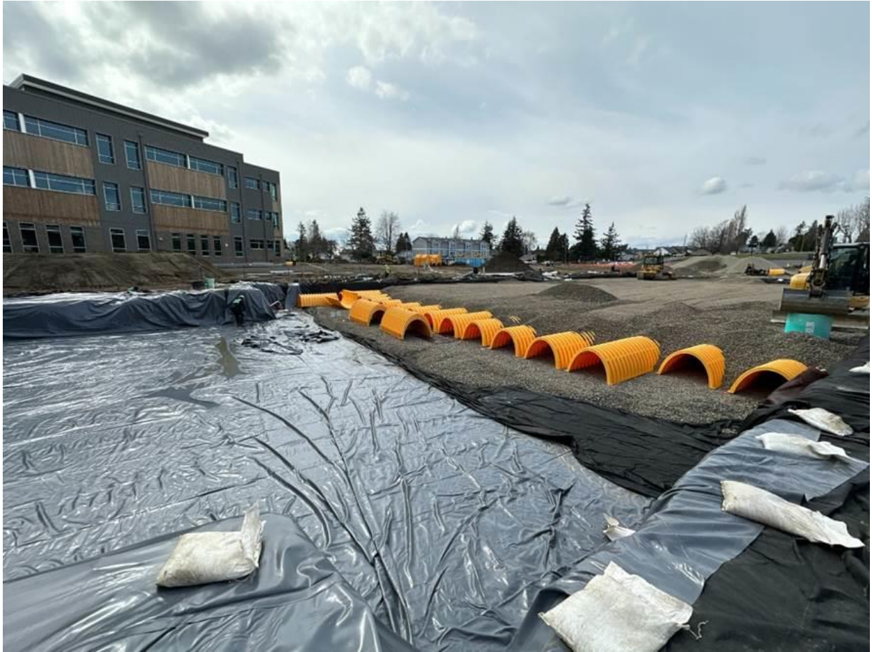
The underground rainwater detention system under the new family drop-off area
