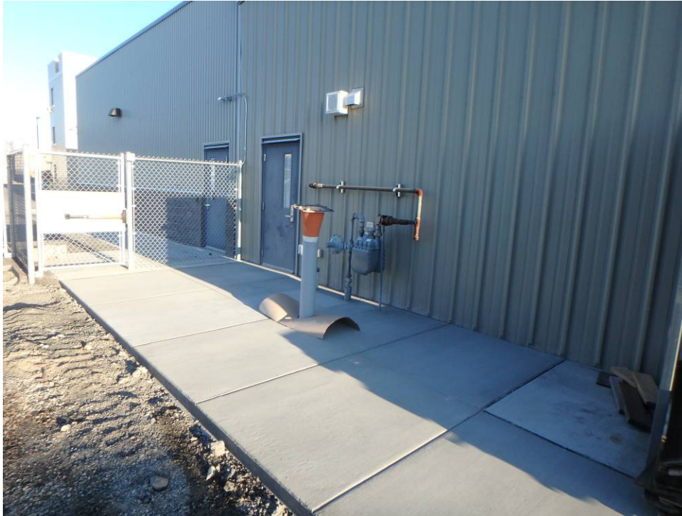
Tri Tech east gas meter slab
