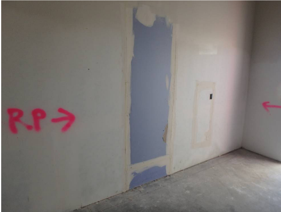
Wallboard repair at the manifold to be relocated in the Kennel Room - lower
