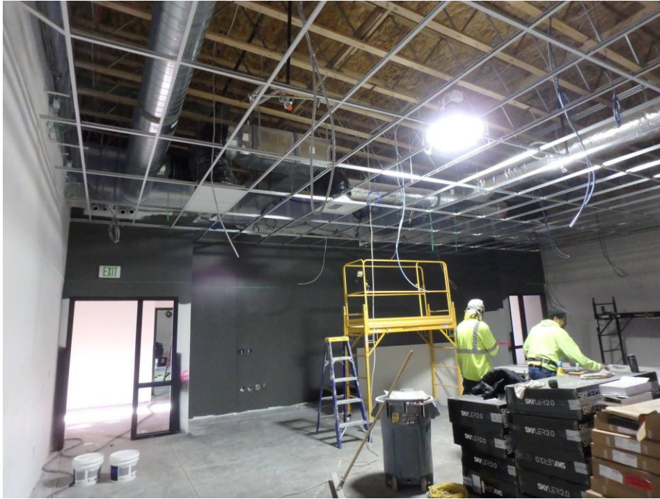
Looking southwest across the north classroom at the ceiling grid and accent wall
