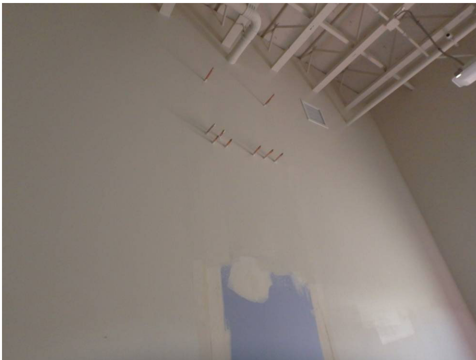
Wallboard repair at the manifold to be relocated in the Kennel Room
