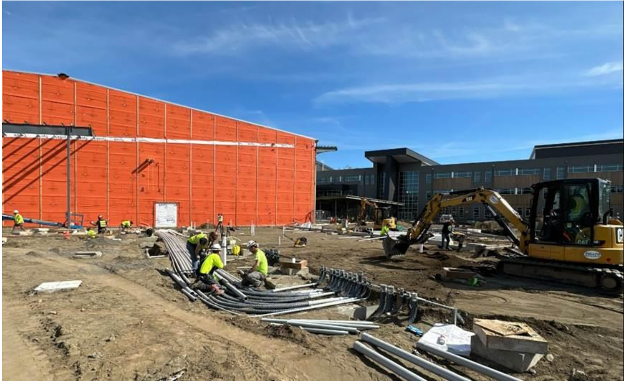
Underground electrical piping in the CTE Wing subgrade (the land underneath the building)
