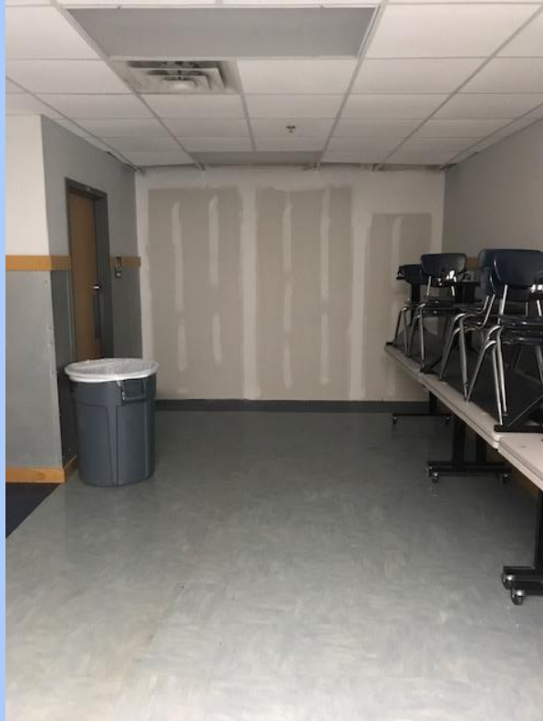
Temporary wall to block off main building from CTE building for the purpose of construction
