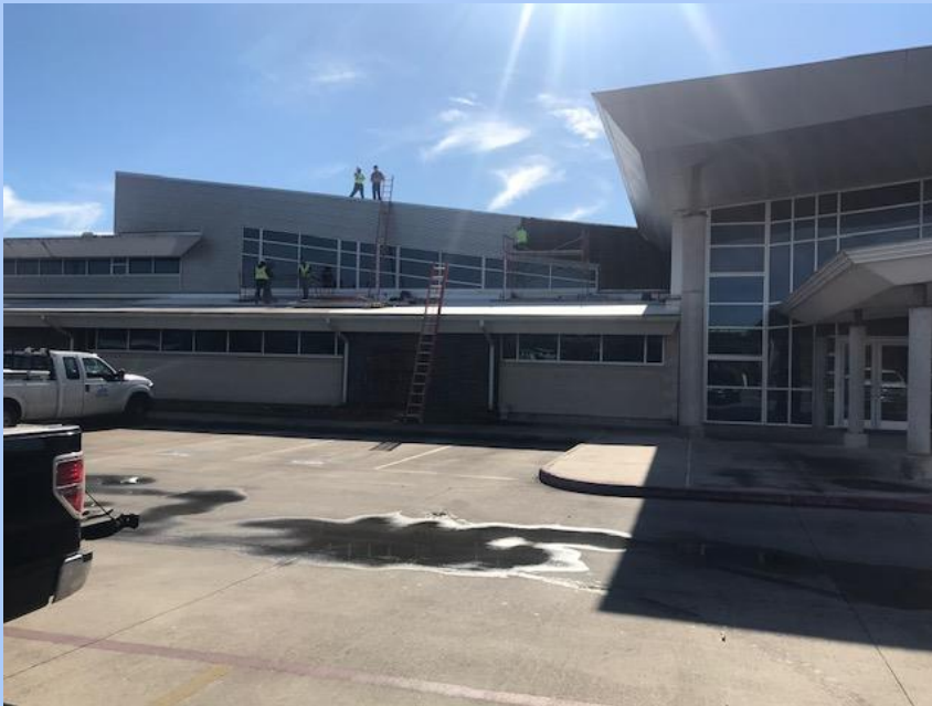
Leak repair work at the front of the high school (remediation from high school remodel)
