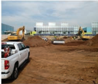
Stormwater Detention System
