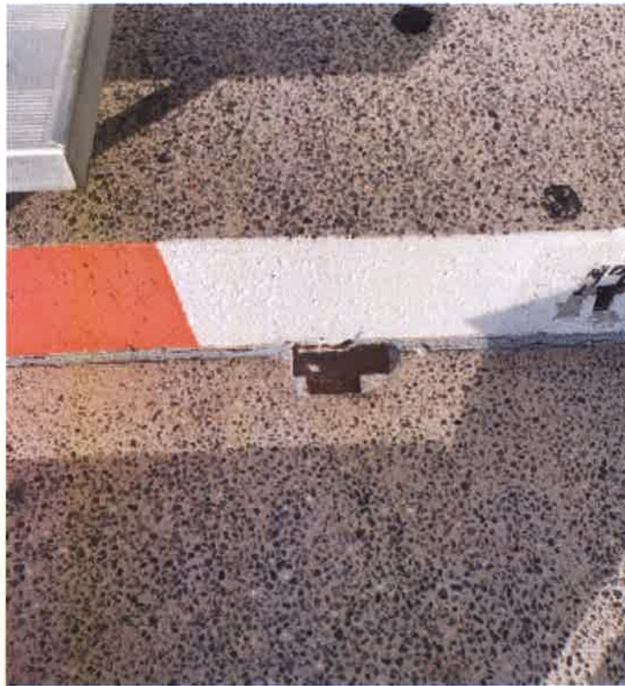
Photo 43: Protruding Rusted Diaphragm Tie Plate
