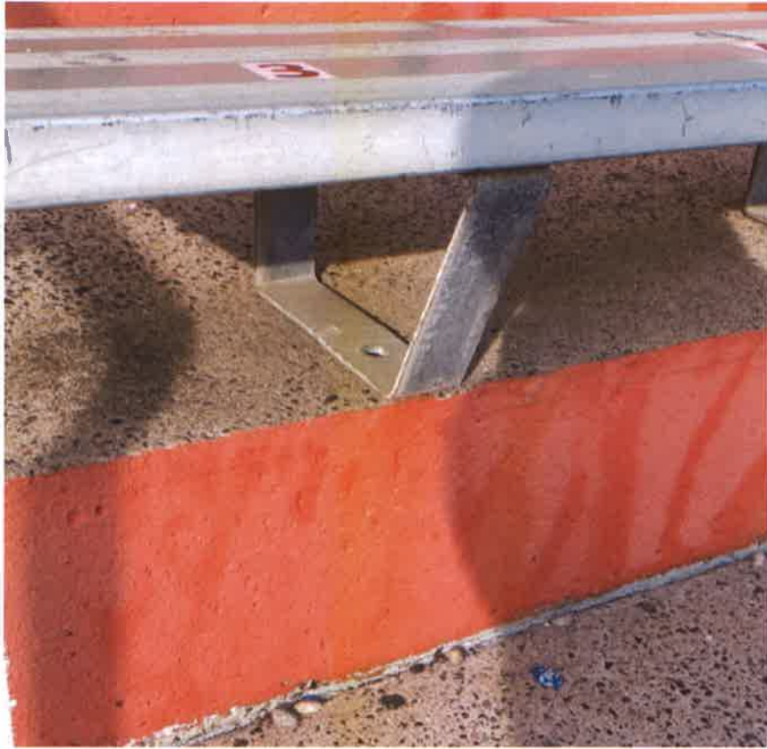
Photo 50: Missing Anchor for Seating Arrangement
