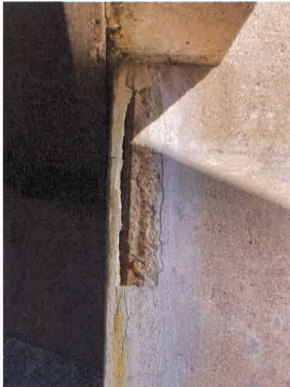
Photo 32: Exposed Rusted Rebar After Spalling of Repair on Ramp Sidewall
