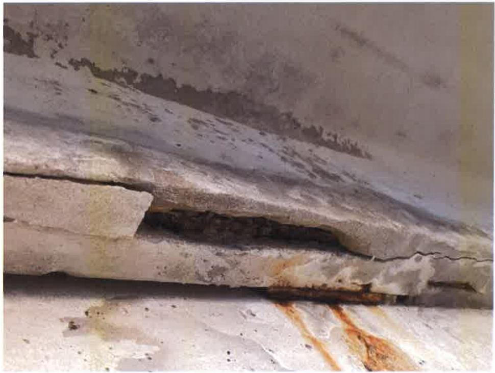
Photo 31: Rusted Diaphragm Tie Plate Causing Deterioration of Surrounding Concrete
