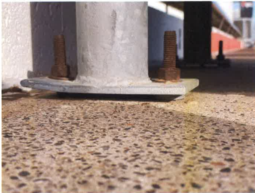
Photo 47: Rusted Anchor Bolts Sitting on Multiple Washers
