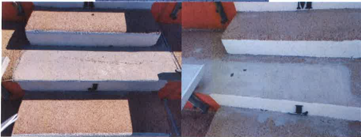
Photo 81: Crack on Repaired Steps on Southern Side
