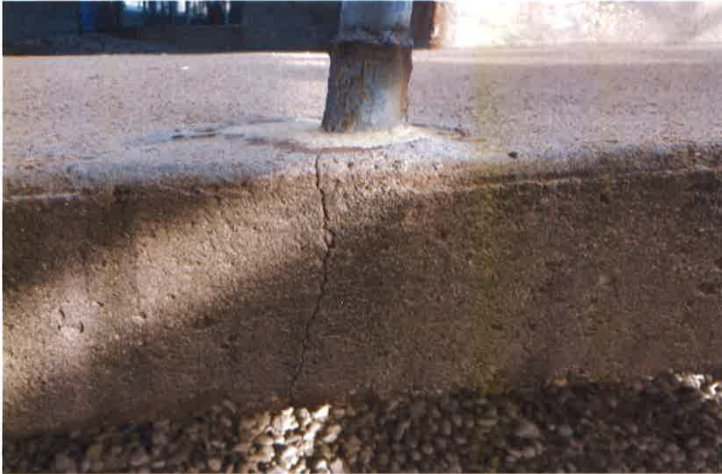
Photo 58: Radiating Crack form Repaired Handrail Post
