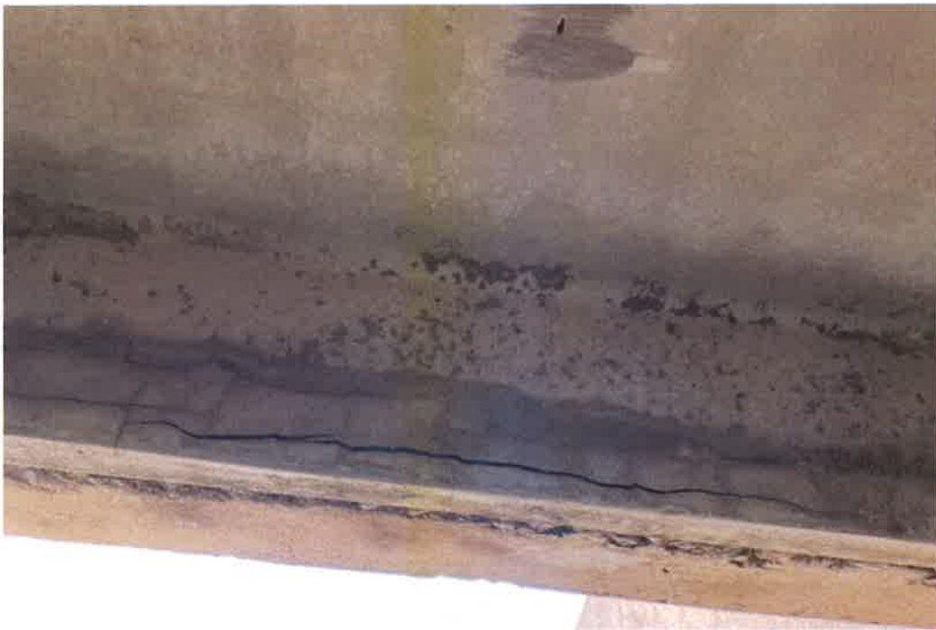
Photo 33: Exposed Rusted Rebar After Spalling of Repair on Ramp Sidewall
