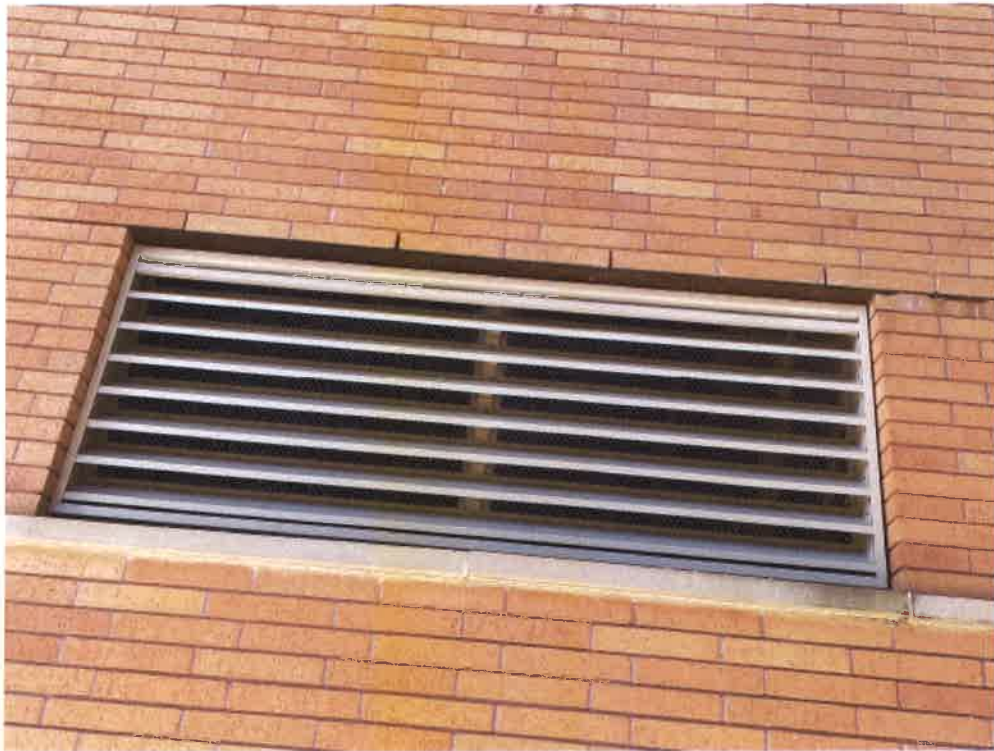
Photo 74: Rusted Lintel for Wall Opening
