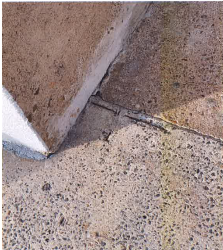
Photo 35: Exposed Welded Wire Mesh Where Ramp Meets Landing
