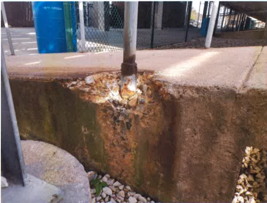
Photo 55: Rusted Handrail with Concrete Damage
