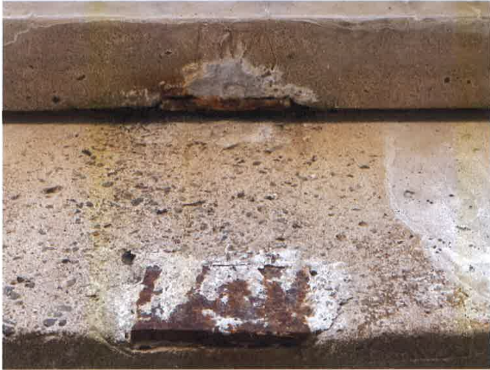
Photo 30: Rusted Diaphragm Tie Plate
