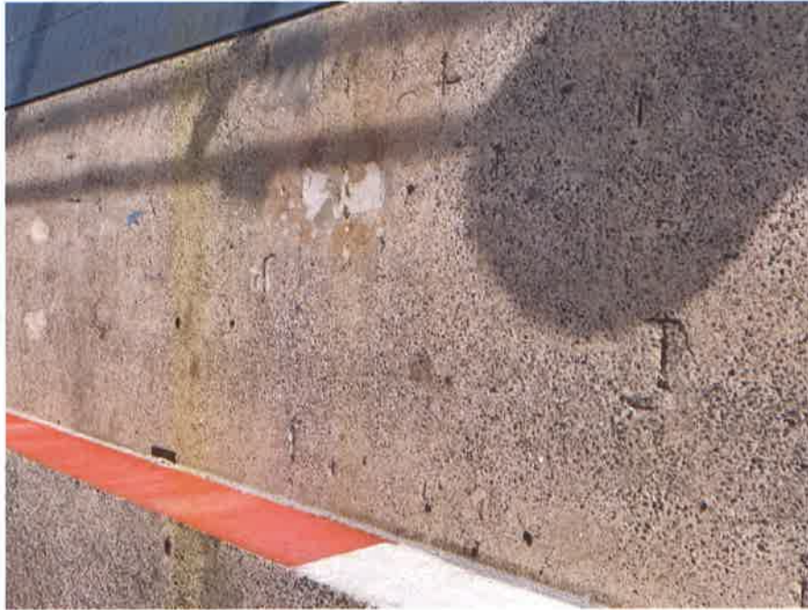
Photo 36: Deteriorated Top Slab
