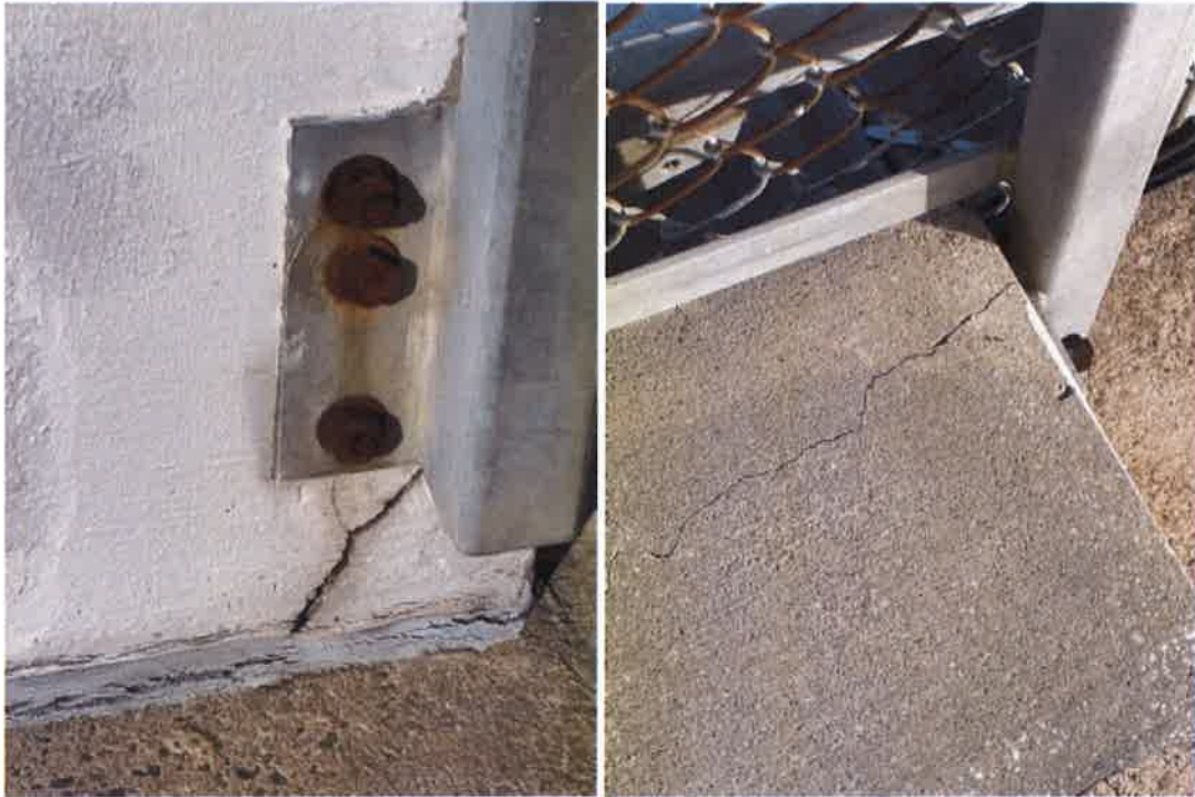
Photo 39: Rusted Anchor of Handrail with Crack in Concrete
