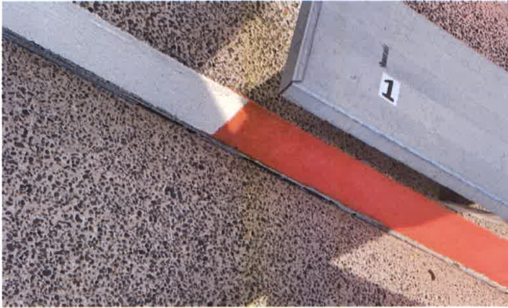
Photo 38: Deterioration of Sealant
