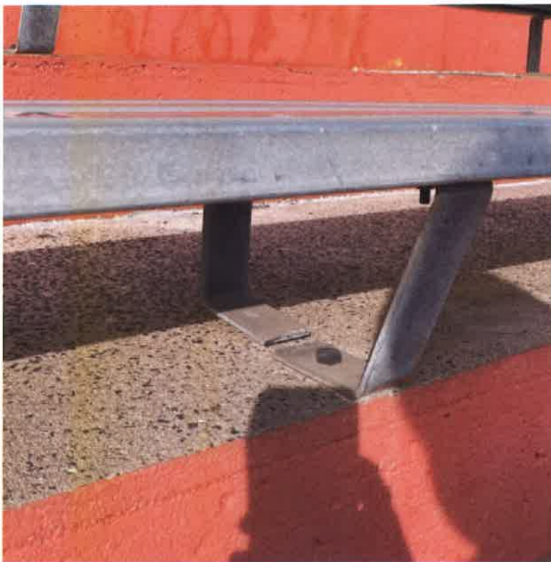
Photo 49: Broken Seating Arrangement
