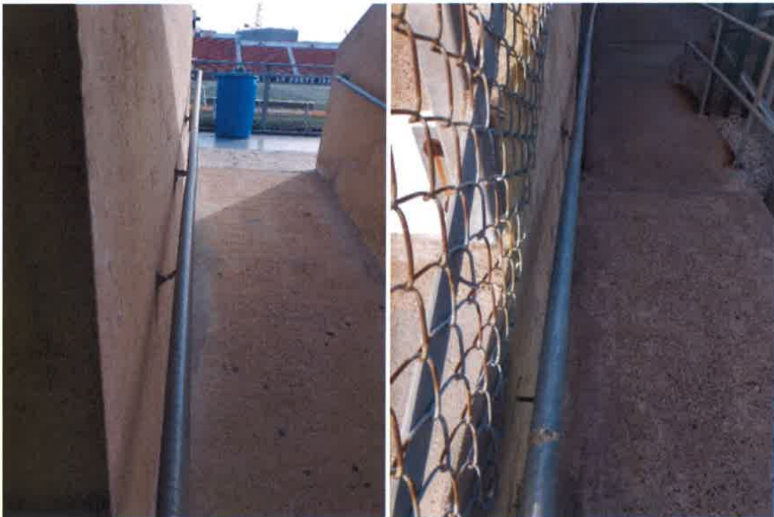
Photo 59: Broken Handrail Embed to Sidewall
