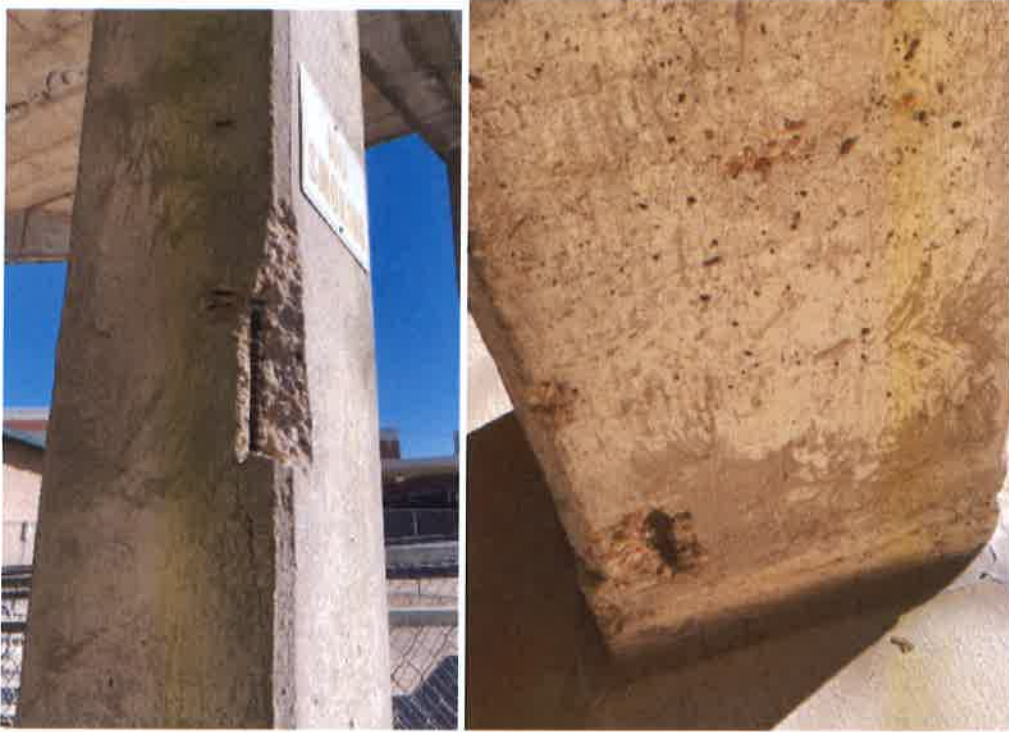
Photo 65: Exposed Rusted Rebar After Spalling of Concrete
