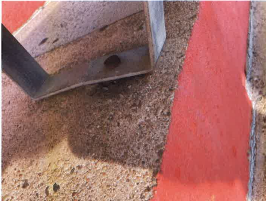
Photo 48: Rusted Anchor Bolts Sitting on Pothole with Dirt
