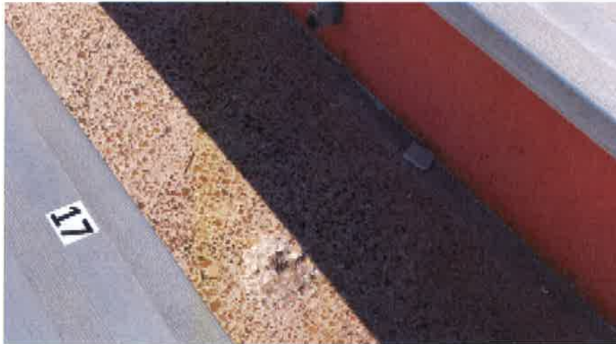
Photo 90: Potholes on Top of Secondary Beams
