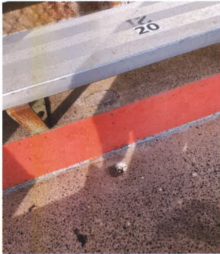
Photo 37: Delamination at Pot Holes
