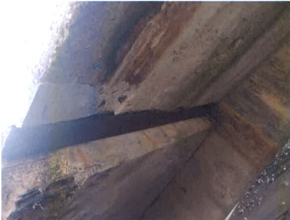
Photo 54: Rusted Lintel with Exposed Rebar After Spalling of Concrete
