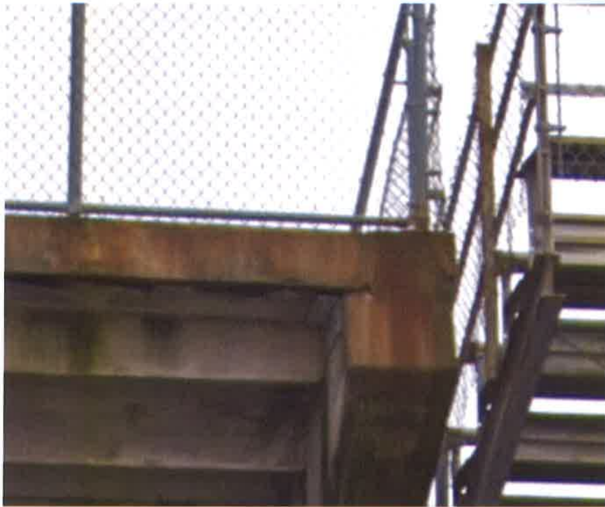
Photo 60: Fence Post Deforming the Concrete Corner
