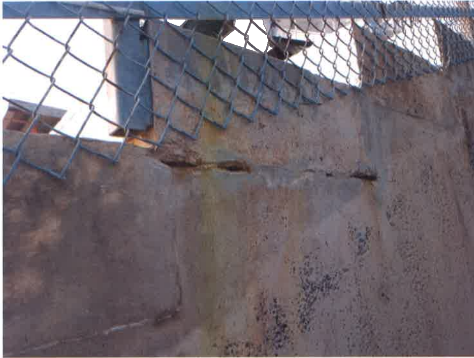
Photo 56: Exposed Rusted Rebar on Top of Raker beam
