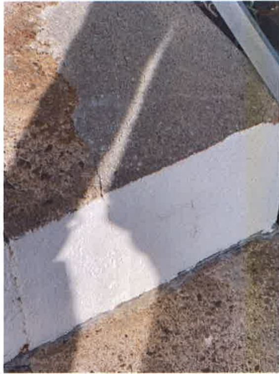
Photo 40: Crack at Repaired Patch of Concrete
