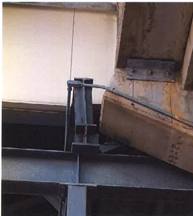
Photo 61: Non-Plumb Steel Beam Supporting Press-box
