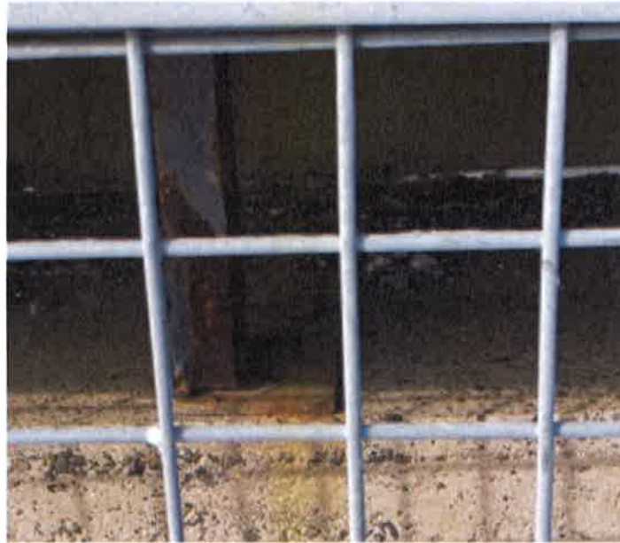
Photo 44: Rusted Support to Press-Box without Anchor bolt
