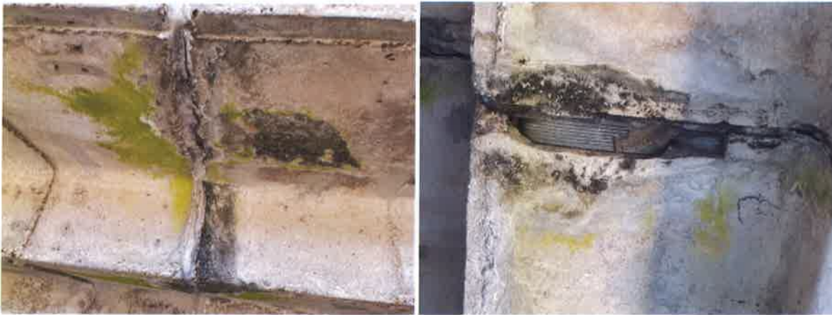
Photo 70: Water Seepage from Deteriorated Cold Joint Sealant
