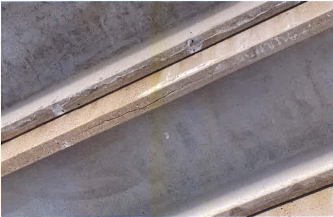
Photo 27: Crack on Joist Web
