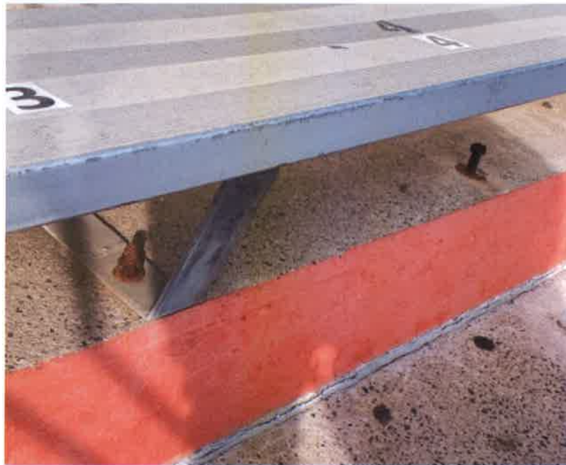
Photo 51: Rusted Anchor Protruding (Source of Hazard)
