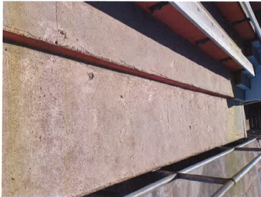
Photo 88: Delamination of Slab with Uniform Cracks for Entire Span
