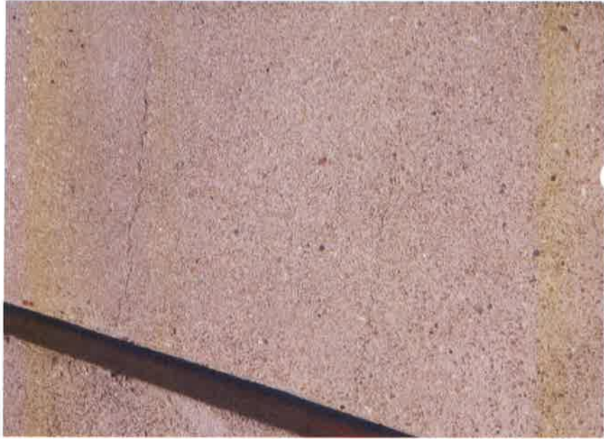
Photo 83: Typical Crack on Slab on Either side of Raker Beam Underneath
