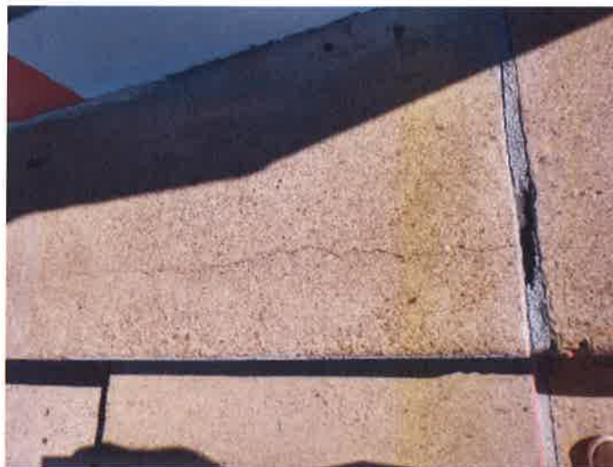
Photo 82: Worn Sealant with Horizontal Crack on Slab
