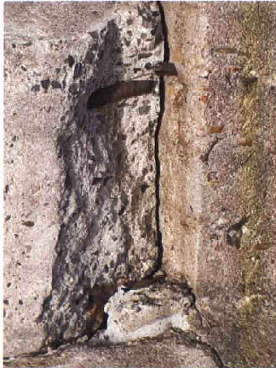
Photo 41: Spalling of Concrete with Exposed Broken rebar on Step "U"
