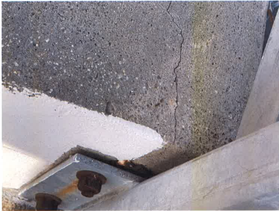
Photo 52: Handrail Support With Rusted Anchor Radiating Crack Across the Topping slab
