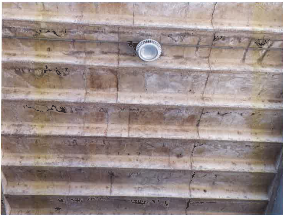
Photo 72: Horizontal Cracks in Secondary Beams Leading to Seepage
