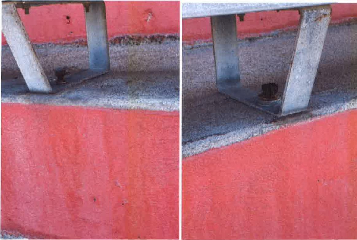
Photo 89: Improper Arrangement of Rusted Anchor Bolts
