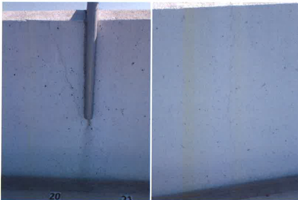
Photo 76: Hairline Cracks on Sidewalls
