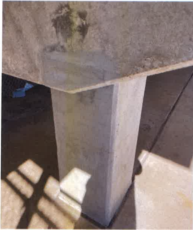
Photo 67: Crack Radiating from Repaired Beam
