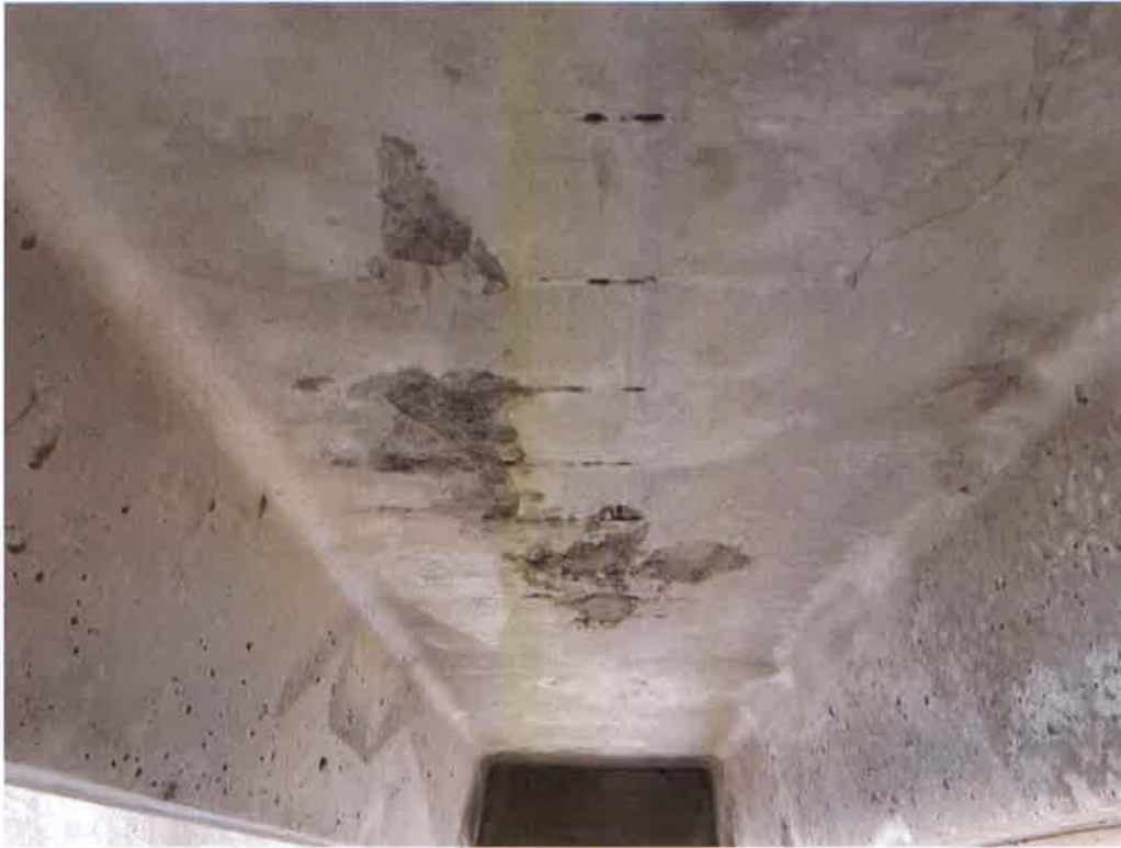
Photo 26: Spalling of Concrete Under Slab
