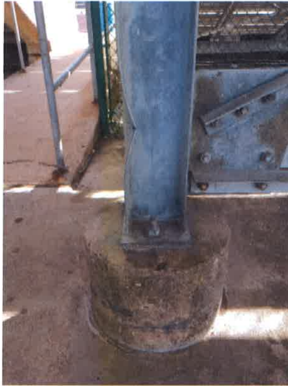
Photo 62: Steel Bleacher Column Deformation
