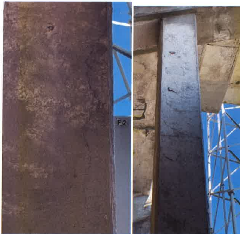
Photo 66: Crack and Delamination in Concrete Column
