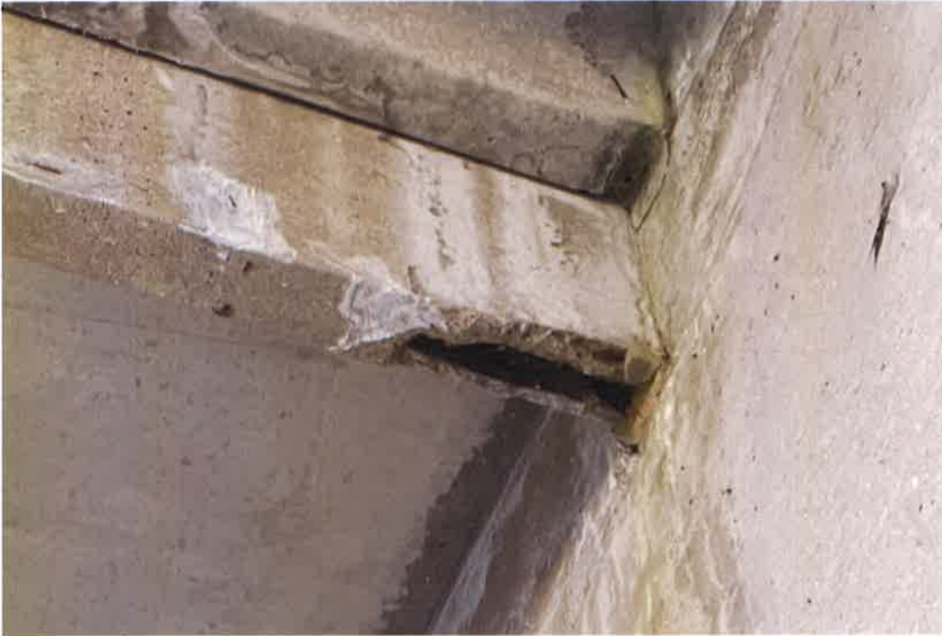
Photo 28: Spalling/Exposed Rebar at Joist Web
