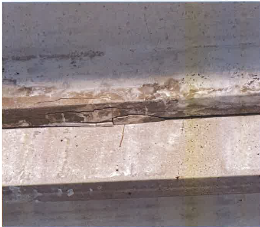
Photo 29: Significant Joist Cracking
