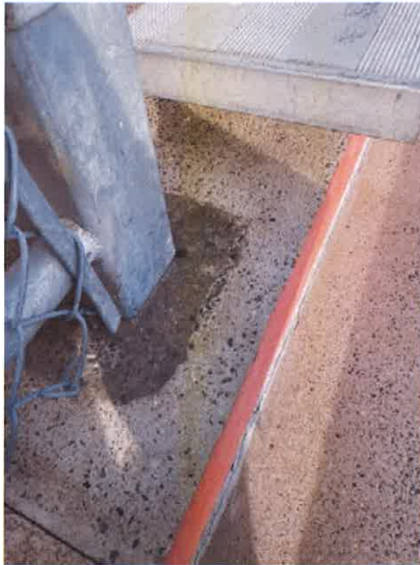
Photo 45: Concrete Crack and Delamination at Posts
