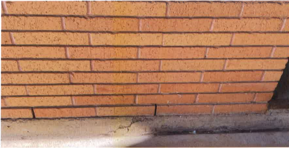
Photo 73: Crack in Brick Ledge of Wall
