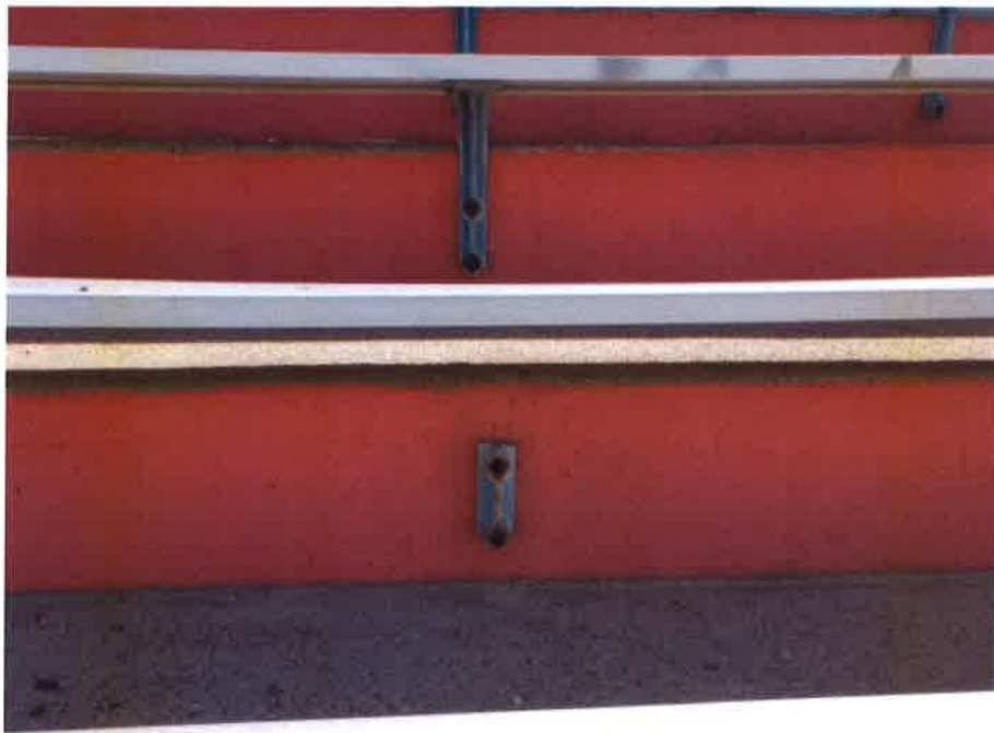
Photo 78: Broken Seating Support
