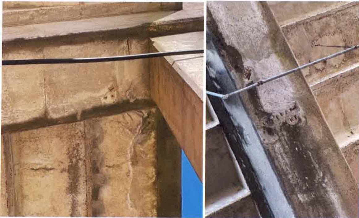
Photo 68: Concrete Spalling with Exposed Rebar in Primary Beams
