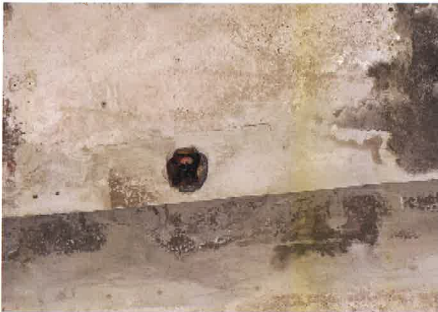
Photo 64: Rusted Duct Inside Stadium Riser
