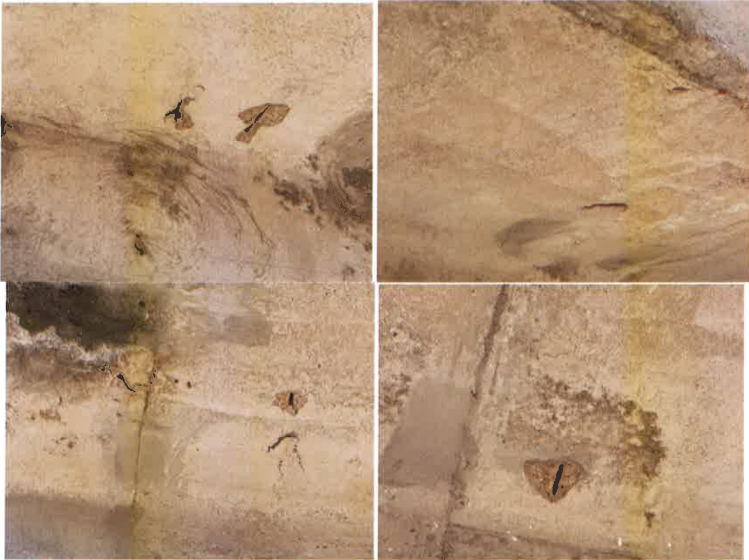
Photo 71: Spot Spalling and Delamination of Secondary Beams
