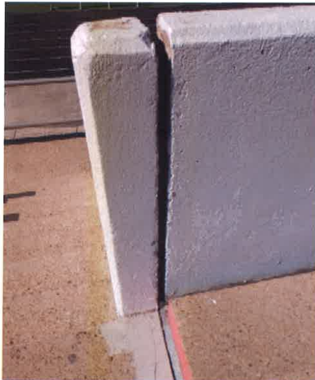
Photo 80: Wide Sidewall Cold Joint (source of Hazard)
