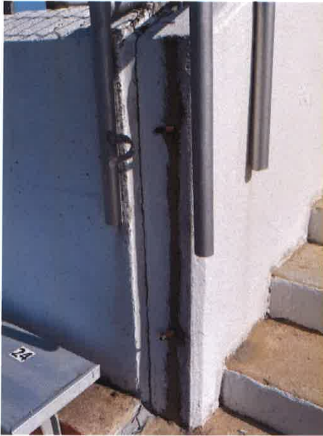
Photo 87: Protruding Rusted Anchor Bolt (Source of Hazard)
