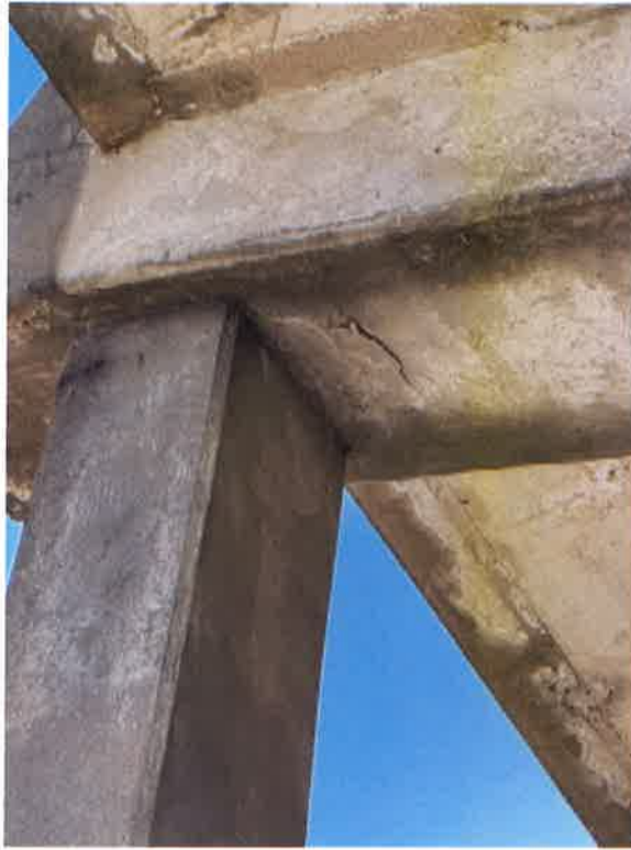
Photo 69: Concrete Delamination in Primary Beams
