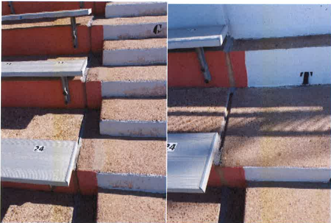
Photo 84: Worn Sealant At All Cold Joint
