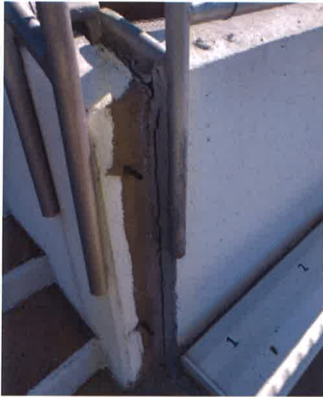
Photo 79: Anchor Rods Protruding from Sidewall (Source of Hazard)
