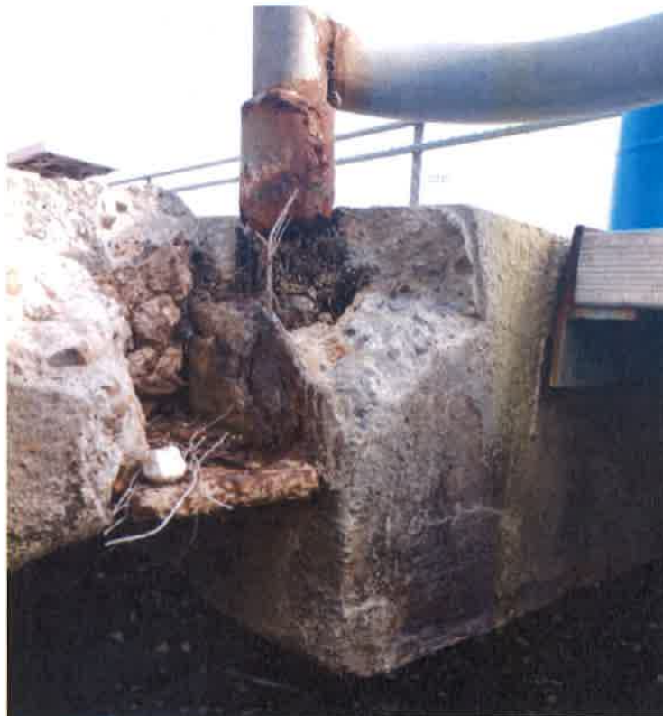
Photo 53: Deteriorated Handrail Support on Top of Rusted Lintel with Spalling of Concrete
