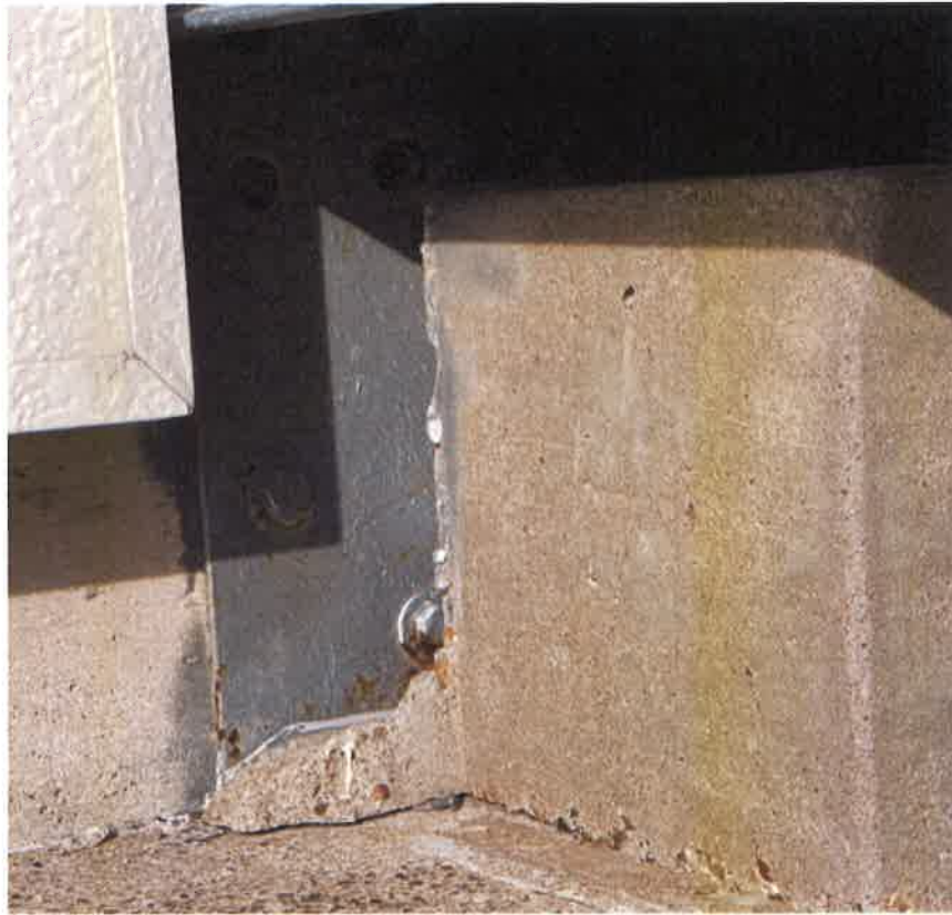
Photo 46: Bearing Plate Missing Anchor bolts
