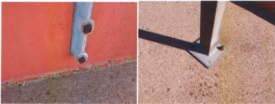
Photo 77: Rusted Anchor for Seating Arrangement
