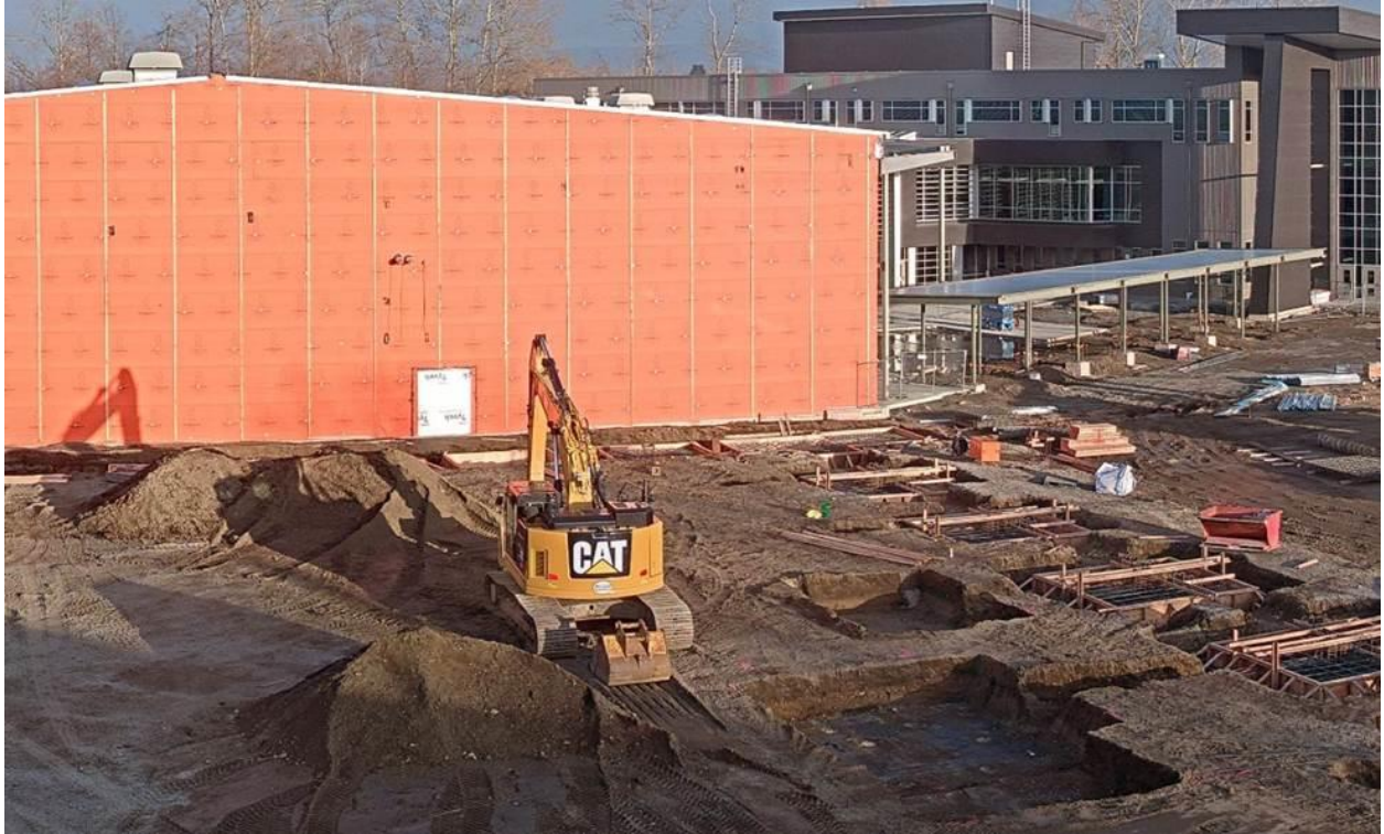
Excavating for and forming of the foundation under the new CTE Wing
