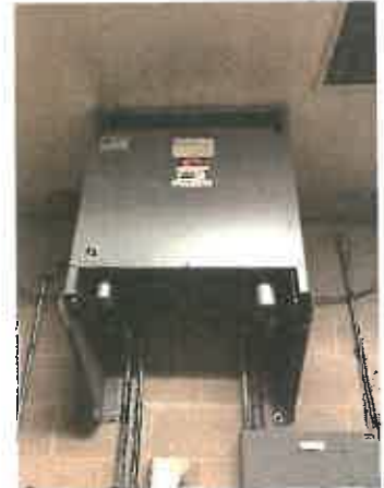
Biglerville ES Transformer
