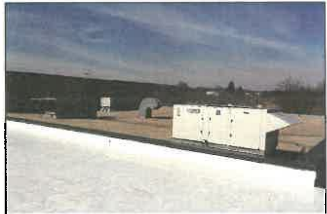
Biglerville HS/MS Rooftop Units
