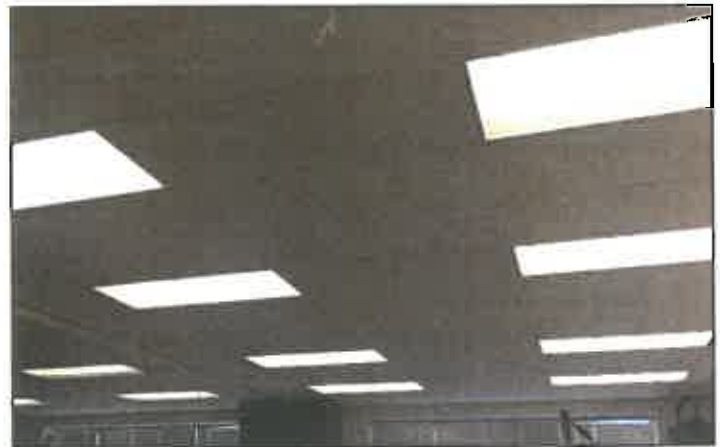
Existing Fluorescent Lighting
