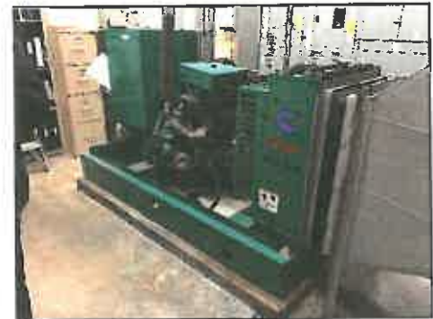
Biglerville HS/MS Generator
