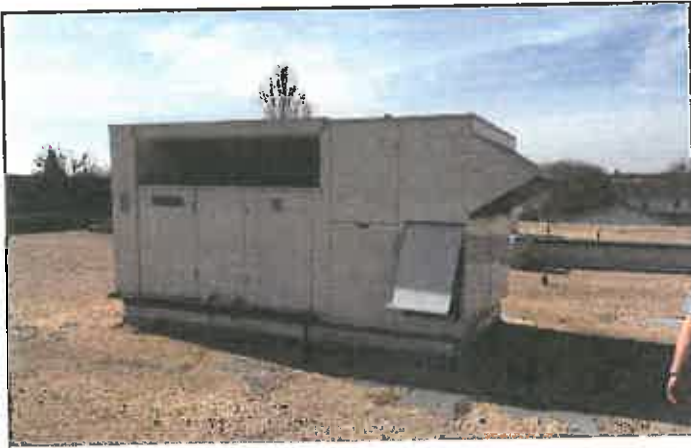
Biglerville HS/MS Rooftop Unit
