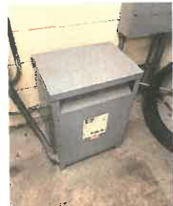
Biglerville HS/MS Transformer
