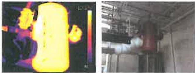
Arendtsville Elementary School Air/Dirt Separator
