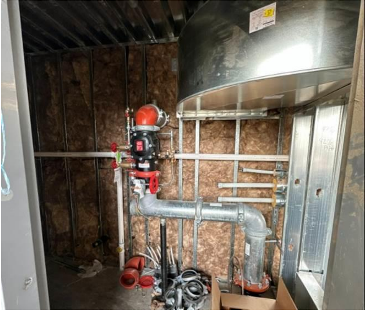
Fire sprinkler piping in the Grandstands' restrooms/concessions area
