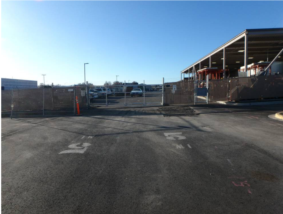
Tri Tech gate (working on the control wiring) waterline trench – west end
