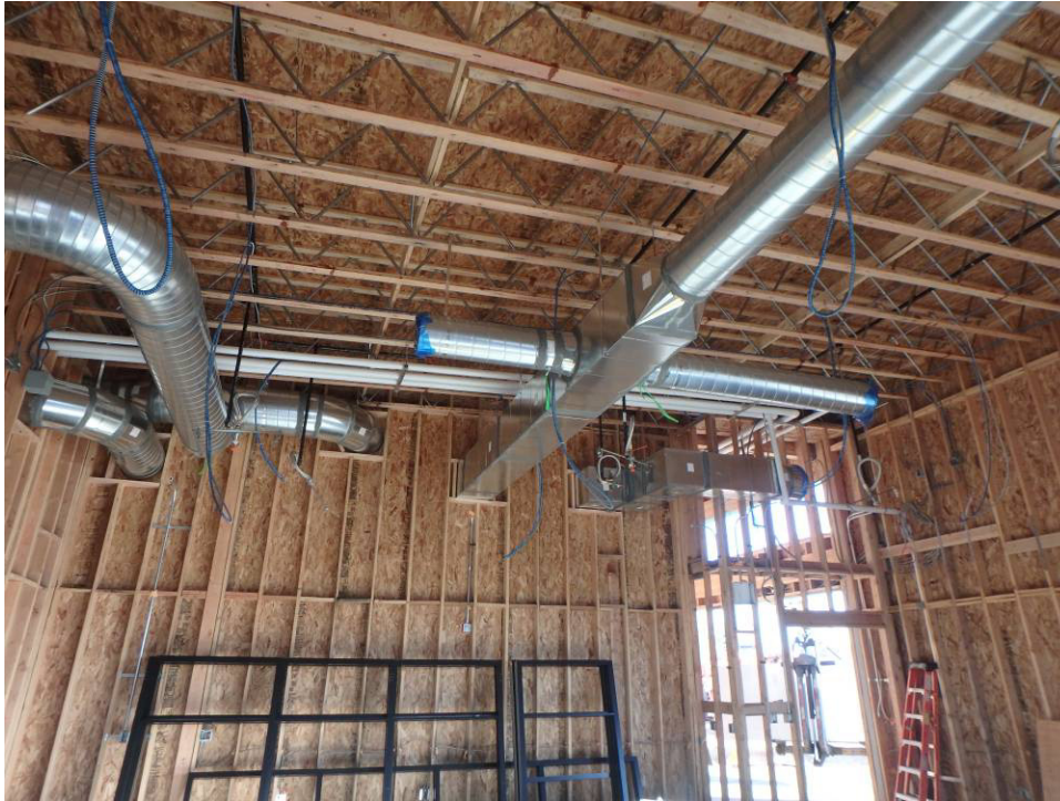
Framing and ductwork above the north wall and entry of the south classroom
