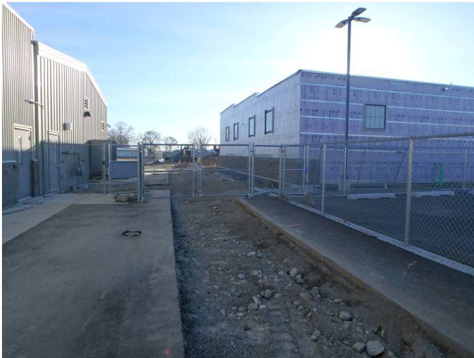
Looking east at the west end of the water line tie-in trench
