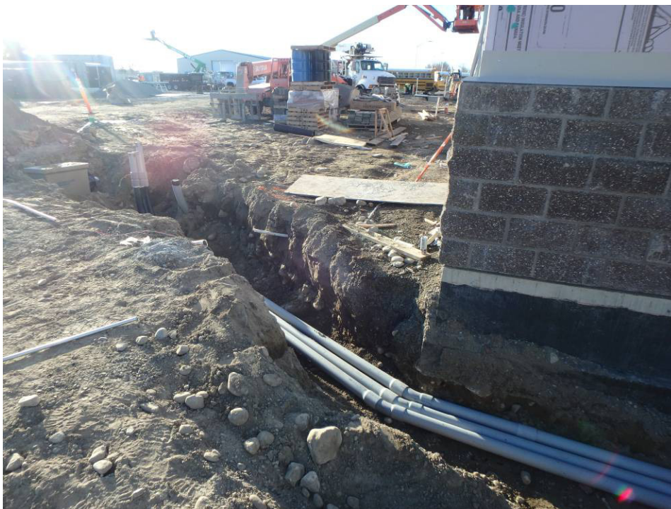
Northeast fire hydrant, and electrical conduits in the NE building island
