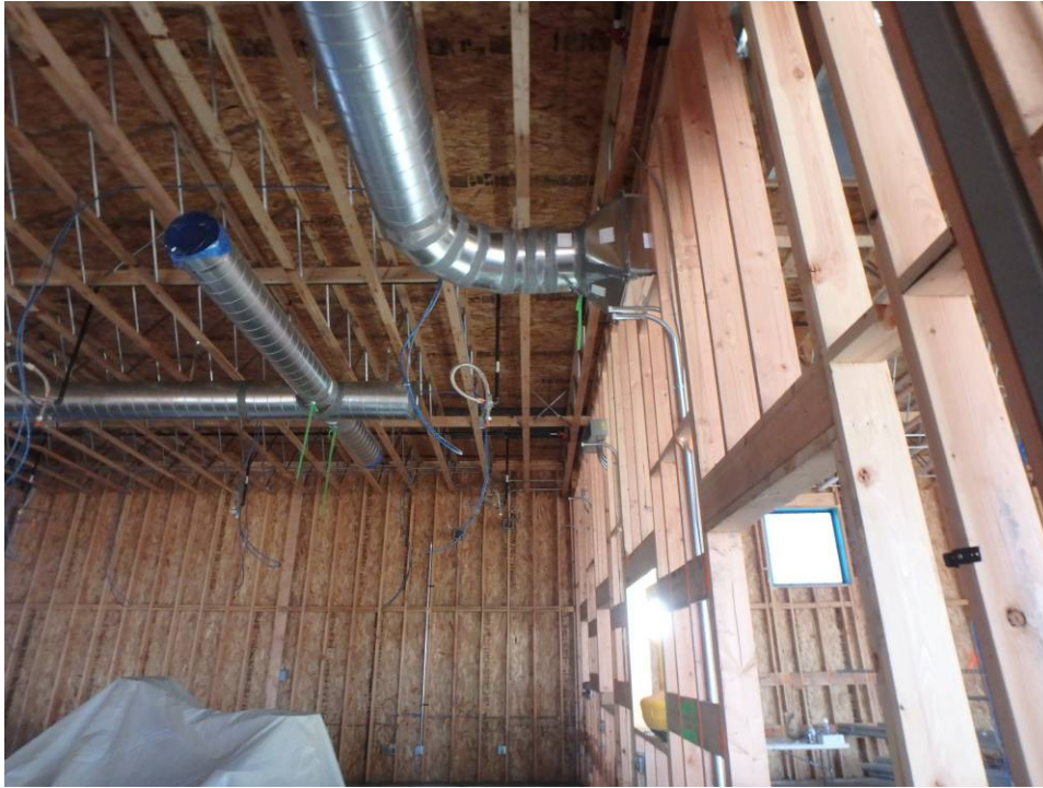
Looking west at the ductwork in the North Classroom
