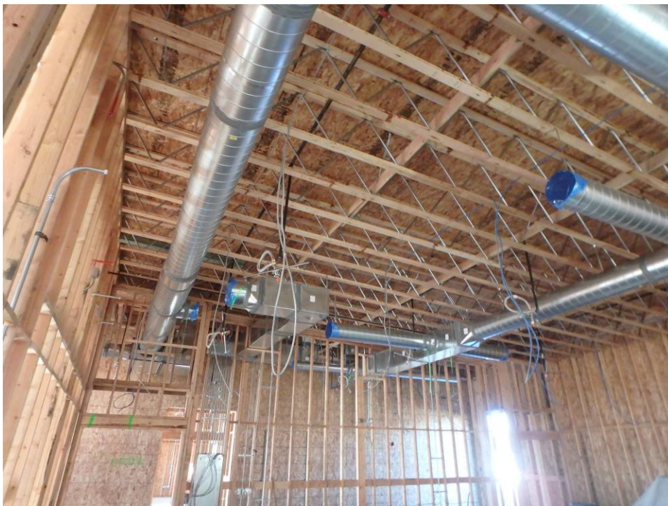
Looking south at the ductwork in the North Classroom
