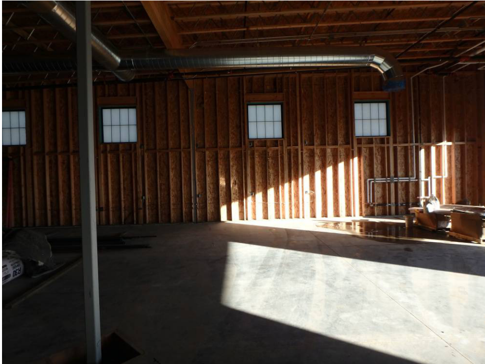
Ductwork above the north wall of the shop
