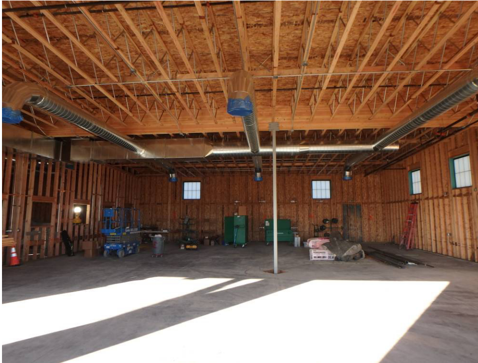
Looking west at the west wall of the shop and the ductwork
