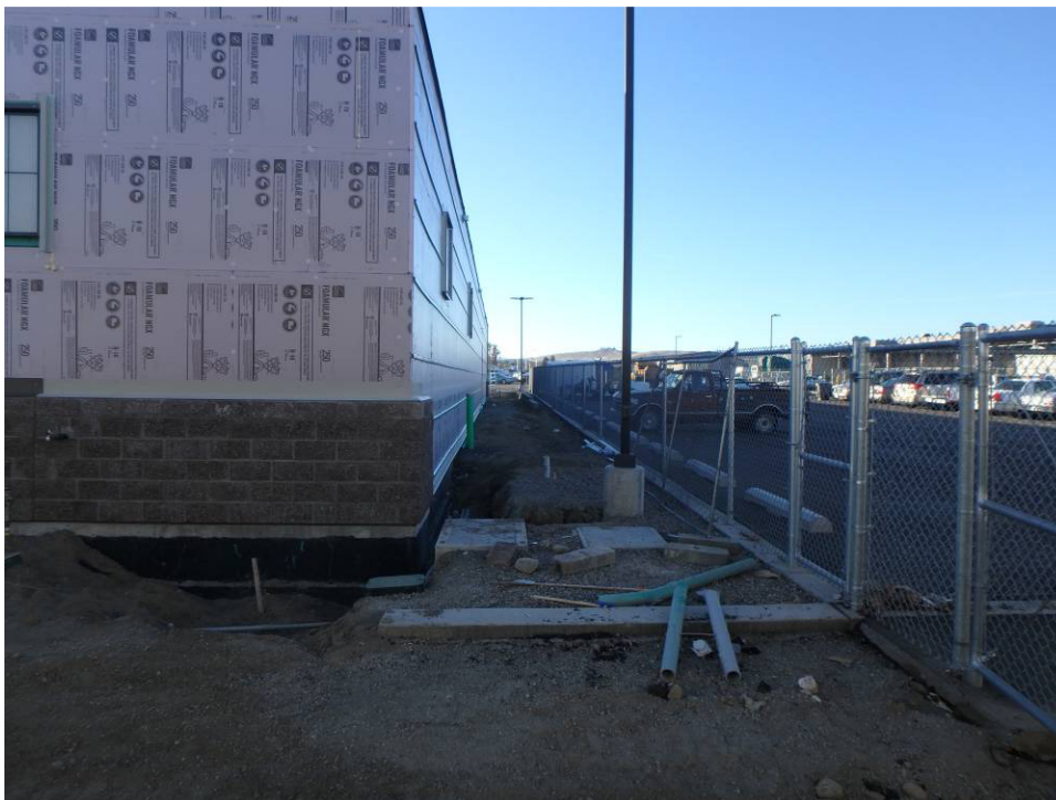
Looking south at the northwest corner of the building and CMU wainscot and the west property line
