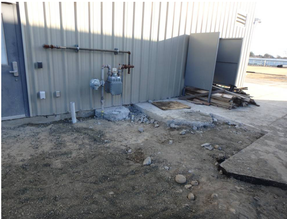
Tri Tech east gas meter
