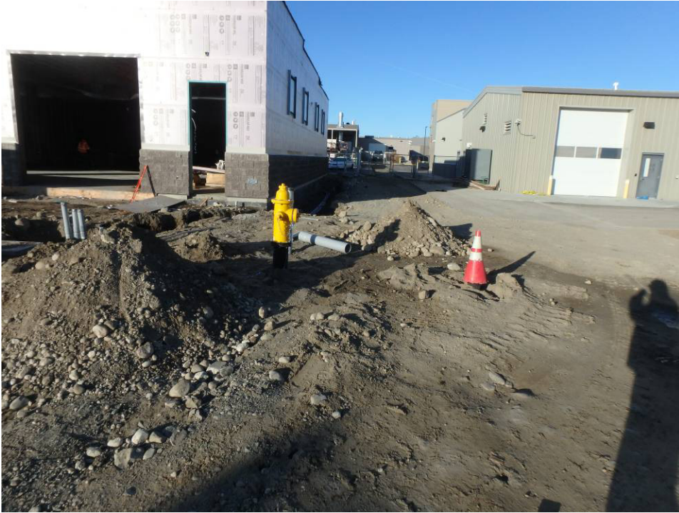
Looking west at the northeast corner of the building and NE island area and waterline backfill
