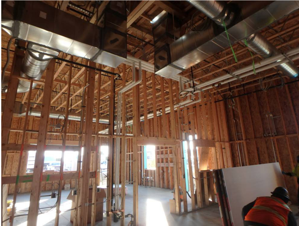
Ductwork over the south classroom
