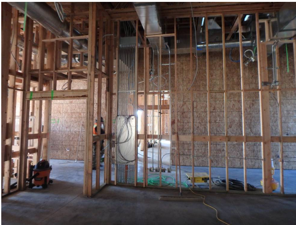
Area above the electrical panel
