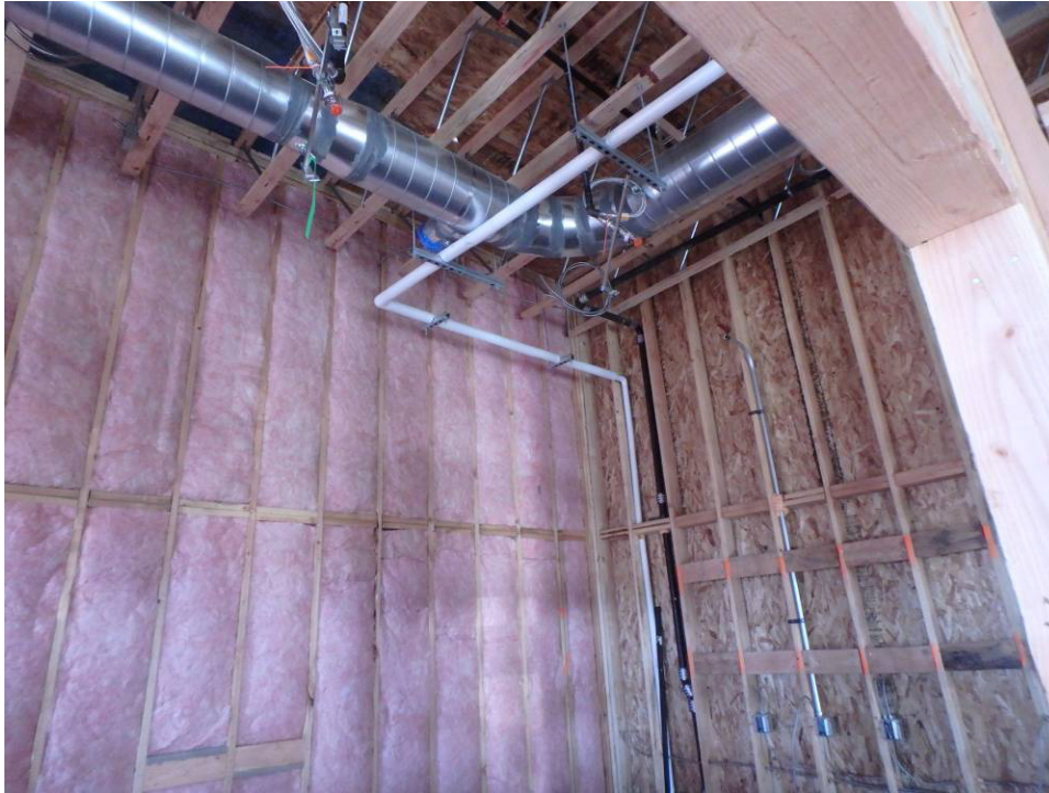
Wall insulation in the south end of the west wall and behind the dryer vent
