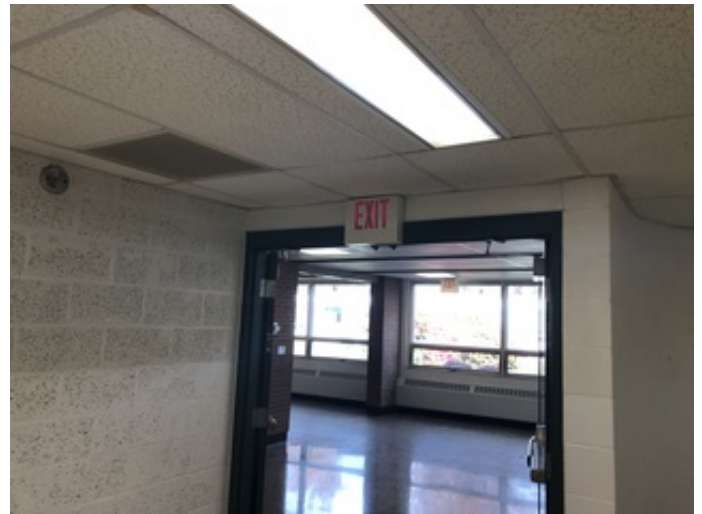
Typical exit fixture
