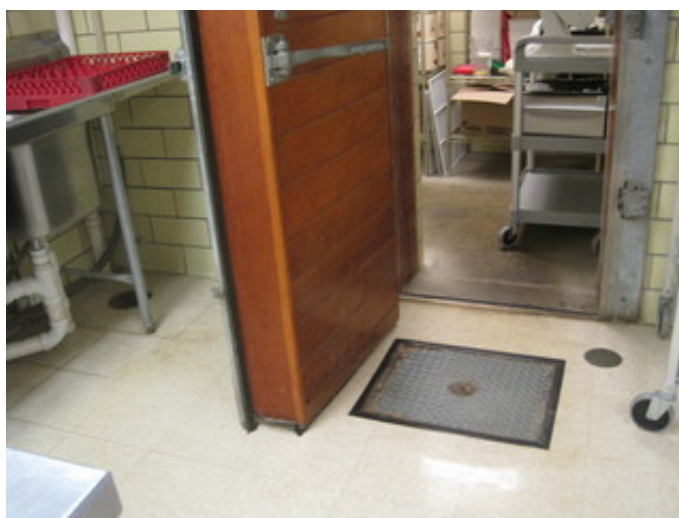
Grease Waste Interceptor Below Dishwasher
