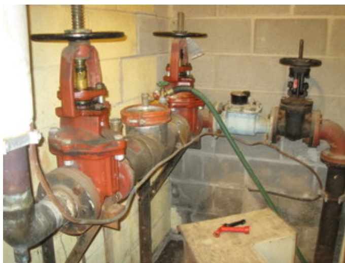
Heating water pumps
