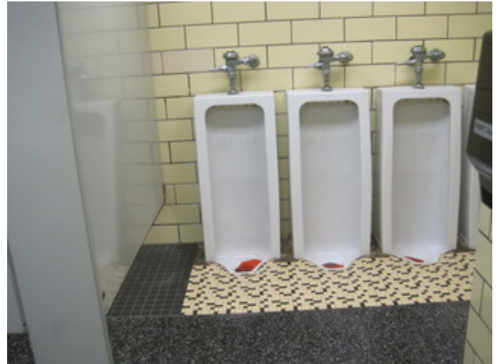
Floor-mounted urinals w/manual flush vales
