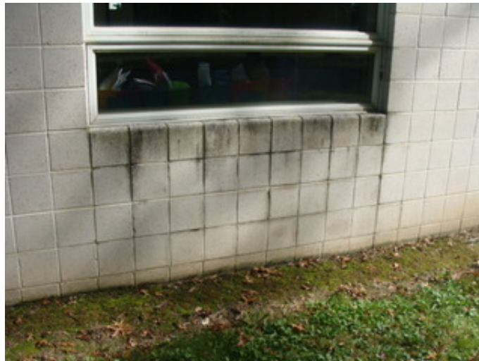
Exterior CMU That Needs To Be Cleaned
