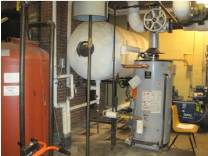
Domestic Water Heater & Storage Tank
