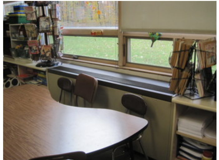
Classroom Univ Ventilator
