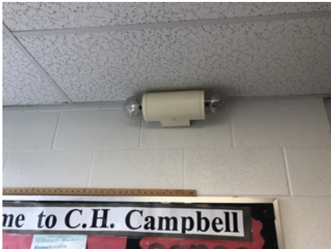
Typical emergency fixture
