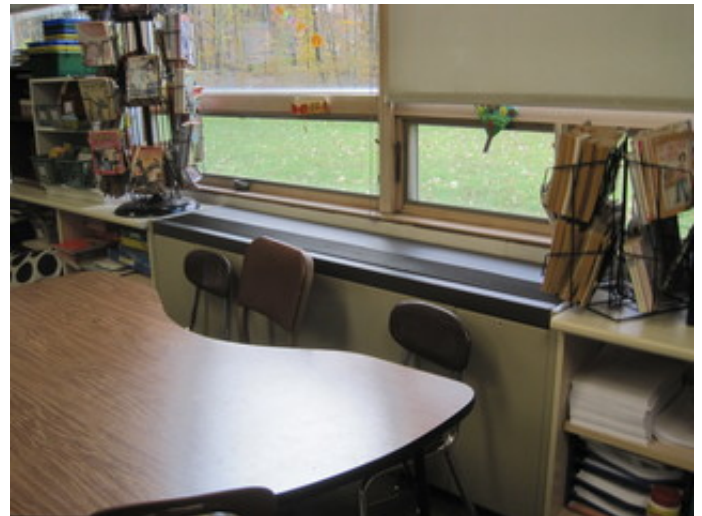
Classroom Univ Ventilator
