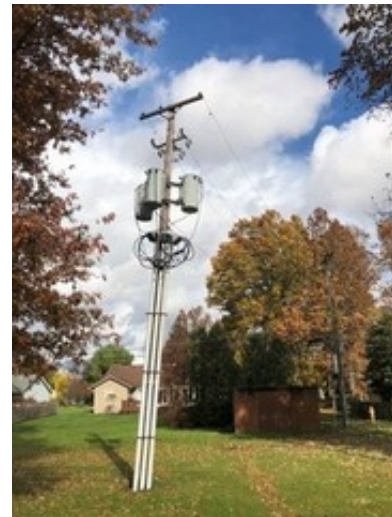
Pole mounted transformer
