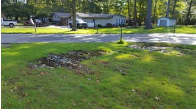
Ponding near Pavement Approach
