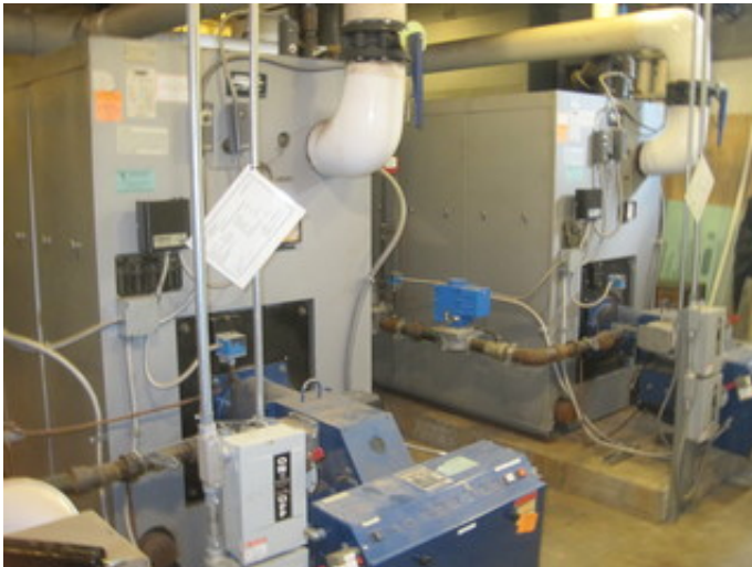
Heating water boilers
