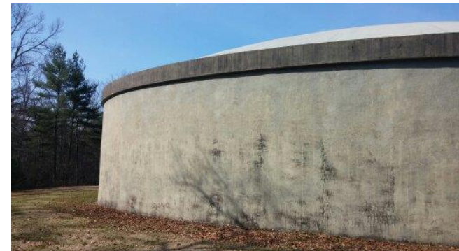
The 4.0 Million Gallon Drury Lane Tank
