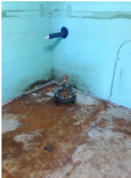
Figure 4-13. Gilbert Road Station – HWW Raw Water Pipe Termination
