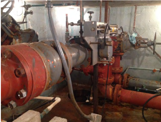
Figure 4-7. Pumping Station Lower Level
