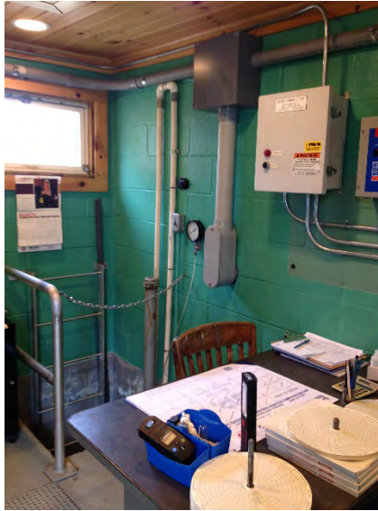
Figure 4-6. Pumping Station Upper Level
