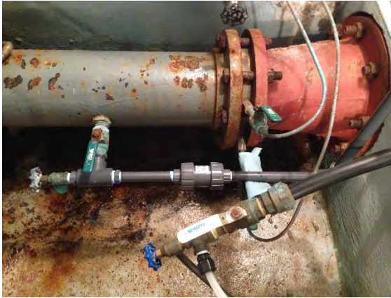
Figure 4-8. Chemical Feed and Flow Meter
