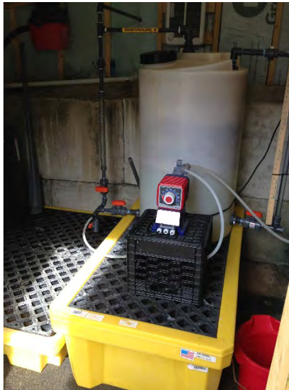
Figure 4-9. Sodium Hypochlorite Feed System
